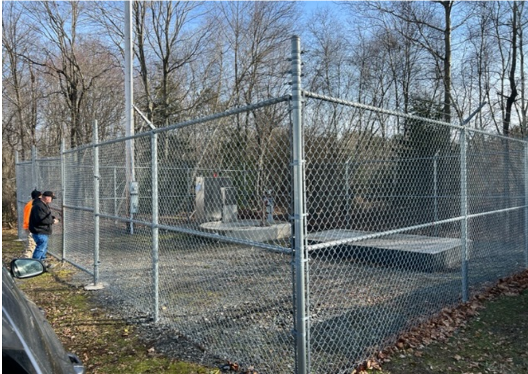
Highland pump station
