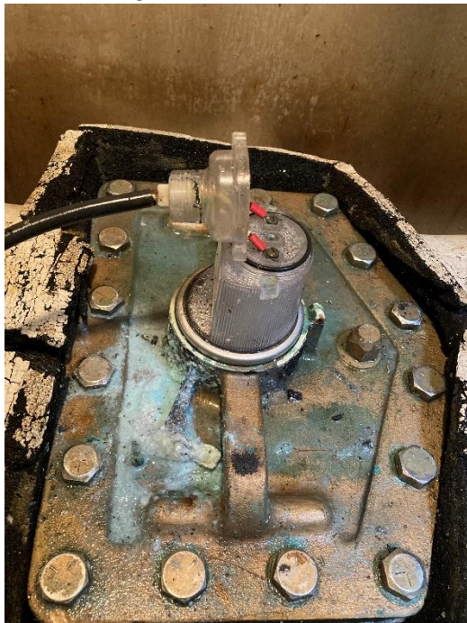
Figure 3 – Vault 1 Pressure Sensor
