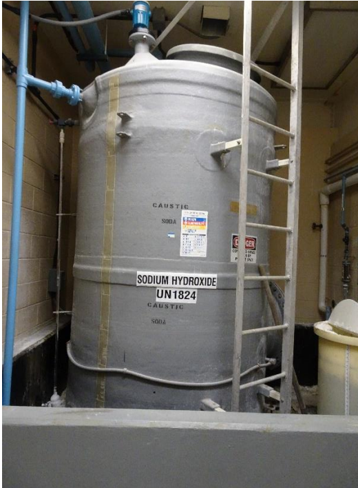
Figure 17 – Sodium Hydroxide Storage
