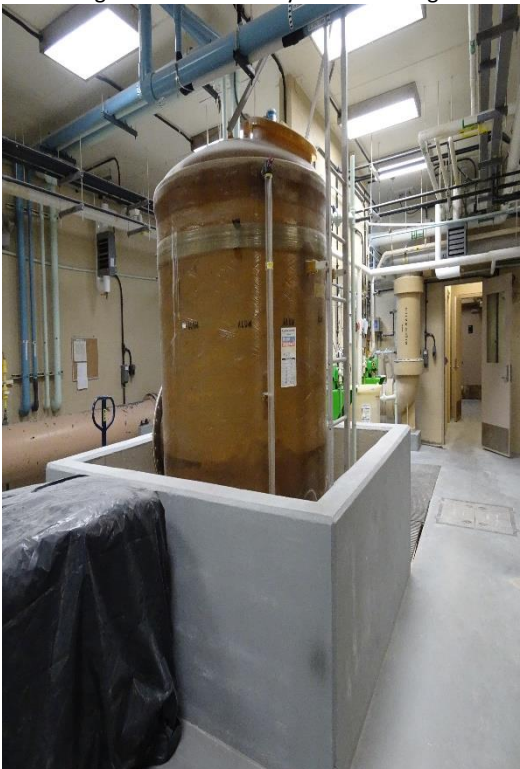
Figure 19 – Alum Storage Tank
