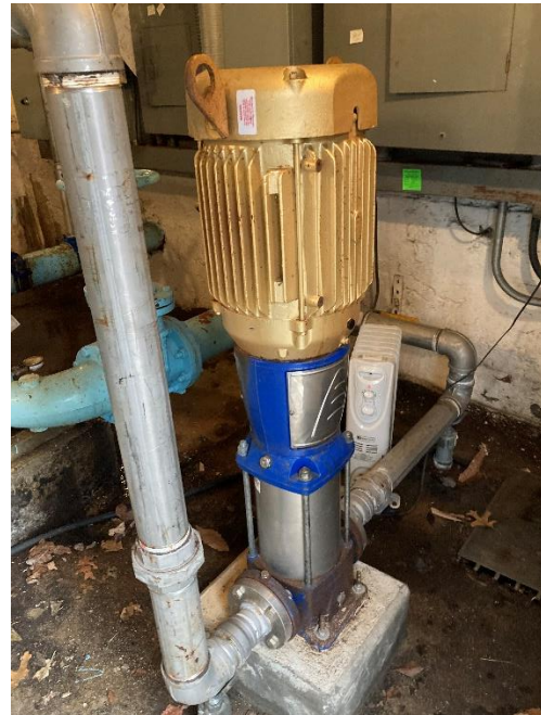
Figure 4 –Vertical Back-up Pumps
