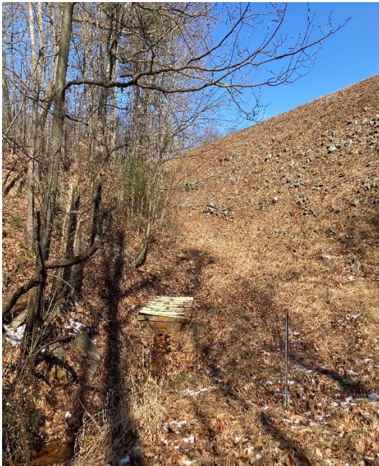
Figure 3 – Raven Run Dam No 2 – Right Embankment – Abutment and Drainage Weir at Toe of Dam
