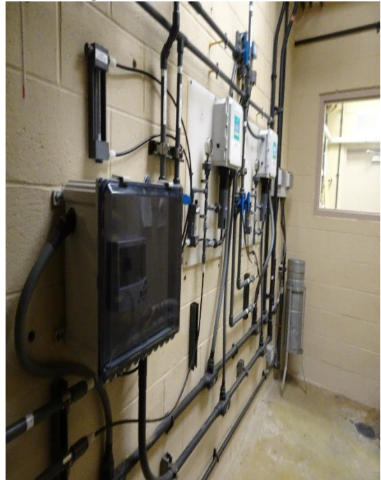
Figure 28 – Chlorine Dosing Room
