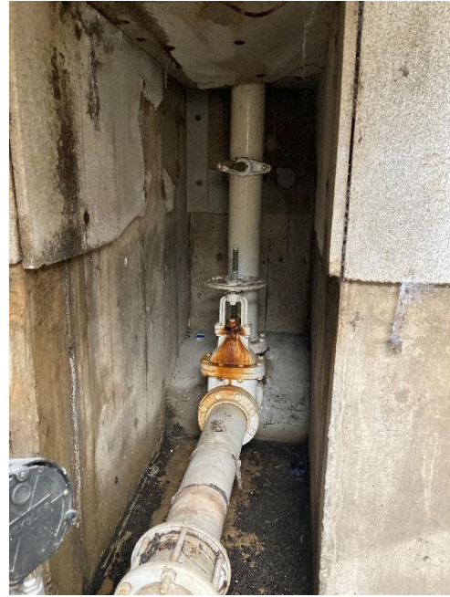
Figure 6 – Valve and Piping
