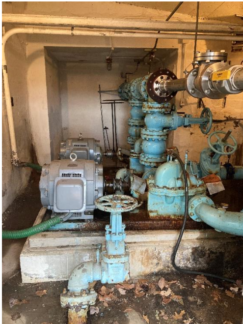
Figure 3 – Main Centrifugal Pumps
