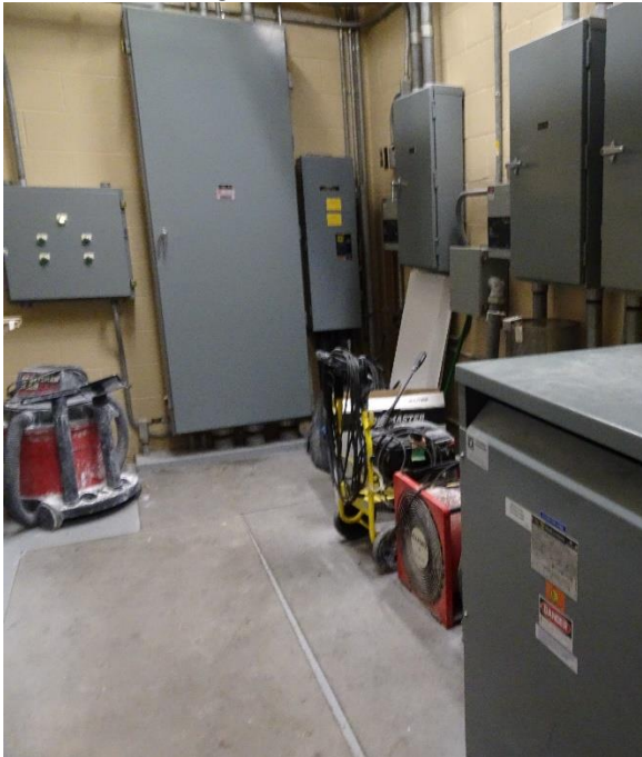
Figure 27 – Plant Electrical Room
