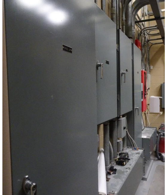
Figure 26 – Plant Electrical Room
