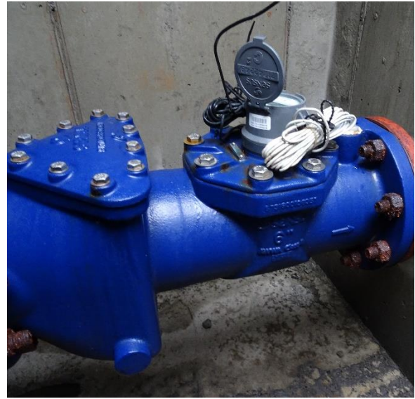
Figure 6 – Vault 2 Flow Meter
