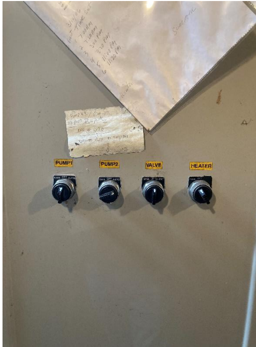
Figure 5 – Pump Control Panel
