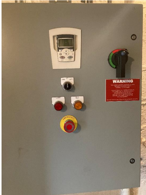
Figure 5 – Pump Control Panel
