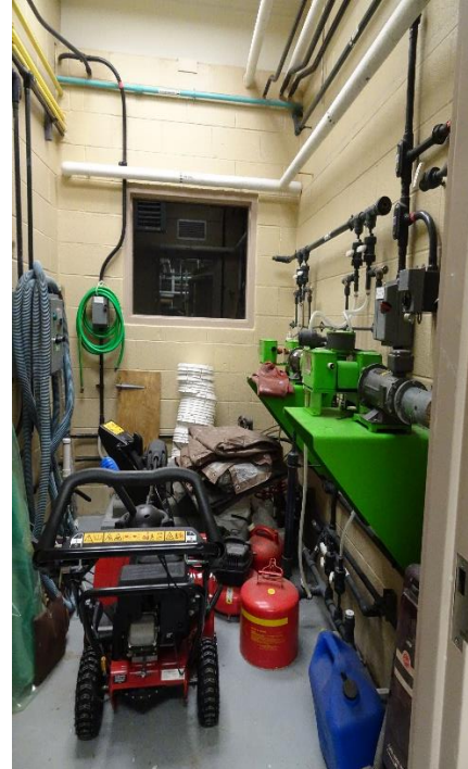
Figure 18 – Carbon Dosing Room
