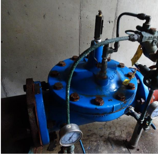
Figure 5 – Vault 2 Pressure Regulator
