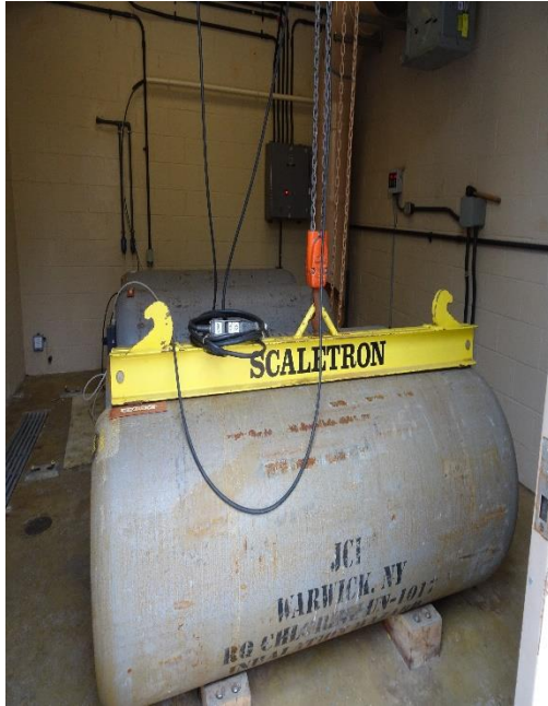
Figure 29 – Chlorine Storage Tanks
