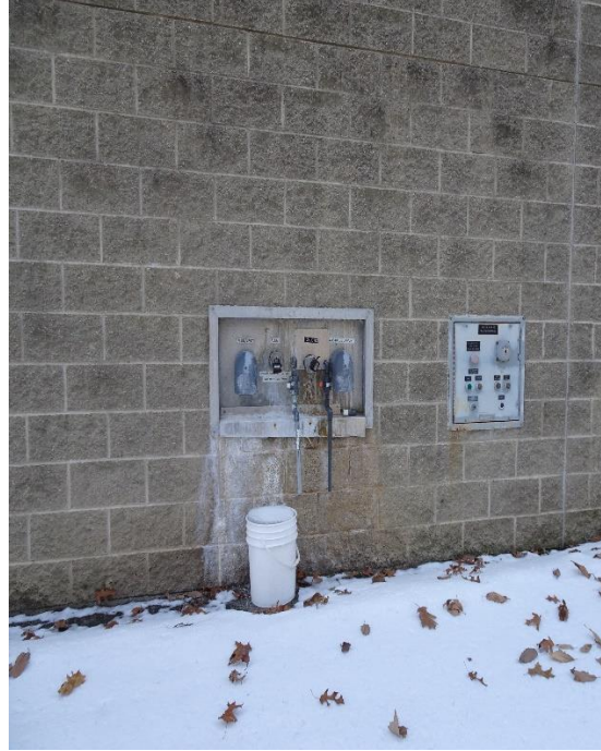
Figure 34 – Chemical Supply Delivery Connections
