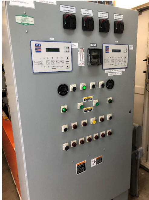
FIGURE 5.2-4: EASTVALE PUMP STATION PUMP CONTROLS
