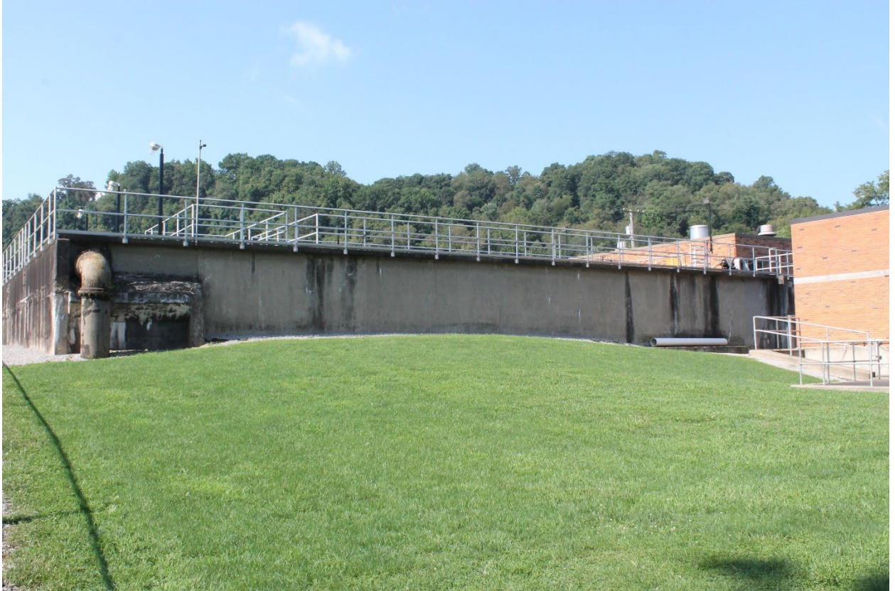
FIGURE 5.3 - 8: PRIMARY SETTLING TANKS-SIDE VIEW
