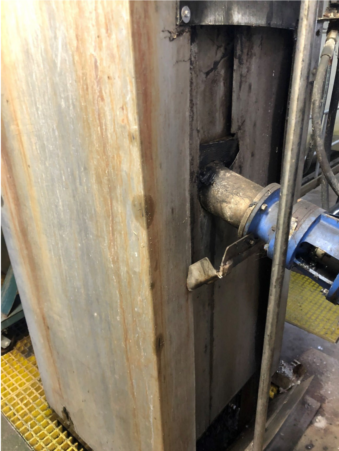
FIGURE 5.3 - 3: MECHANICAL BAR SCREEN
