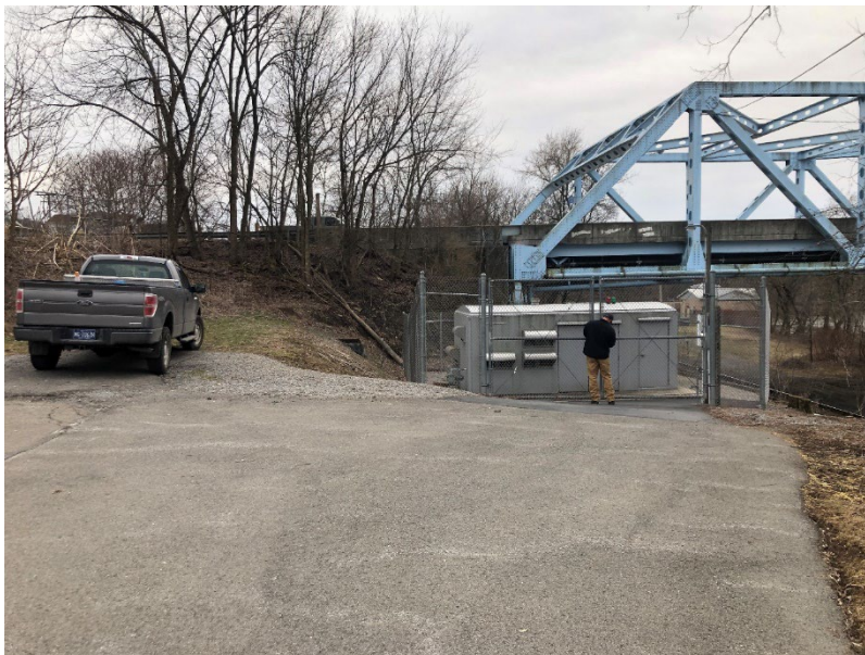
FIGURE 5.2-1: EASTVALE PUMP STATION VICINITY AND SECURITY FENCING
