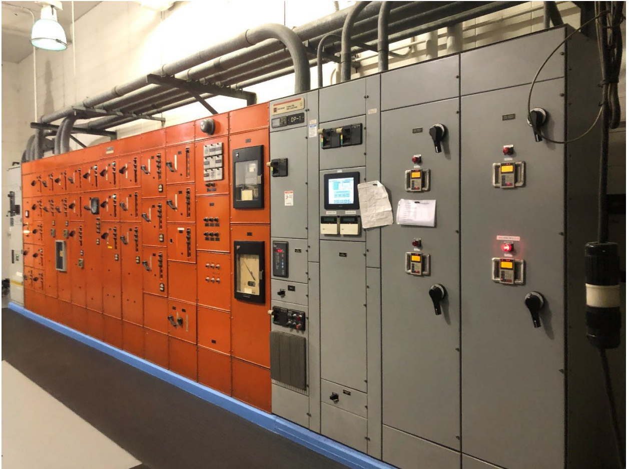
FIGURE 5.3 - 34: MOTOR CONTROL CENTERS
