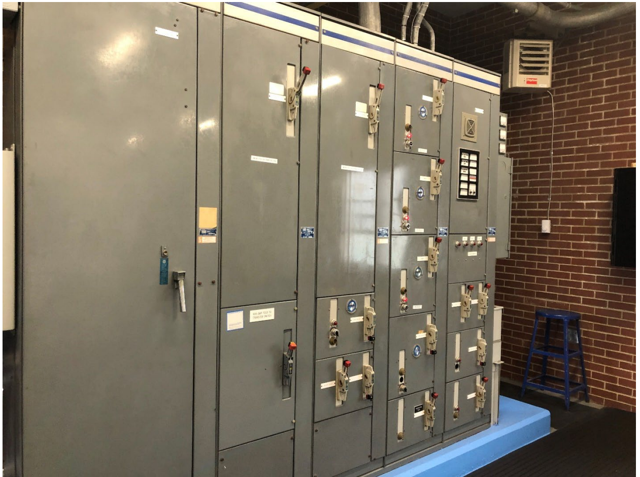
FIGURE 5.3 - 36: MOTOR CONTROL CENTER
