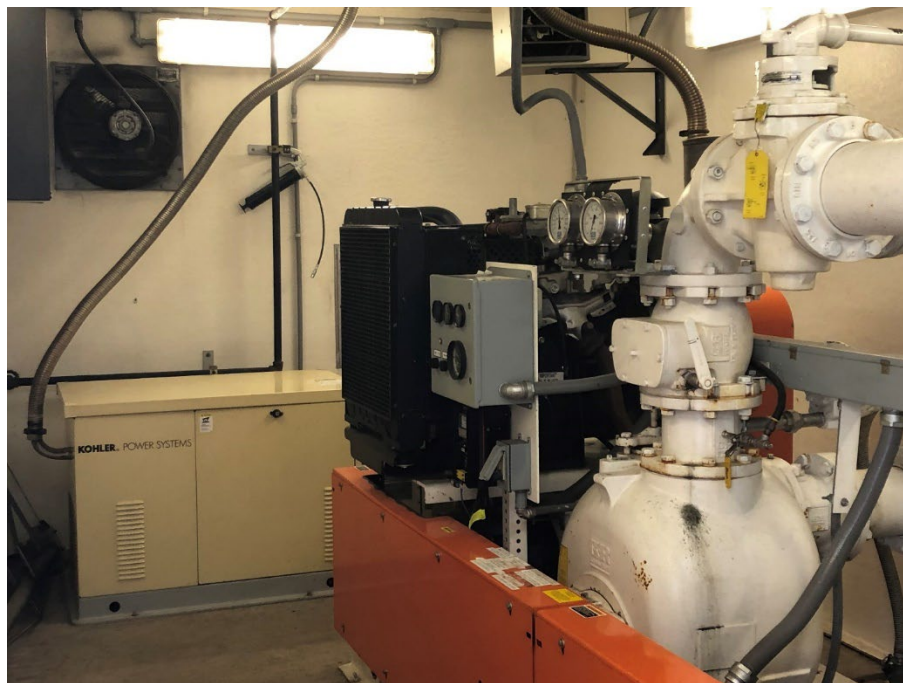
FIGURE 5.2-3: EASTVALE PUMP STATION SUCTION LIFT PUMPS
