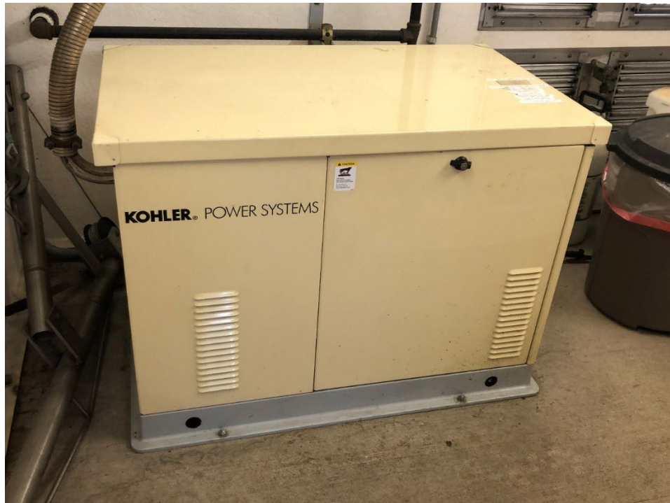
FIGURE 5.2-5: EASTVALE PUMP STATION NATURAL GAS POWERED EMERGENCY GENERATOR
