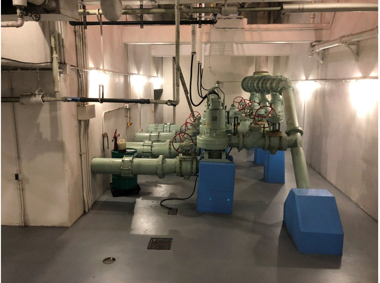
FIGURE 5.3 - 4: RAW SEWAGE PUMPS
