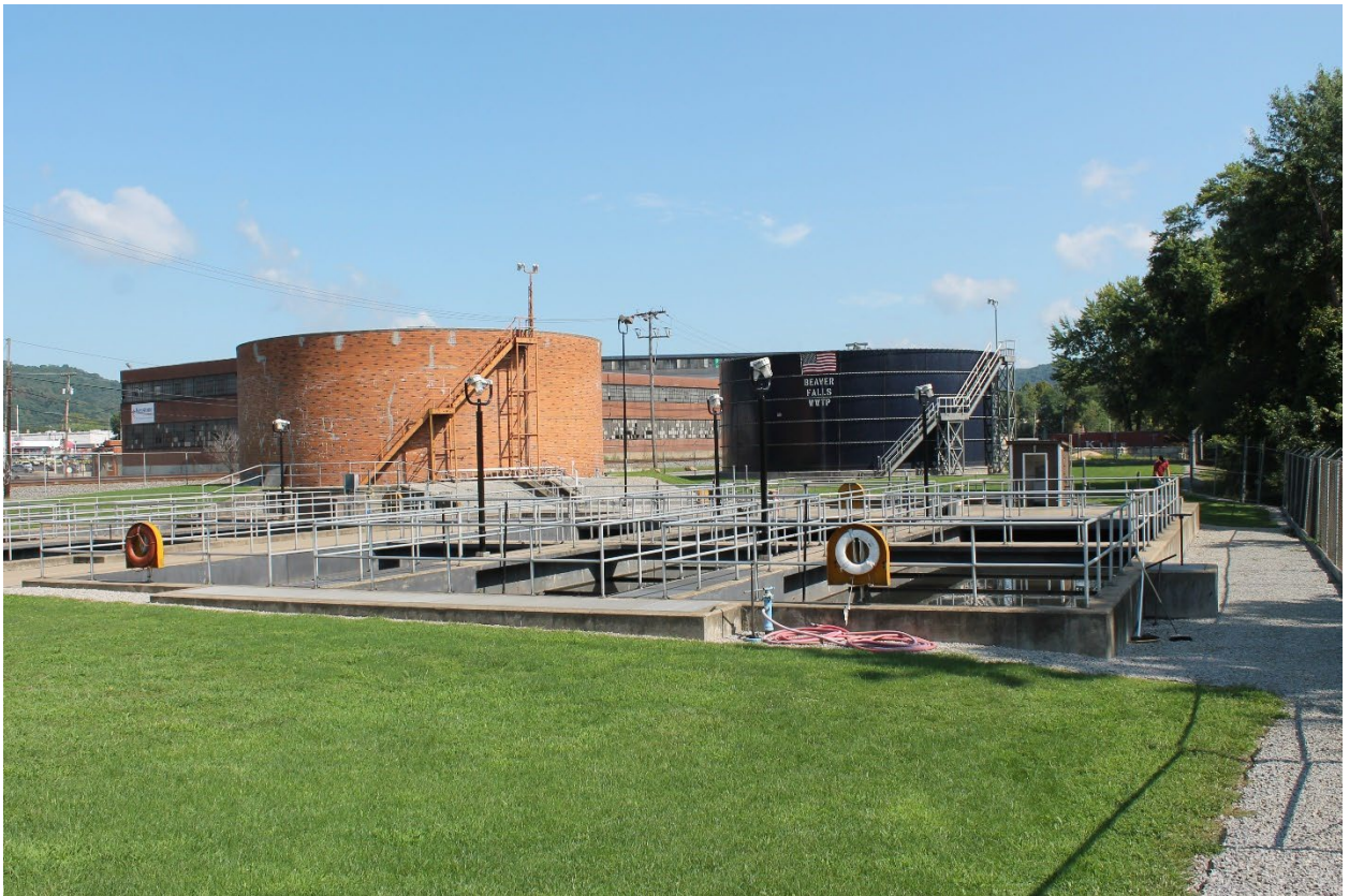
FIGURE 5.3 - 10: SECONDARY SETTLING TANKS AND OXIDATION TOWERS
