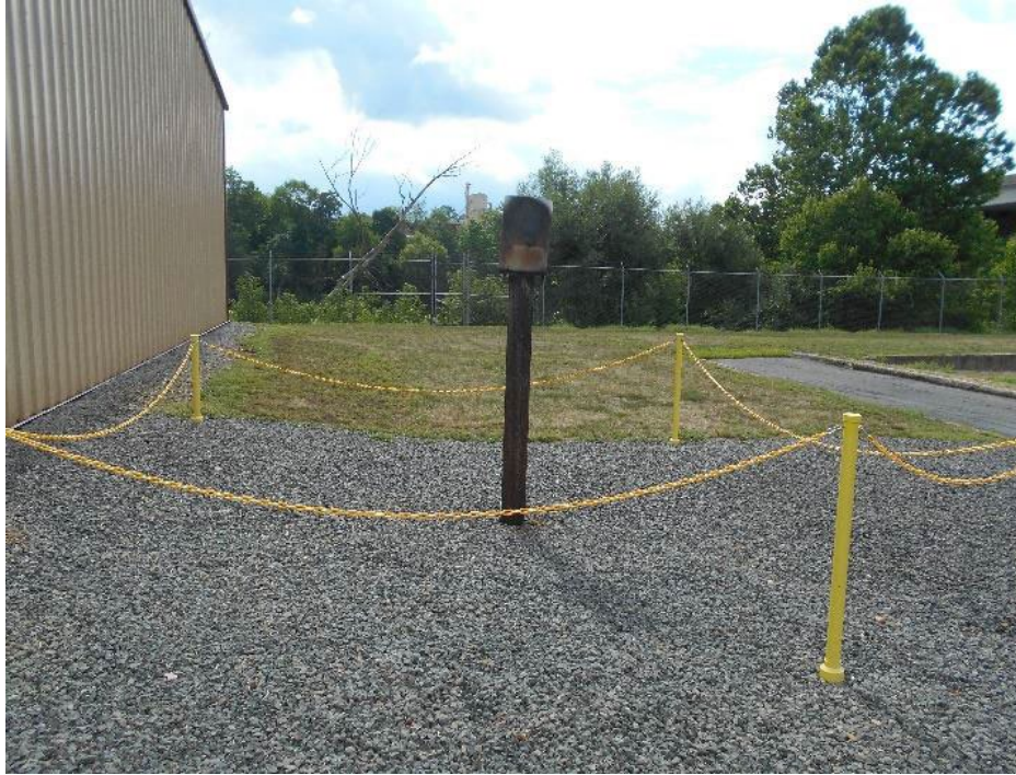
FIGURE 5.3 - 25: DIGESTER WASTE GAS BURNER
