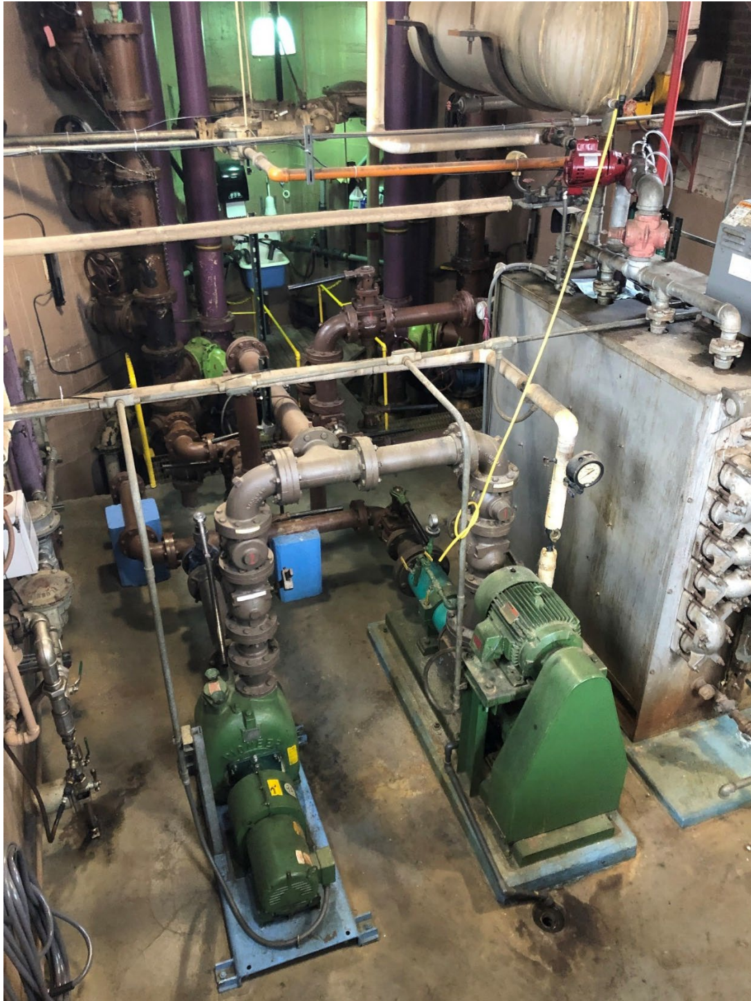
FIGURE 5.3 - 27: ANAEROBIC DIGESTER PIPING AND EQUIPMENT
