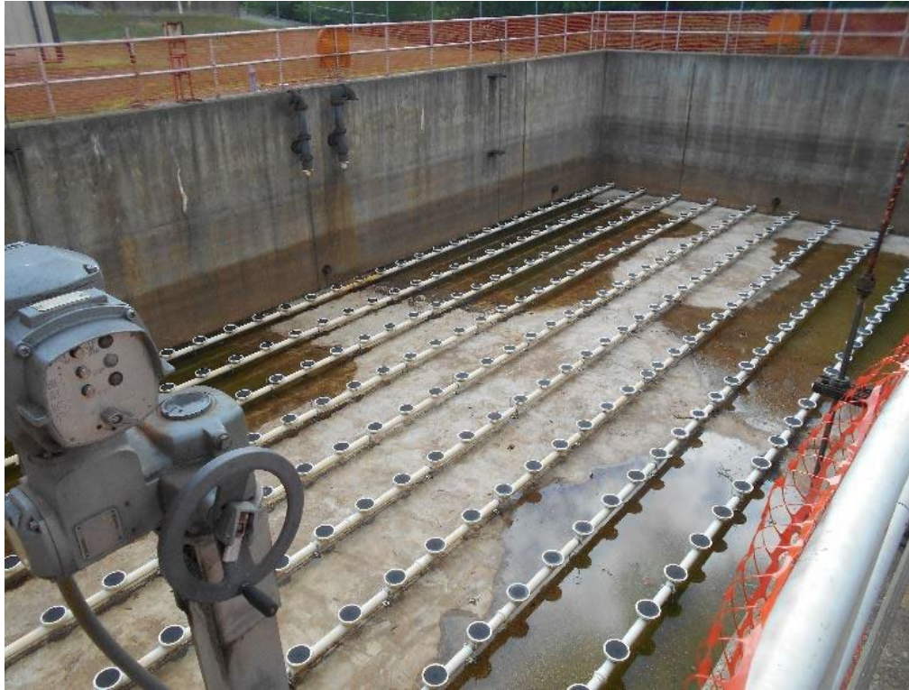
FIGURE 5.3 - 14: SLUDGE THICKENING TANK
