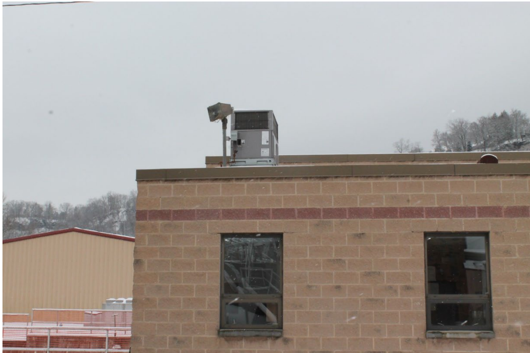
FIGURE 5.3 - 43: ROOF TOP AC UNIT OFFICE AREA
