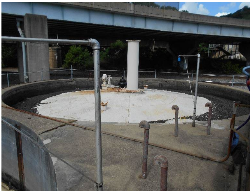
FIGURE 5.3 - 22: ANAEROBIC DIGESTER – TOP VIEW - FLOATING COVER
