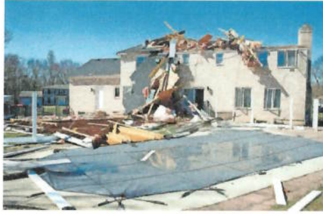
Tornado damage is seen in Howell, New Jersey, on Sunday. At least eight twisters struck southeastern Pennsylvania, southern New Jersey and Delaware on April 1. Noah K. Murray, for The Express-Times
