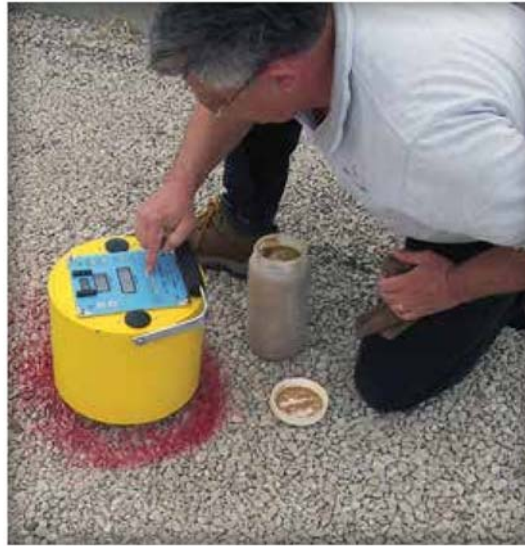
Figure 24. A base stiffness gauge can also be used to assess compacted density of aggregates.
