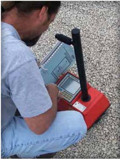
Figure 23. Density testing with a nuclear gauge in backscatter mode can help assess consistent density of the ASTM No. 57 base layer.
