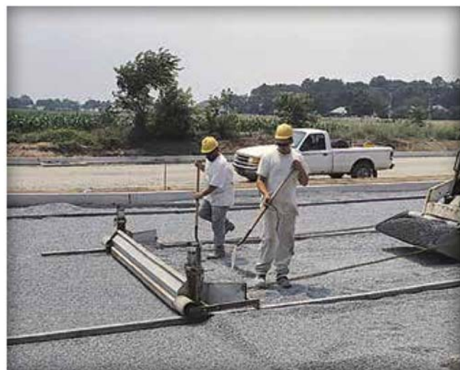
Figure 26. A screed beam pulled by equipment can be more efficient and productive.
