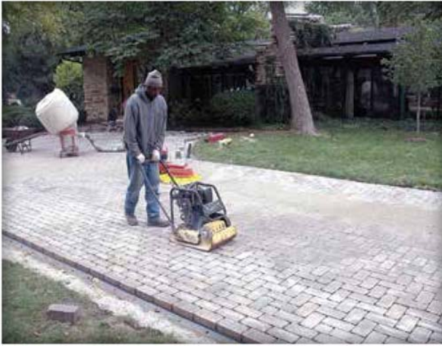
Figure 19. Edge restraint is spiked into the dense-graded base berms so it can hold the pavers in place during compaction and service.
