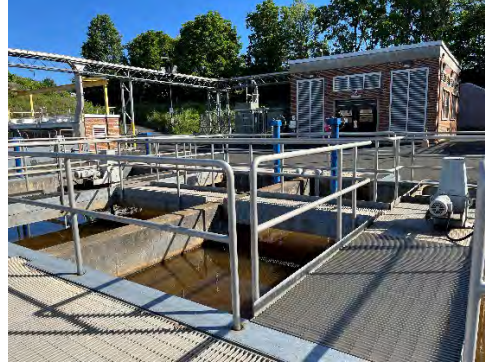
Flash Mix & Flocculation Tanks
