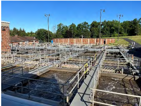
Aeration Tanks Stage 1
