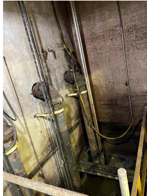
Wet Well and Piping
