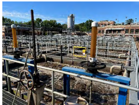
Aeration Tanks Stage 2
