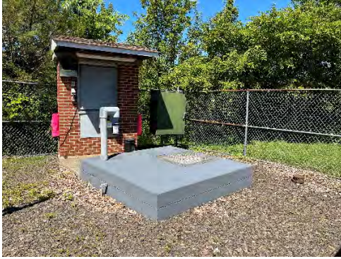
Control Panel and Valve Vault
