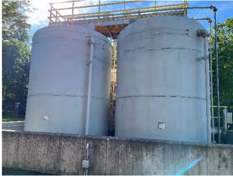
Ferric Chloride Storage Tanks
