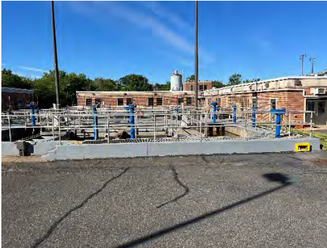
Flash Mix & Flocculation Tanks
