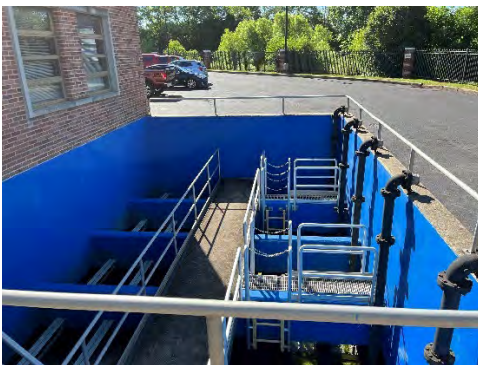
Chlorine Contact Tank
