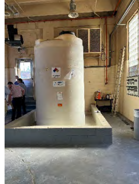
Poyaluminum Chloride Tank
