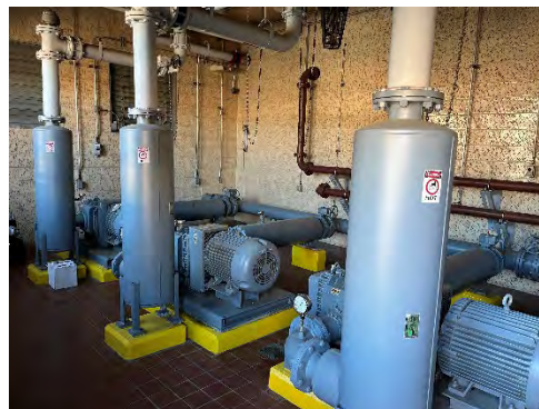
Sludge Storage Blowers
