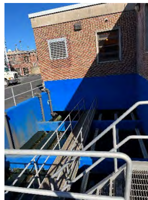
Chlorine Contact Tank
