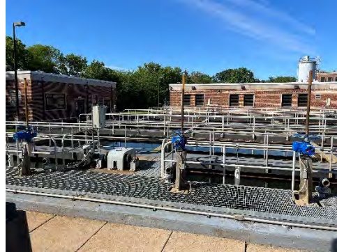
Final Settling Tanks
