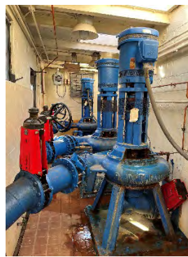
Trickling Filter Pump Station
