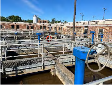
Flash Mix & Flocculation Tanks
