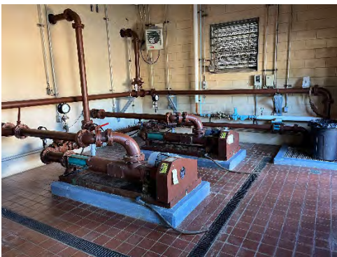
Sludge Transfer Pumps
