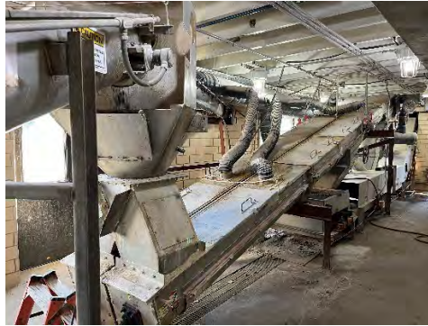
Sludge Cake Conveyors
