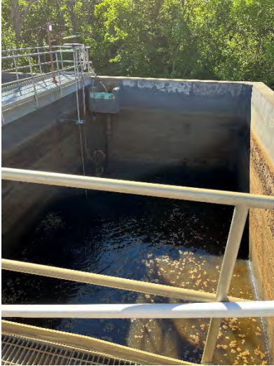
Sludge Holding Tanks
