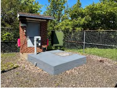
Control Panel and Valve Vault
