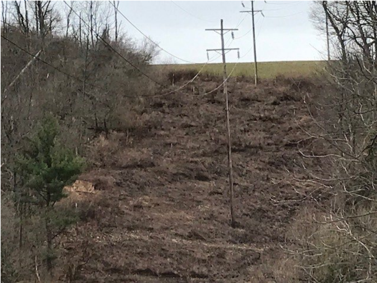
Figure 8: Sub-Transmission line that supplies the Lynnville Sub. Very good vegetation management.
