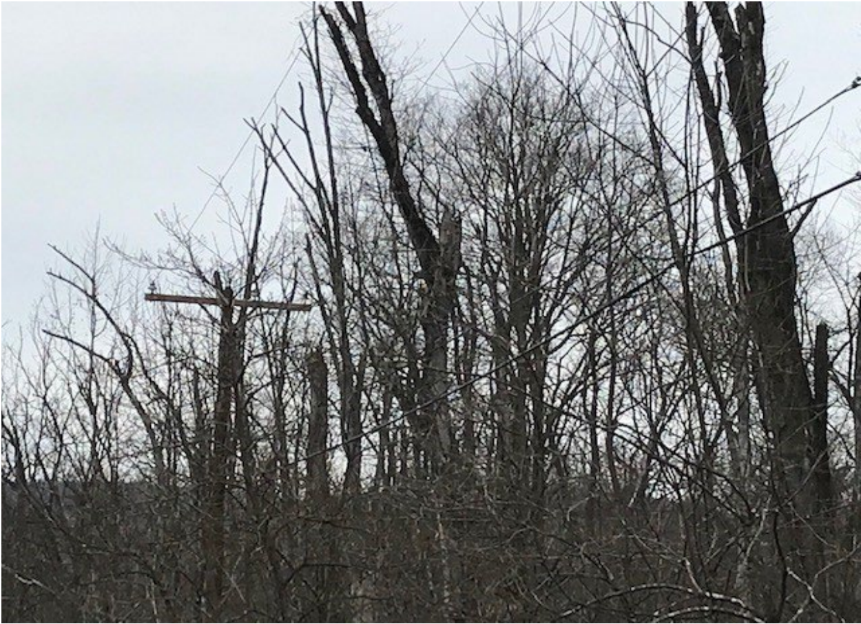
Figure 2: Three-phase OROW line section of 737-1 12kV. Note the floor vegetation and difficult access.
