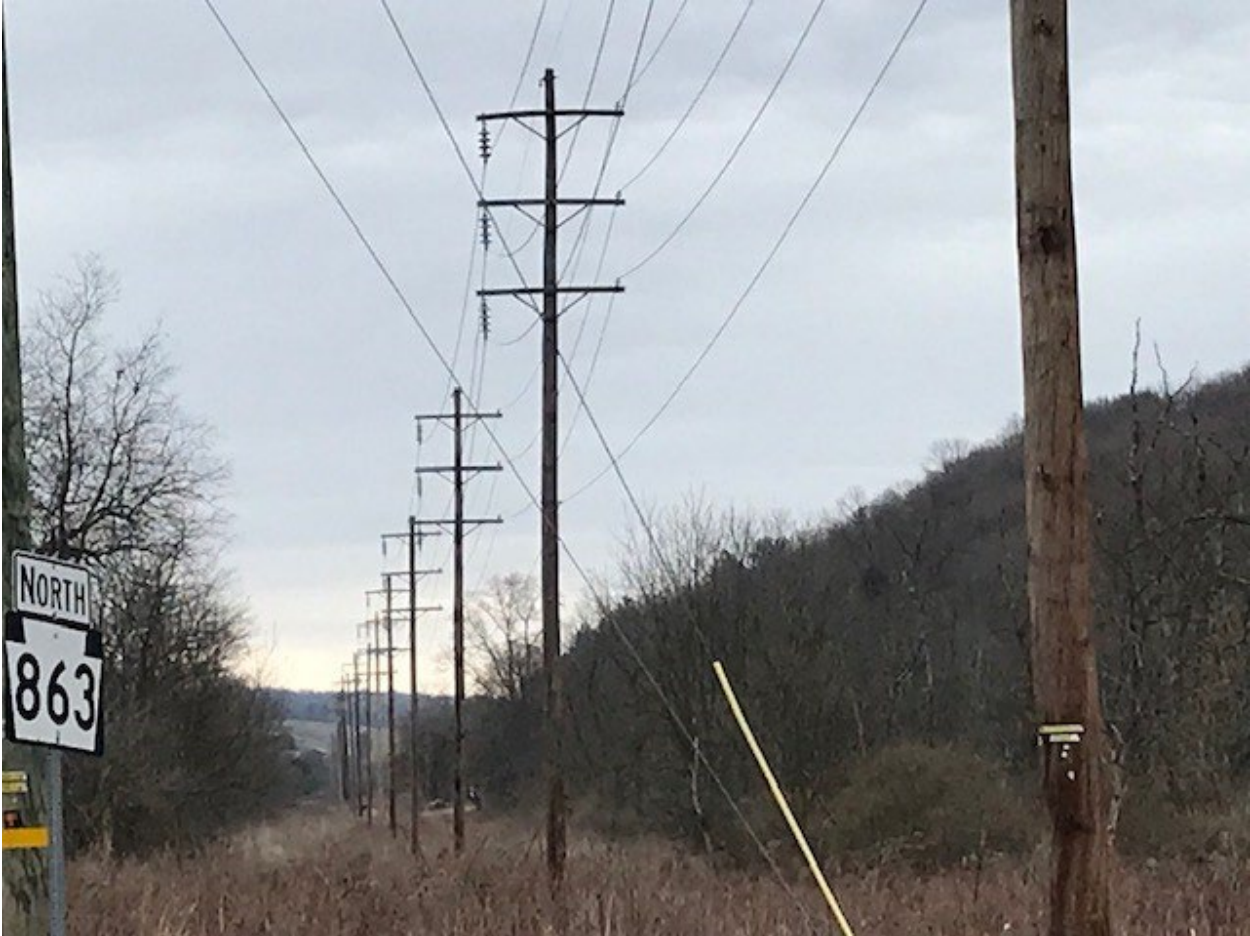
Figure 10: Dual Circuit line section near the Lynnville Sub. The Sub Transmission Feeder in on the left and the Lynnville 737-1 12kV line is on the right. Note very well-maintained line tree trimming.
