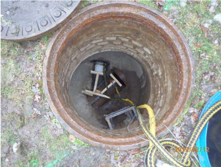
Greenville Sanitary Authority STP PA0027367 2/12/2019 Manhole prior to siphon chamber with plugs installed.
