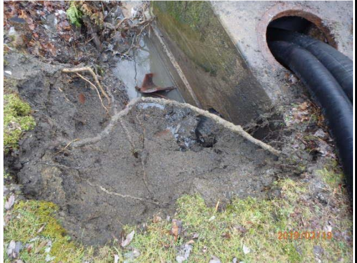
Greenville Sanitary Authority STP PA0027367 2/12/2019 Broken line and siphon chamber with plug installed.
