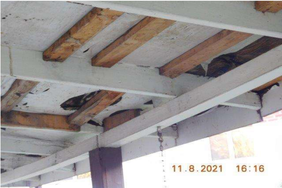
PHOTO 15 - AREA ABOVE PHOTO 14
