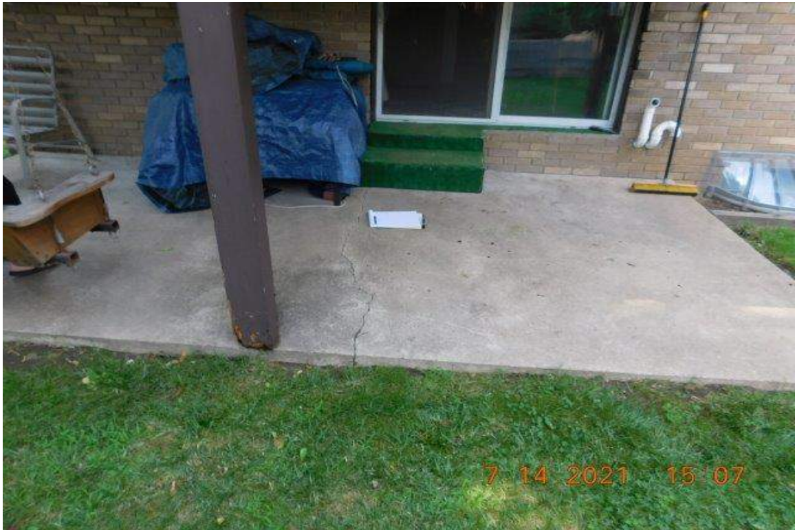
PHOTO 43 - DWELLING REAR WALL PATIO SLAB
