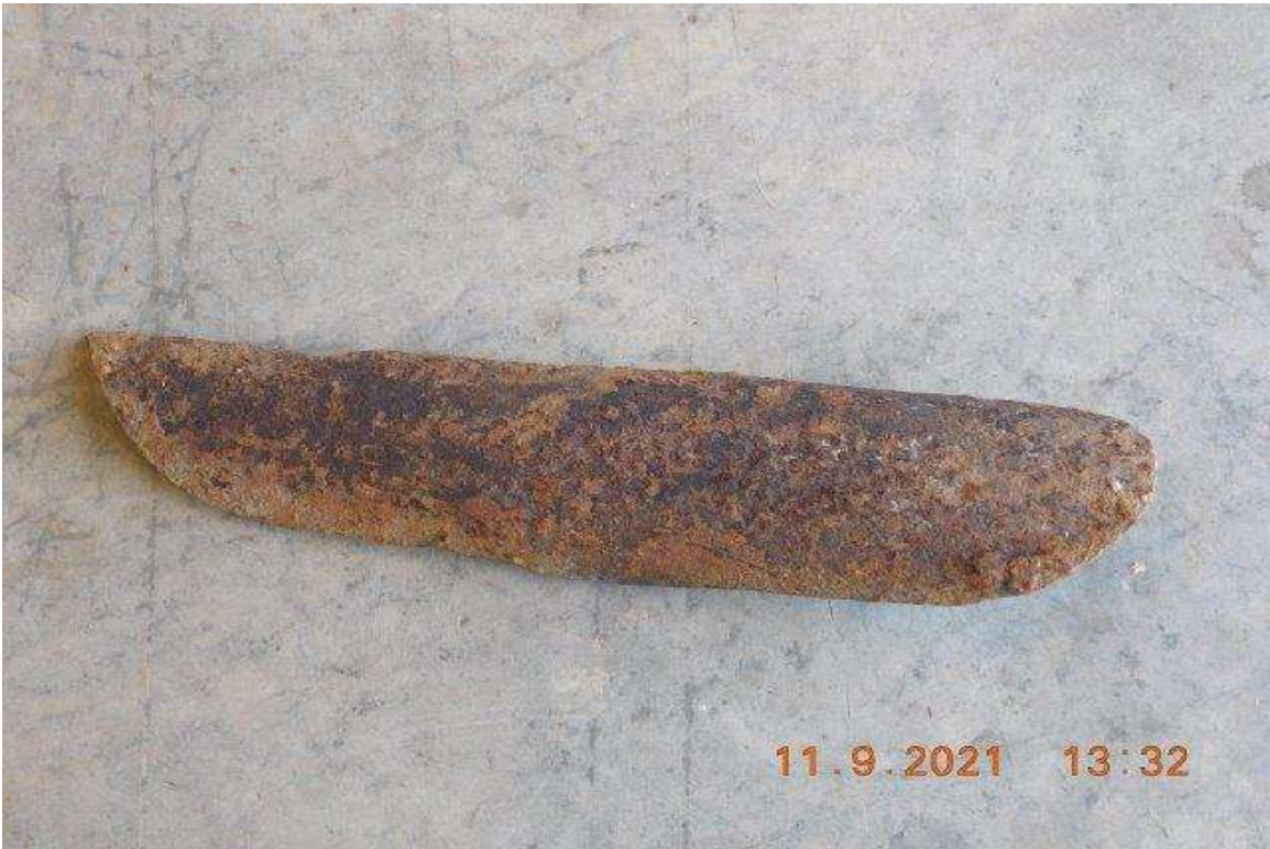
PHOTO 47 - EXTERIOR FACE OF PIECE OF BROKEN WATER LINE
