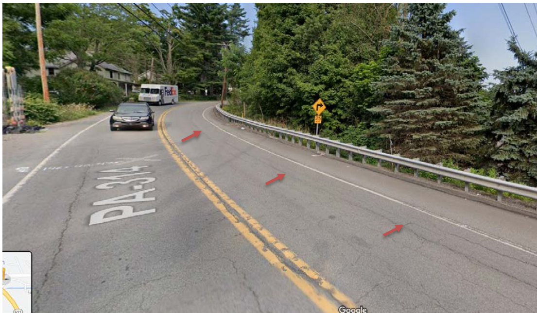
Photo 5 – Cracking in Roadway Along Utility Trench Limits, 2019
