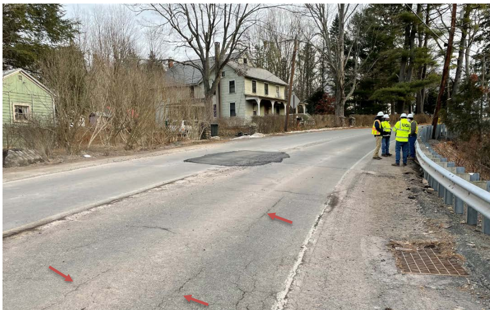
Photo 4 – Cracking in Roadway Along Utility Trench Limits
