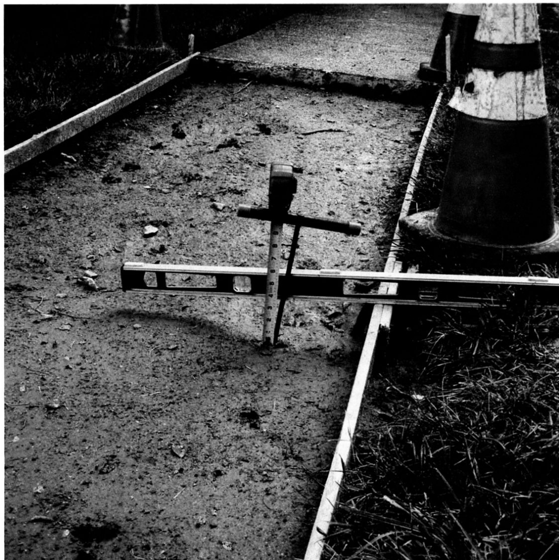
P1 339 PEPPER ROAD - SOIL PROBE DEPTH 38-INCHES BGS LOCATION ID : SLAB CENTER - STREET SIDE DATE/TIME : 20220613_1105AM_ FOTO ID : P6137584_RS_
