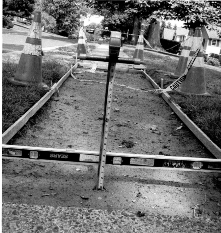
P5 339 PEPPER ROAD - SOIL PROBE DEPTH 26-INCHES BGS LOCATION ID : EAST SIDE OF SLAB - CENTER OF SLAB DATE/TIME : 20220613_1111AM_ FOTO ID :P6137590_RS_
