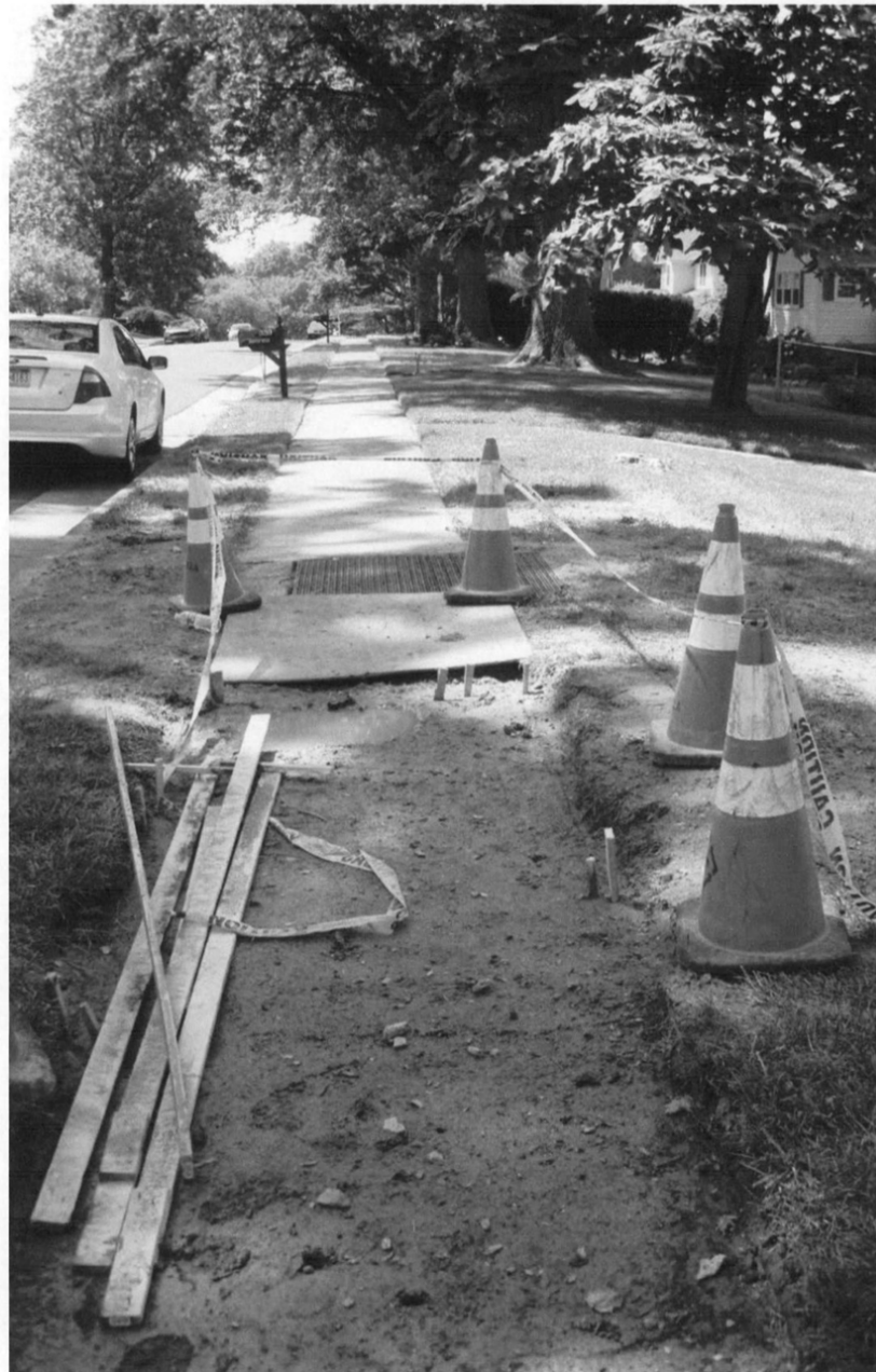
P10 339 PEPPER ROAD - SOIL PROBE SURFACE LOCATIONS LOCATION ID : OVERALL VIEW - SLAB CENTER FACING WEST DATE/TIME : 20220613_1452PM_ FOTO ID : P6137602_RS_
