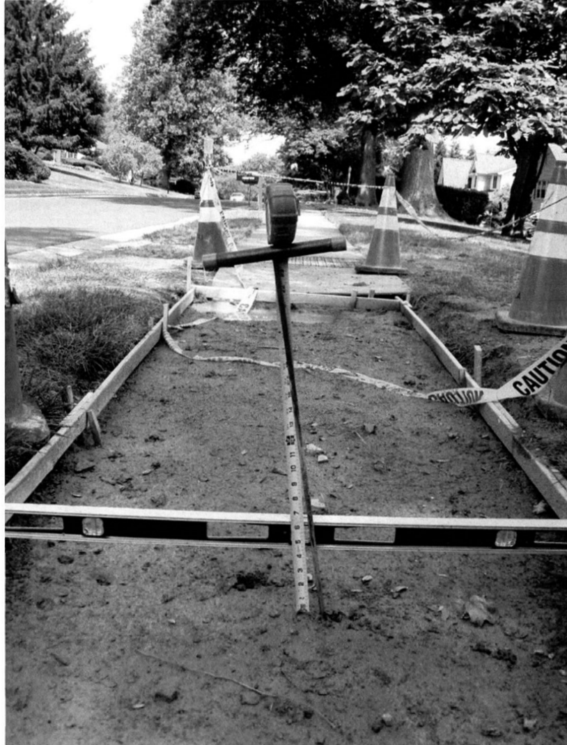
P3 339 PEPPER ROAD - SOIL PROBE DEPTH 24-INCHES BGS LOCATION ID : SLAB_CENTER LENGTH - WIDTH CENTER DATE/TIME : 20220613_1109AM_ FOTO ID : P6137586_RS_
