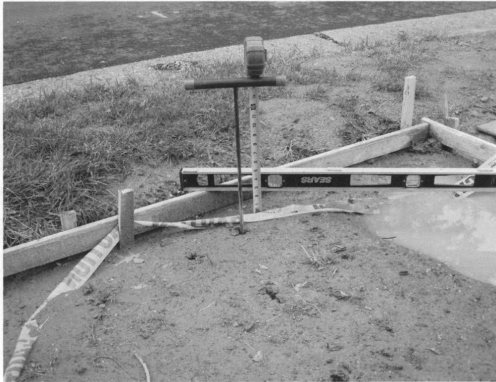
P0 339 PEPPER ROAD - SOIL PROBE DEPTH 34-INCHES BGS LOCATION ID : WEST END AT BURIED ELECTRIC TRANSFORMER DATE/TIME : 20220613_1103AM_FOTO_ID: P6137575_RS_
