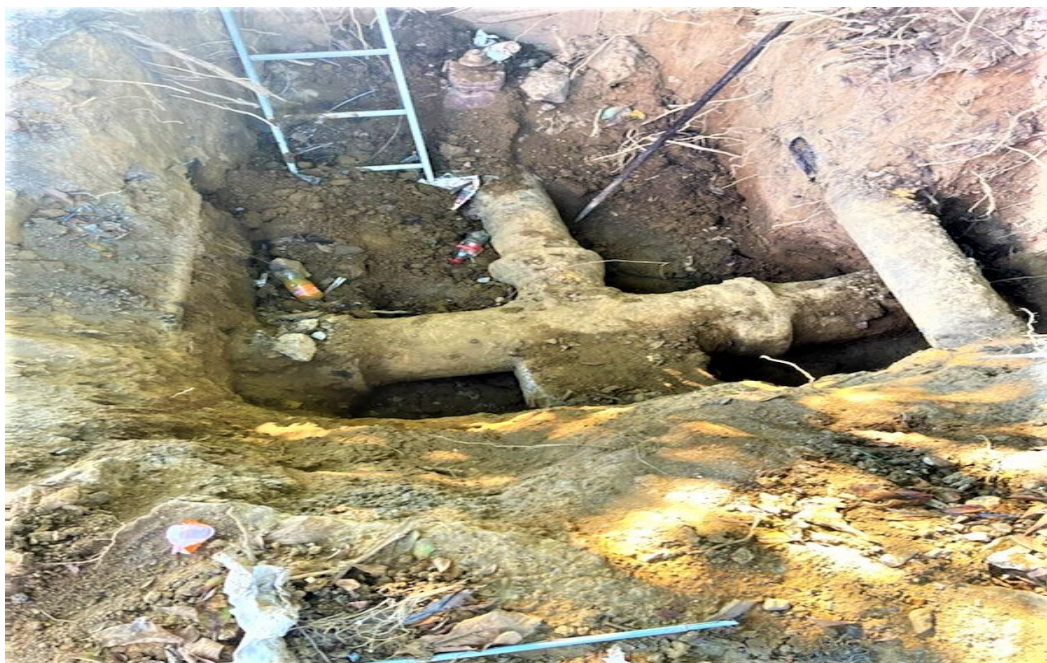
Figure 4: View of the PECO ducts that are encased in concrete Source: USIC
