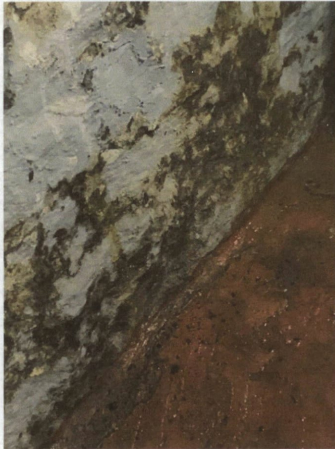
Water damage in basement bathroom along Argonne Avenue side of house
