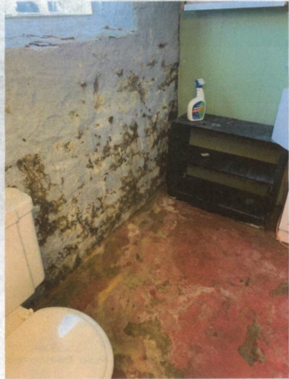
May 2022 evidences wet, moldy basement all along inside walls along Argonne Avenue (alley) side of home
