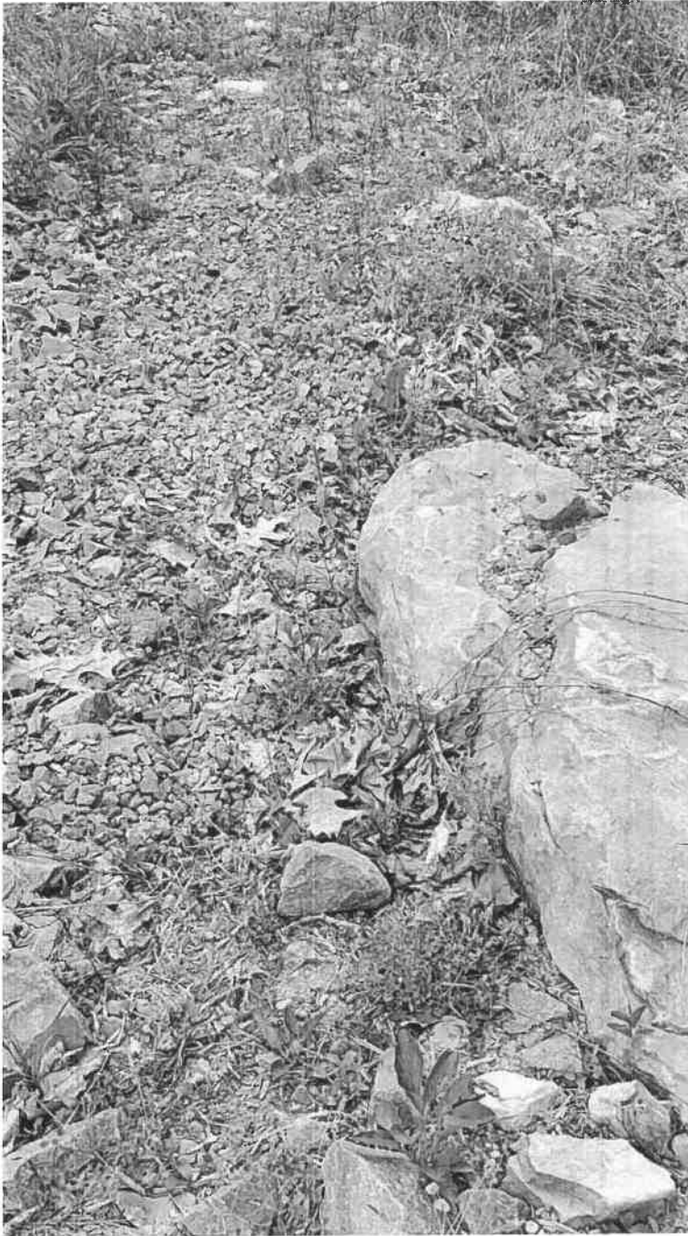
June 6, 2022 Photograph 15 – Access Road Stone that washed off access road onto former vegetated area
