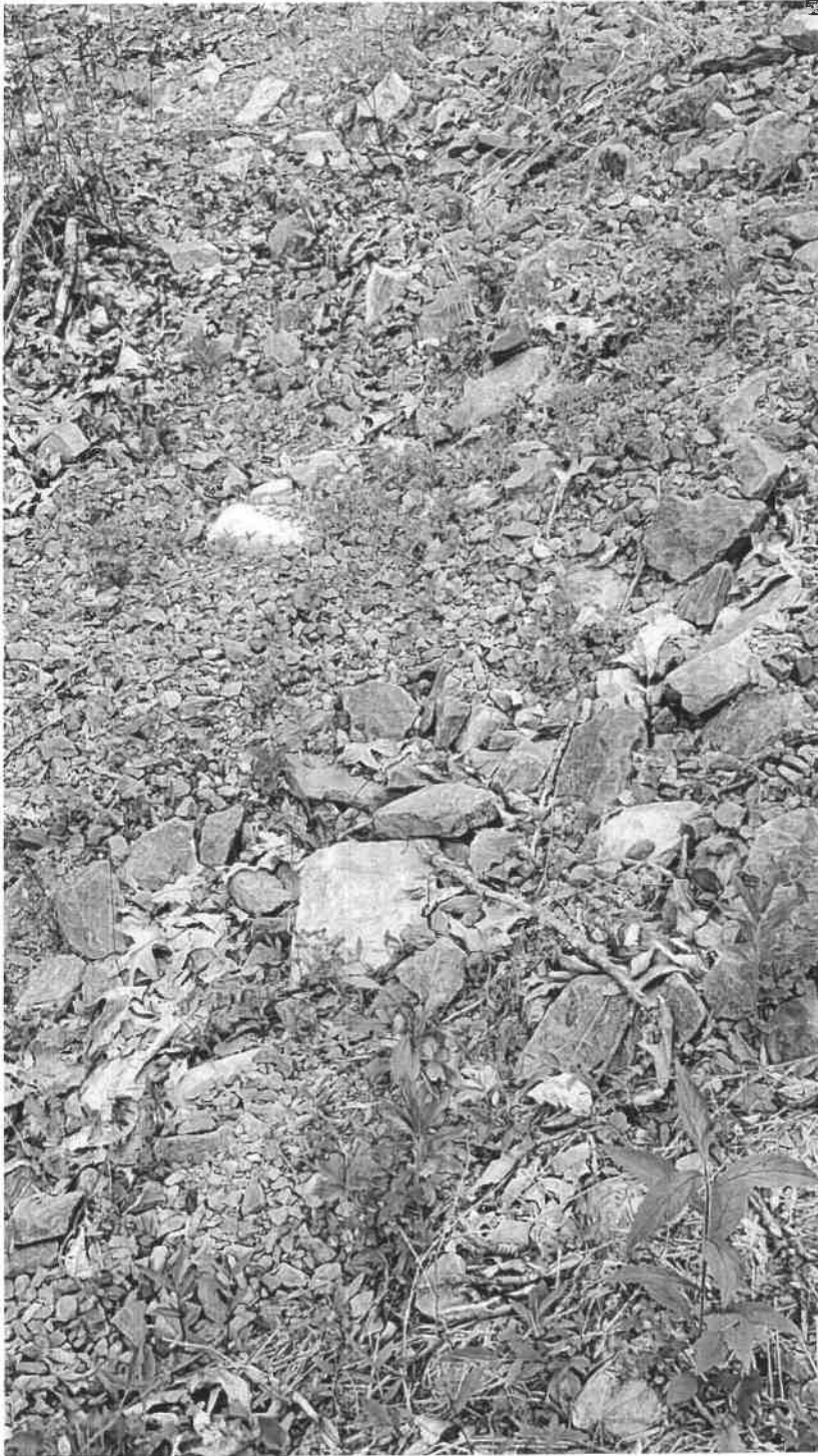
June 6, 2022 Photograph 14 – Access Road Stone that washed off access road onto former vegetated area
