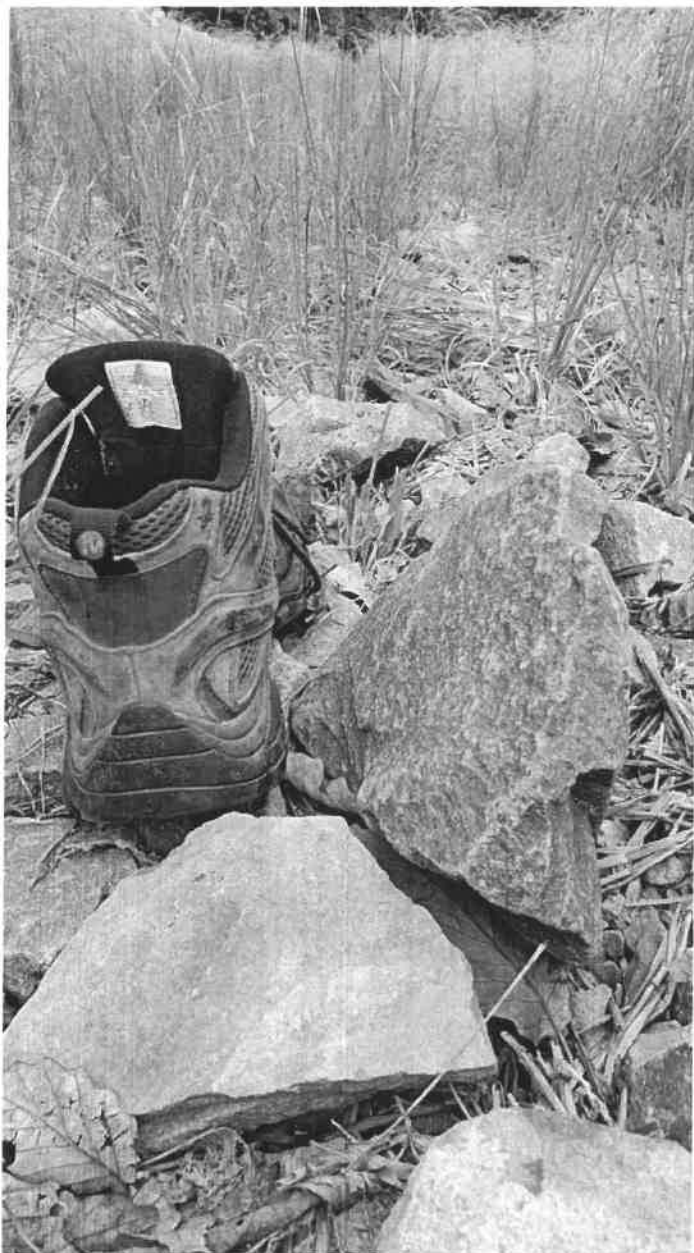
Sharp Protruding Rip Pap on Access Road
