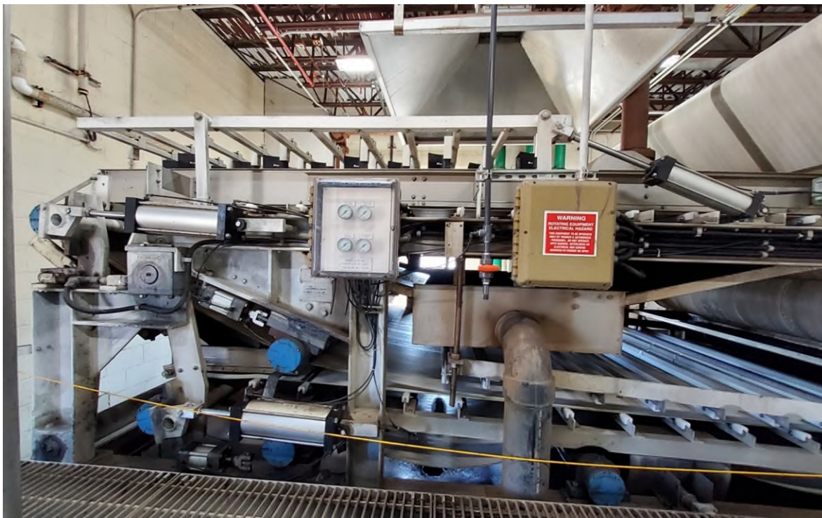
Belt filter press from North side close.
