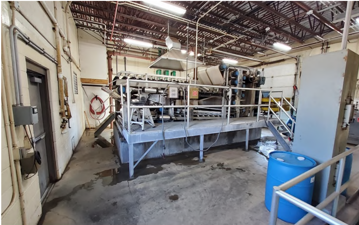
Belt filter press from North side of room.
