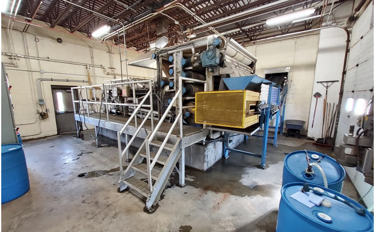
Belt filter press from West side of room.
