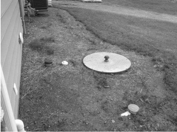
Photo above-Grinder pump station with fiberglass tank and stainless steel lid installed outside a home
