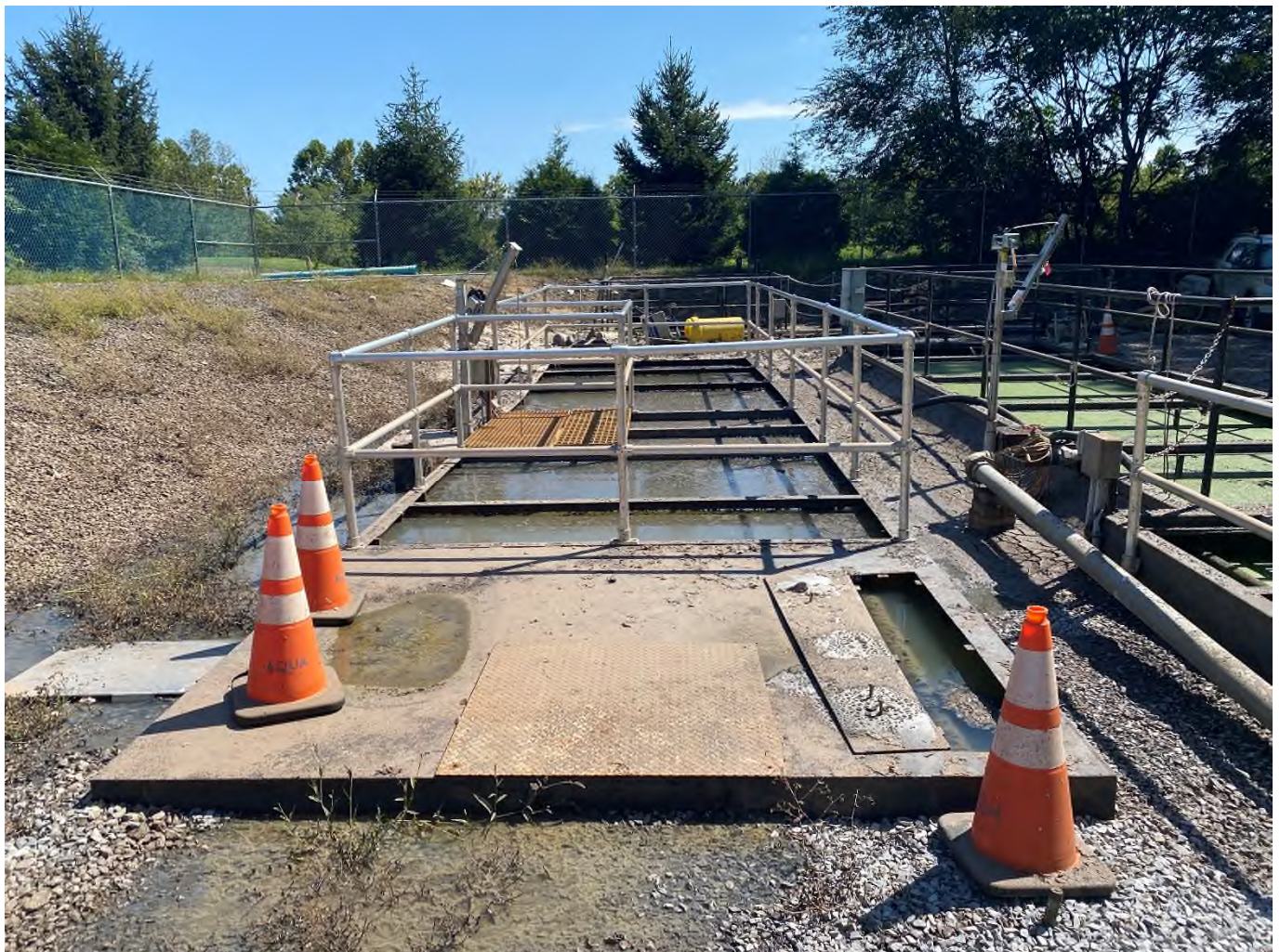
VIEW FROM WEST LOOKING EAST OF EQ TANK IN CENTER AND SLUDGE HOLDING TO THE RIGHT AFTER FLOOD WATERS RECEDED.
