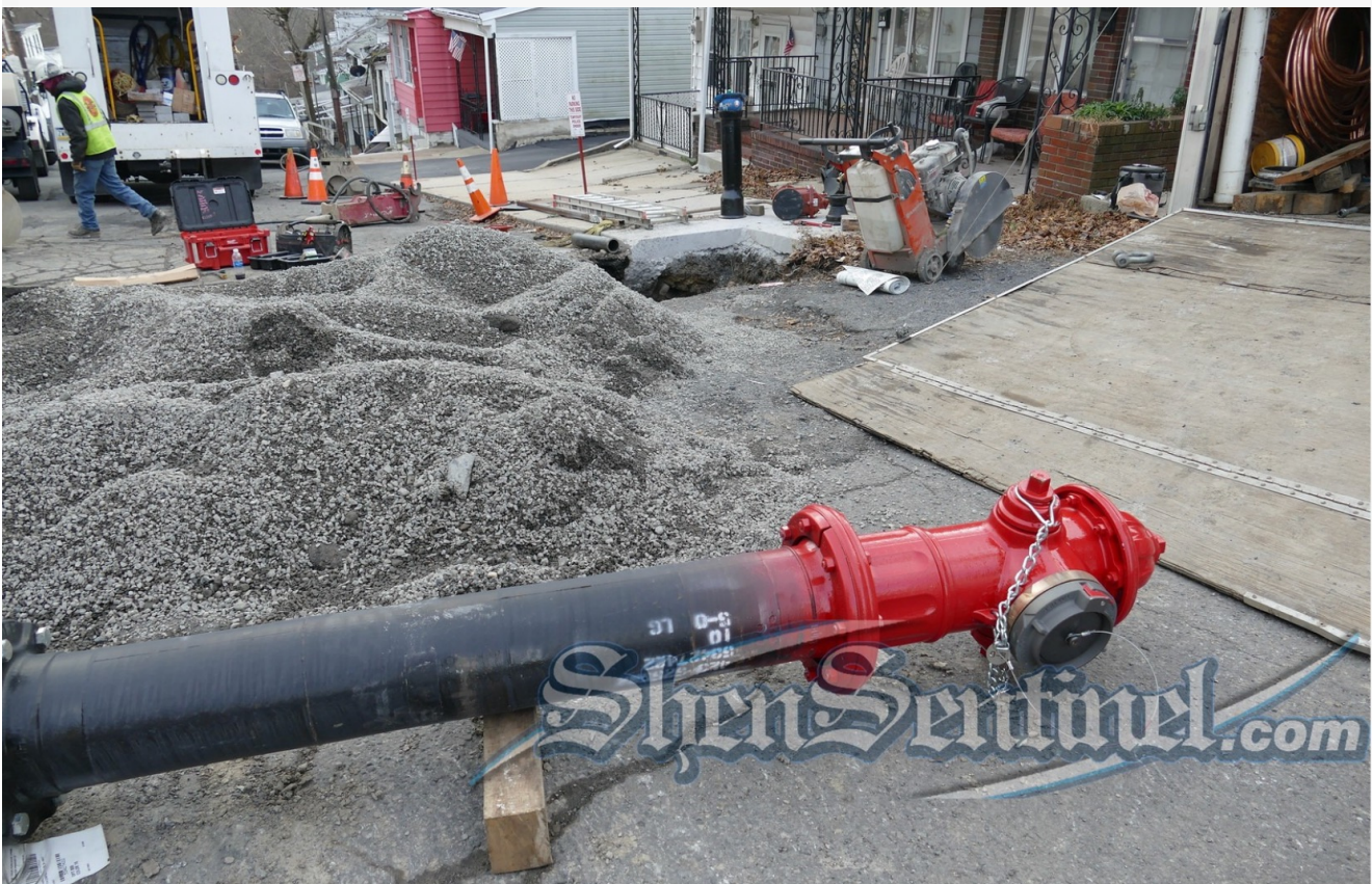
KAYLEE LINDENMUTH / SHENANDOAH SENTINEL - The worksite at Chester and West Streets in Shenandoah where a contractor was replacing a fire hydrant on Dec. 20, 2023.
