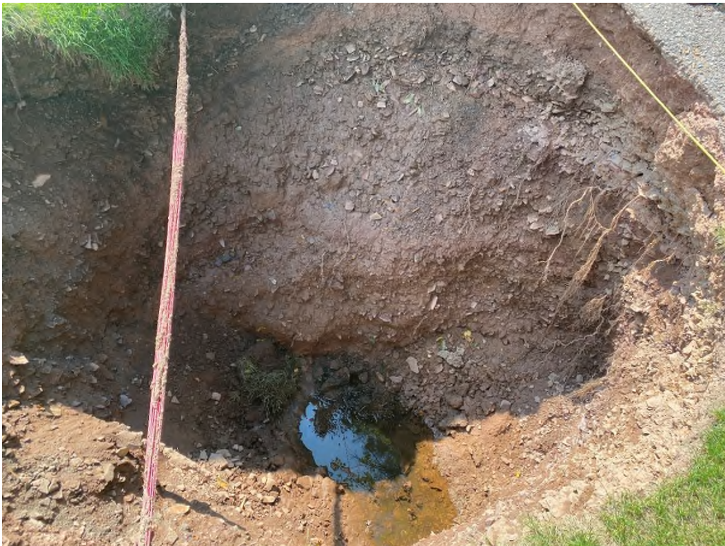
SINKHOLE APPROXIMATELY 12 FEET IN DIAMETER AND 12 FEET DEEP.
