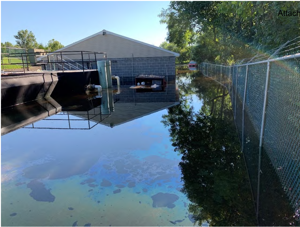
SUBMERGED WASTEWATER TREATMENT PLANT VIEW FROM WEST (ENTRY) SIDE OF PLANT LOOKING EAST.
