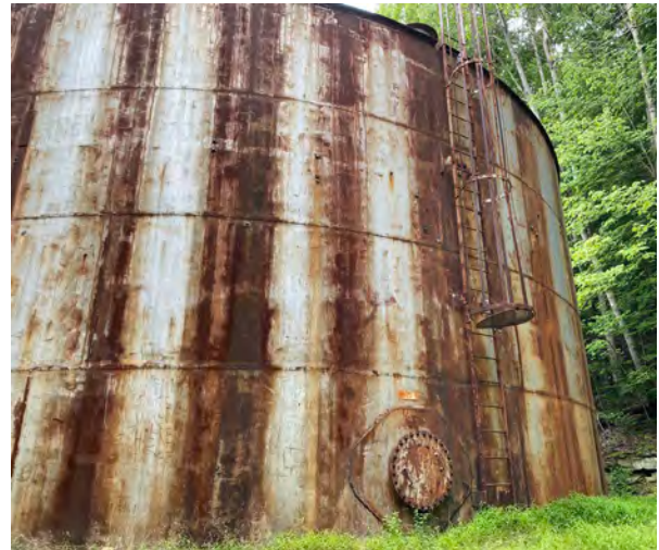
PHOTO #2: Coating is in poor condition with rust and erosion.
