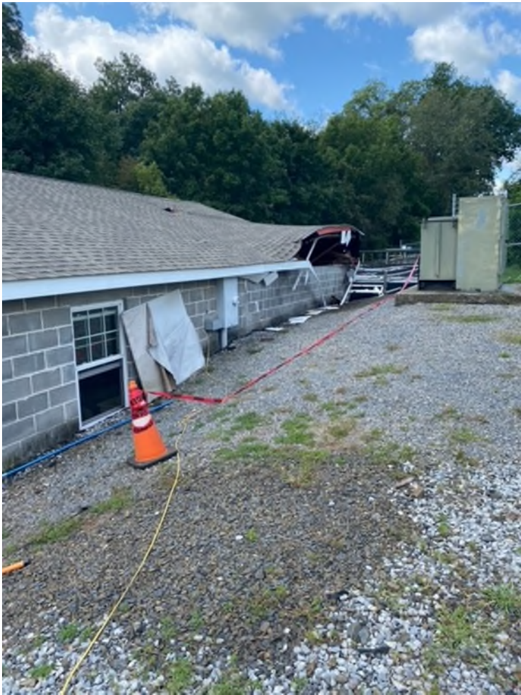
CONTROL BUILDING ROOF DAMAGE DUE TO THE FLOATING OF THE RAPID SAND FILTER TANK / ULTRAVIOLET DISINFECTION SYSTEM IN ABOUT HALF OF THE BUILDING.
