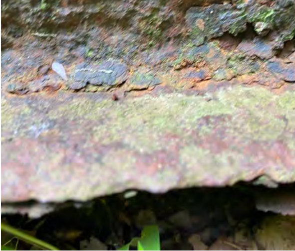
PHOTO #13: Corrosion along bottom of sidewall.
