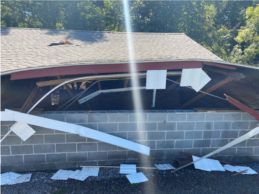
RAISED UP ROOF TRUSSES AND ROOF RESULTANT FROM TANK FLOATING IN THE CONTROL BUILDING.
