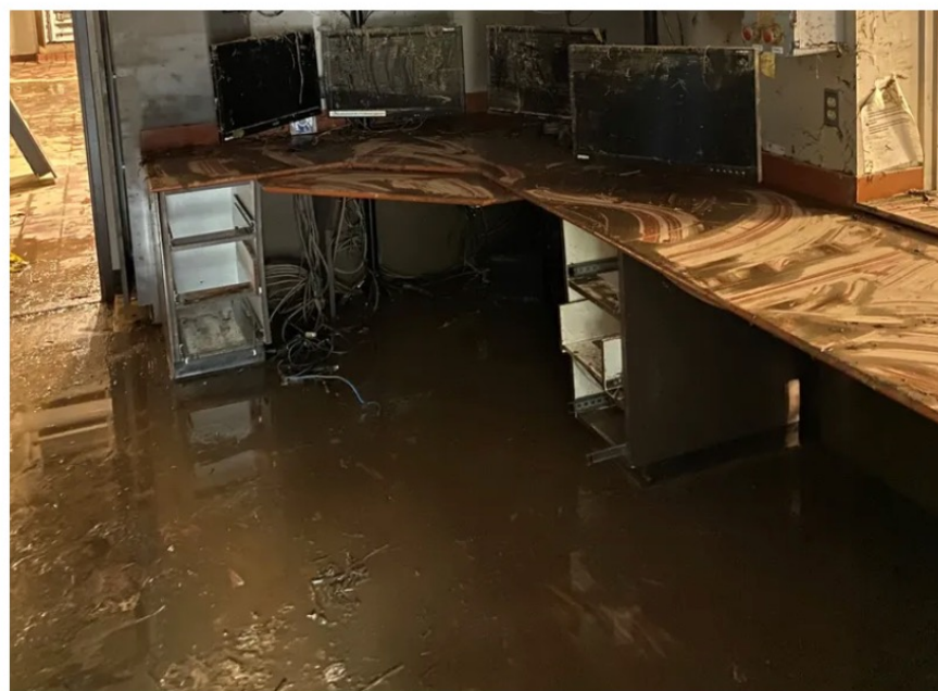
The control room where operators monitored plant operations was destroyed. Photo credit Aqua Pennsylvanianormal
