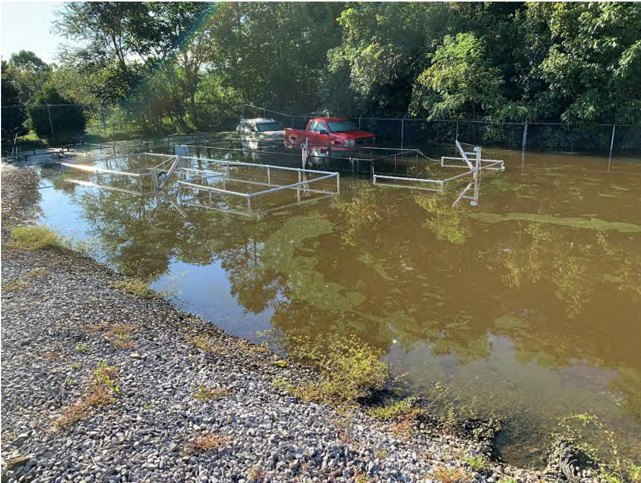
SUBMERGED WASTEWATER TREATMENT PLANT VIEW FROM SOUTHEAST SIDE OF PLANT LOOKING IN A SOUTH EASTERLY DIRECTION. GOLF COURSE CARTWAY BERM NEAR CULVERT SINK HOLE IN BACKGROUND (BEHIND WHITE CAR).
