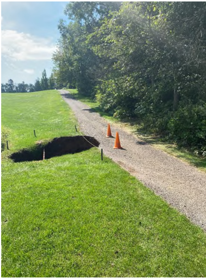
SINKHOLE LOCATION ON GOLF COURSE PROPERTY OVER TOP OF CULVERT. NHSC PROPERTY LINE AT WOODS/FENCE LINE TO THE RIGHT. EARTH WASHED INTO THE COLLAPSED CULVERT SUBSTANTIALY BLOCKING IT.
