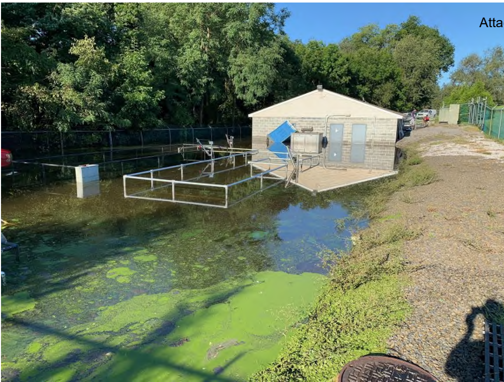
SUBMERGED WASTEWATER TREATMENT PLANT VIEW FROM EAST SIDE OF PLANT LOOKING WEST. RAILINGS ON EQ AND SLUDGE HOLDING TANKS CAN BE SEEN. GENERATOR IS TO THE LEFT OF CONTROL BUILDING DOOR.
