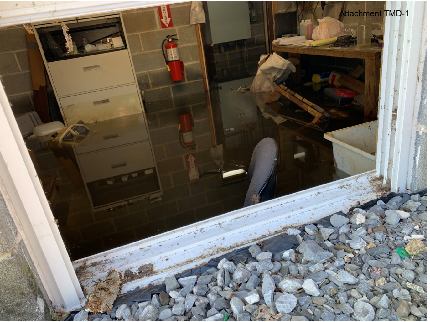
VIEW INTO CONTROL BUILDING OFFICE WHILE STILL UNDER WATER.
