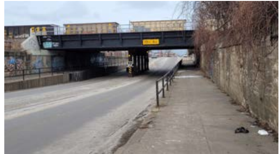
While railroads transport freight, railroad bridges often cause difficulties for large trucks underneath creating breaks in urban freight corridors.
