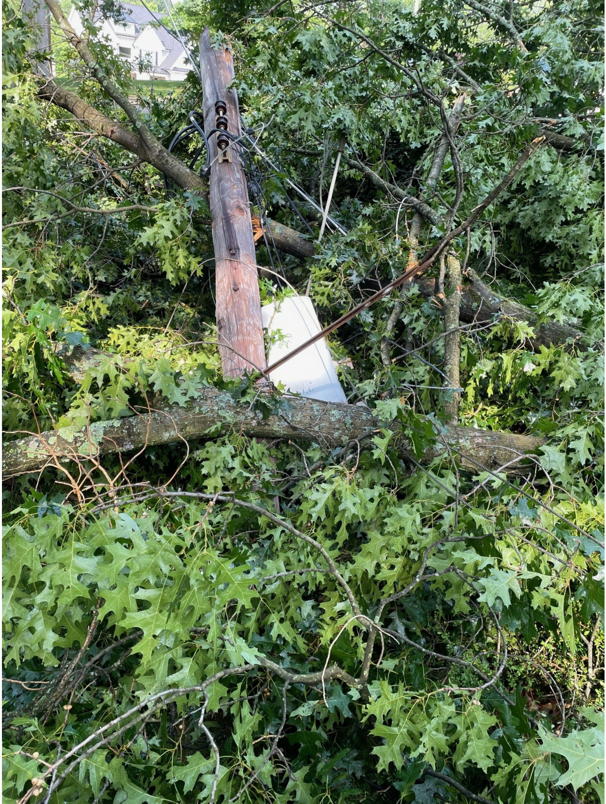
Figure 4: DLC storm photos, Babcock Blvd in McCandless
