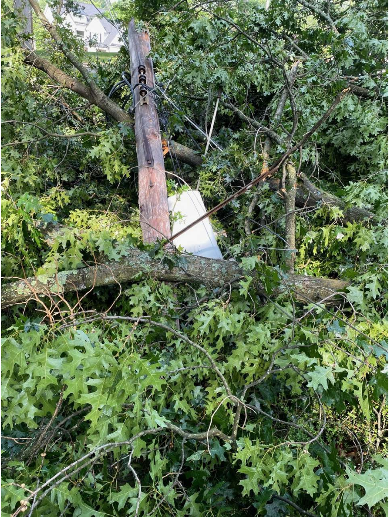
Figure 4: DLC storm photos, Babcock Blvd in McCandless
