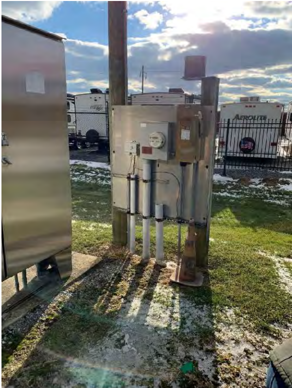
Northern Pump Station
