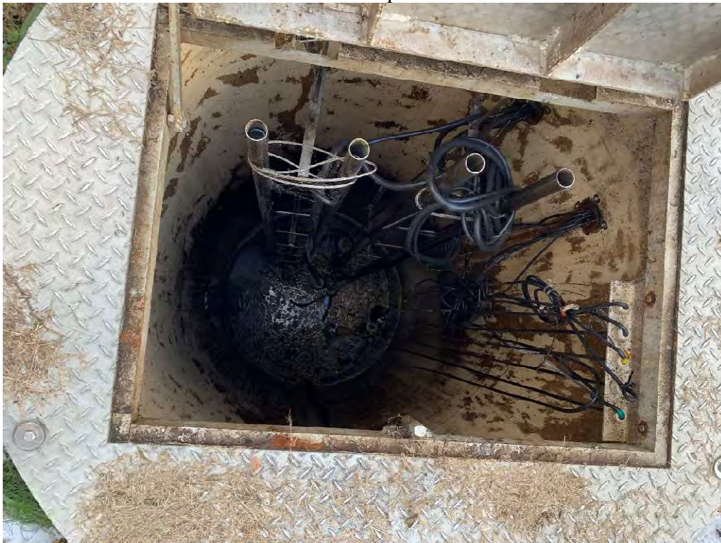
Southern Pump Station
