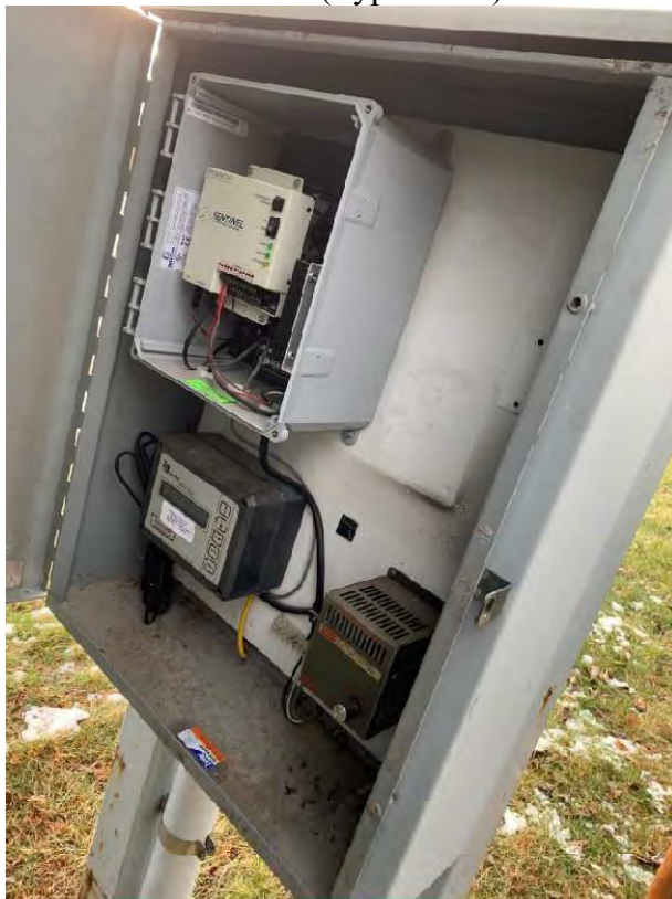
Meter Pit (Typical – 4)
