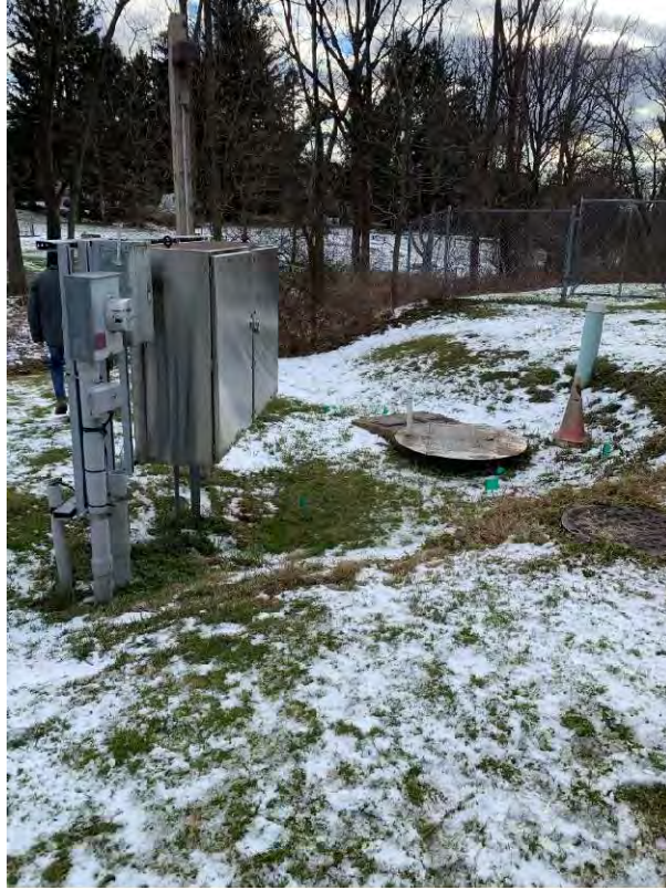
Southern Pump Station
