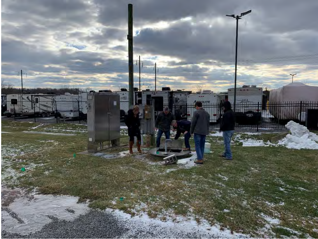
Northern Pump Station
