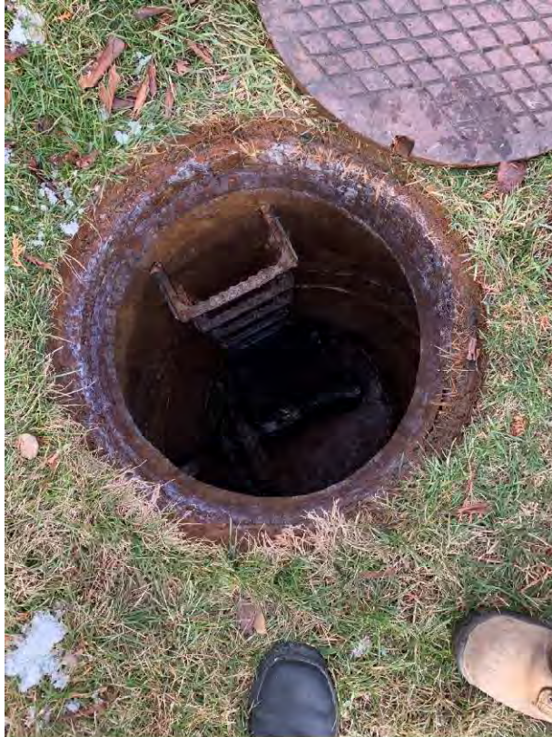
Meter Pit (Typical – 4)
