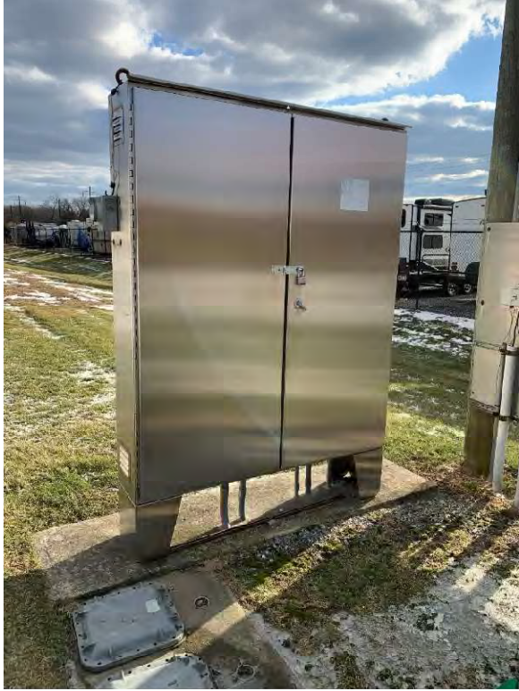
Northern Pump Station
