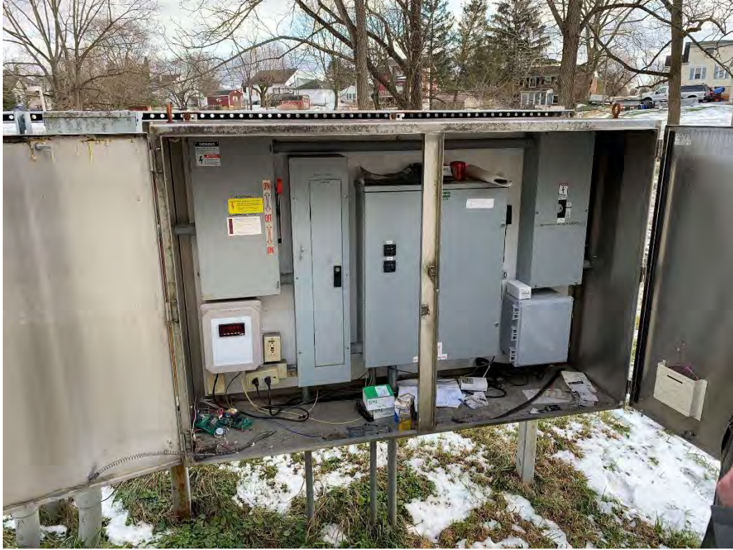
Southern Pump Station
