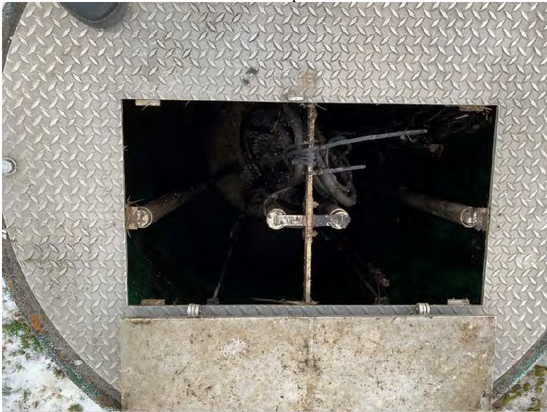
Northern Pump Station
