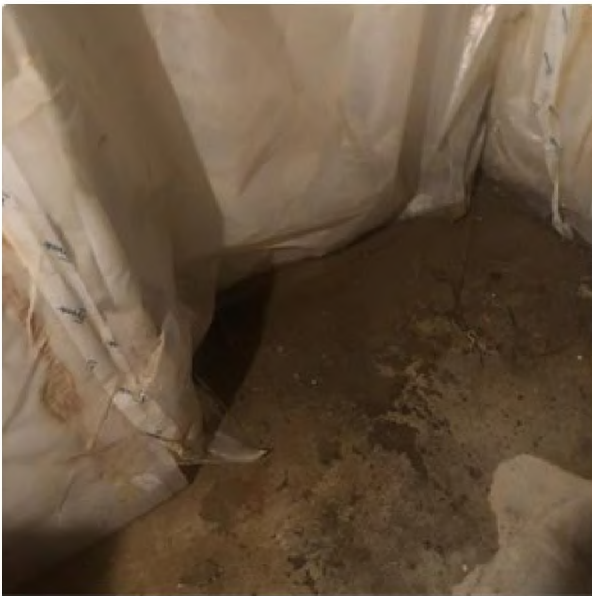
Flooding Under Window where meter was installed from below ground
