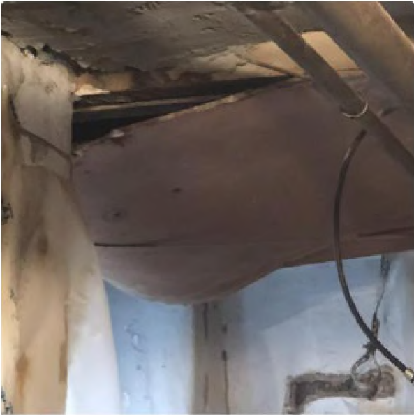
utility room ceiling from stone missing in chimney water flowing down on outside of liner
