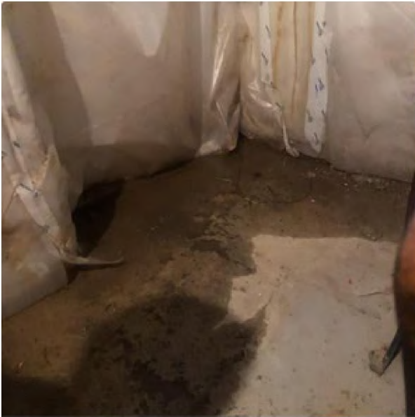
flooding at floor and area where meter was installed and reinstalled
