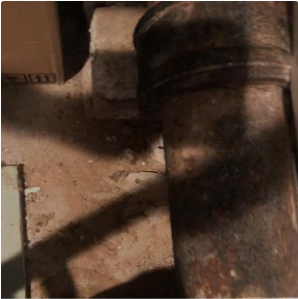
Pipe next to heater
