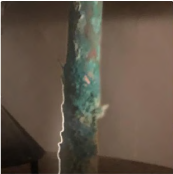
hot water heater pipe corrosion from multiple leaks
