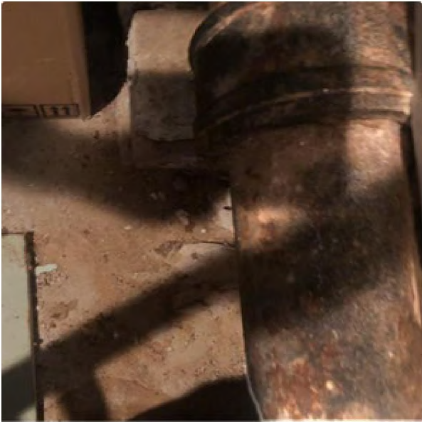
Pipe next to heater
