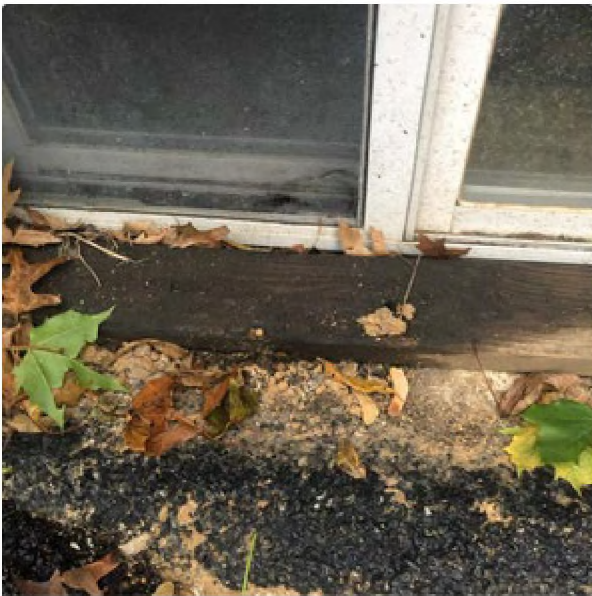
Window/ Foundation patch
