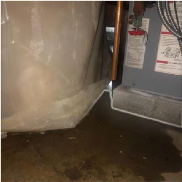
flooding around heater
