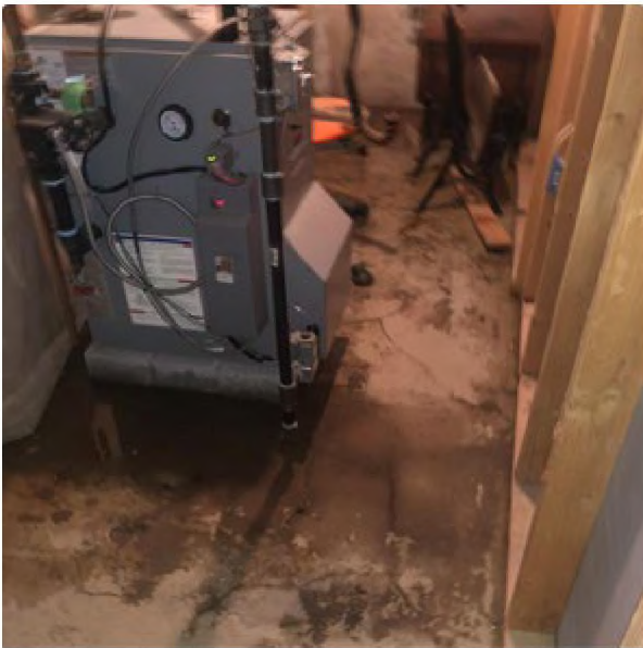
Utility Room /heater
