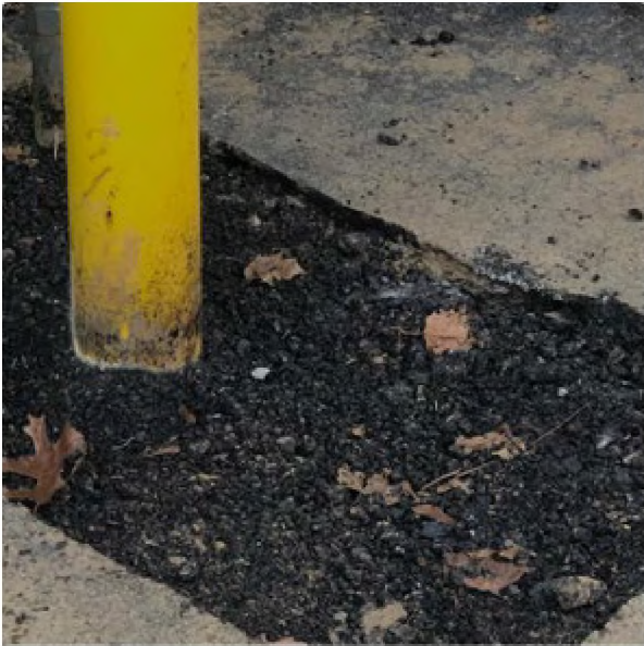
Sinking Line mark on pole
