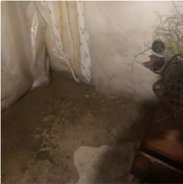
Under window and right wall where meter was removed
