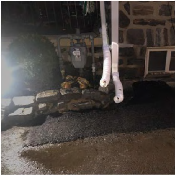
flooding during rain after relocating
