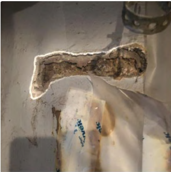
Wall to right of basement (utility room) window where meter was originally ( not repaired/ patched)
