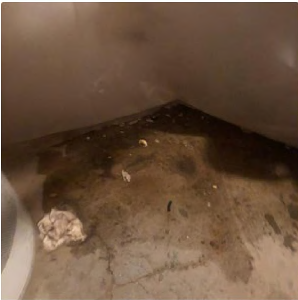
flood reaching water heater located to the left of chimney wall
