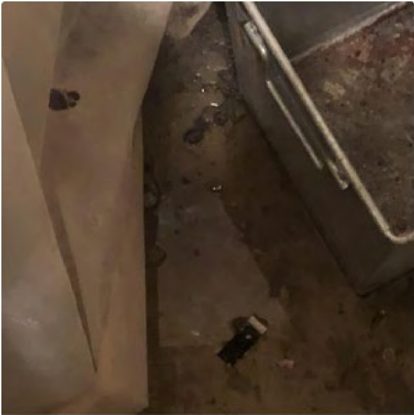
Along chimney floor
