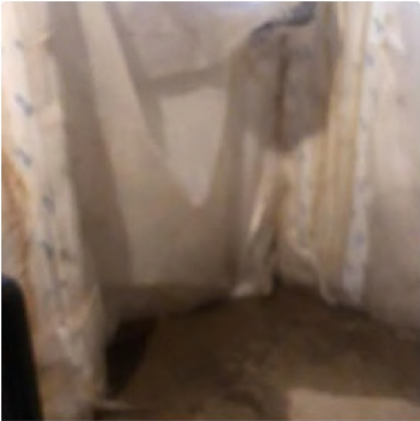
Flooding from ground level under window where meter was relocated
