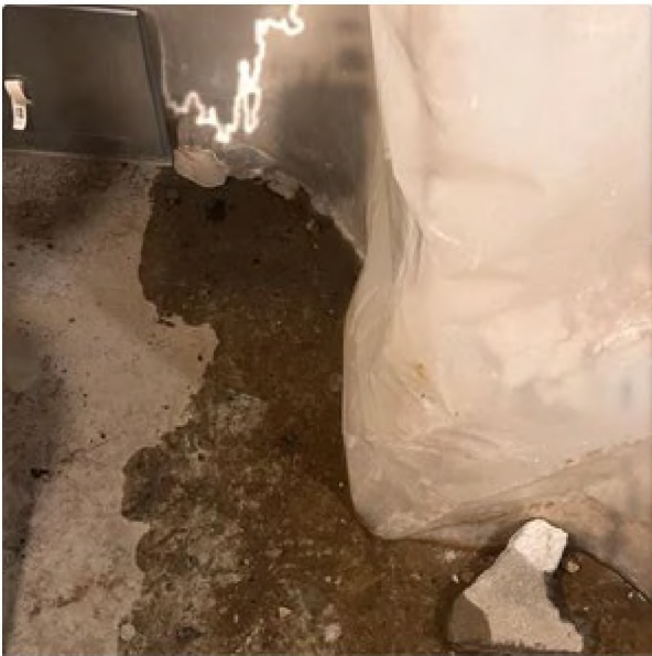
stone knock out chimney still flooding
