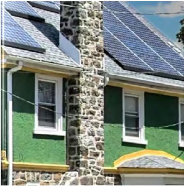
hole in chimney
