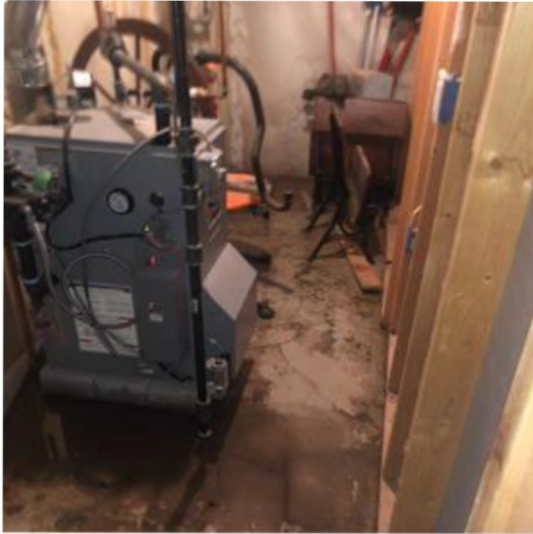
Utility Room with heater/and antics along sons bedroom door
