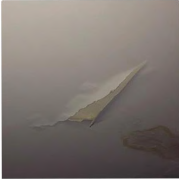
pic of daughter room that runs along chimney damaged (stone knocked out side) ceiling damage
