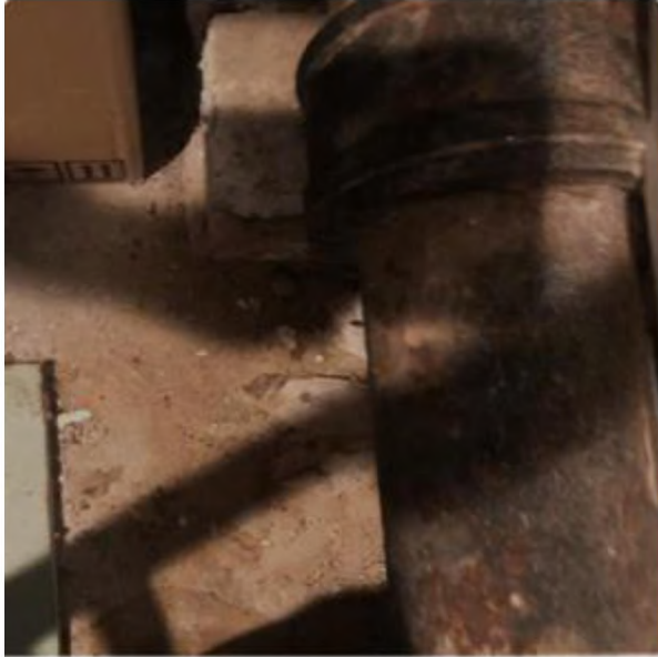
Pipe next to heater
