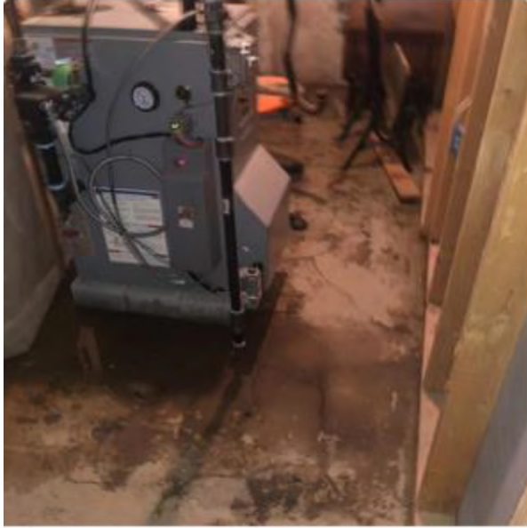
Utility Room /heater
