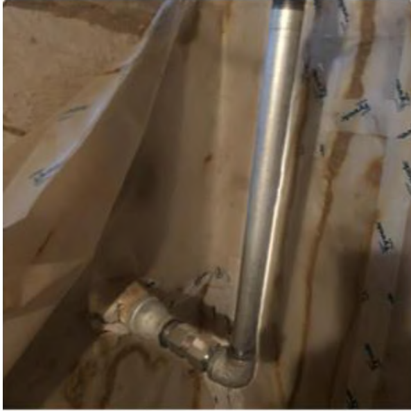
Gas Meter pipe
