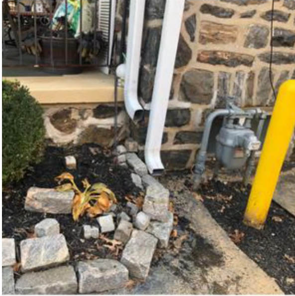
Sinking and new location ( not courtesy)
