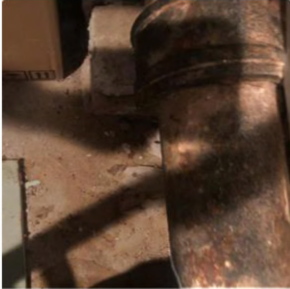
Pipe next to heater
