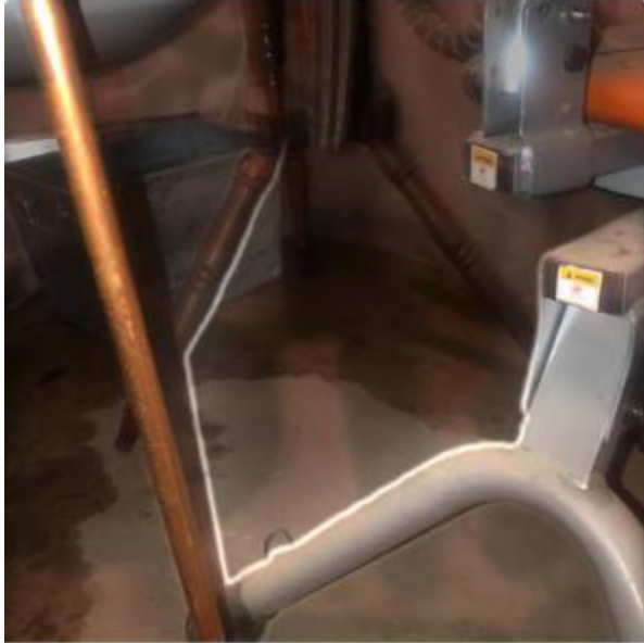
flooding at base of chimney in utility room ( the gray pan is my fireplace shoot catcher. Copper pipe is part of my heater * note corrision ... more
