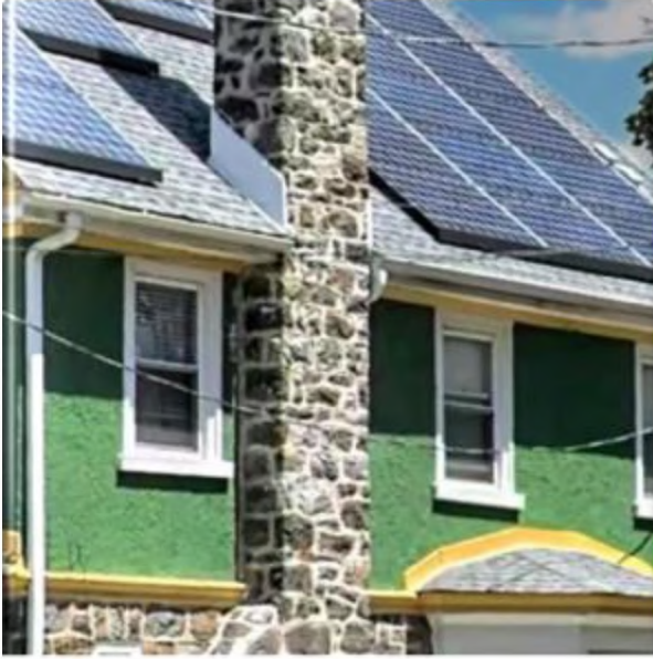
hole in chimney
