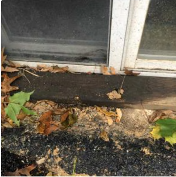
Window/ Foundation patch
