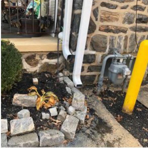
Sinking and new location ( not courtesy)
