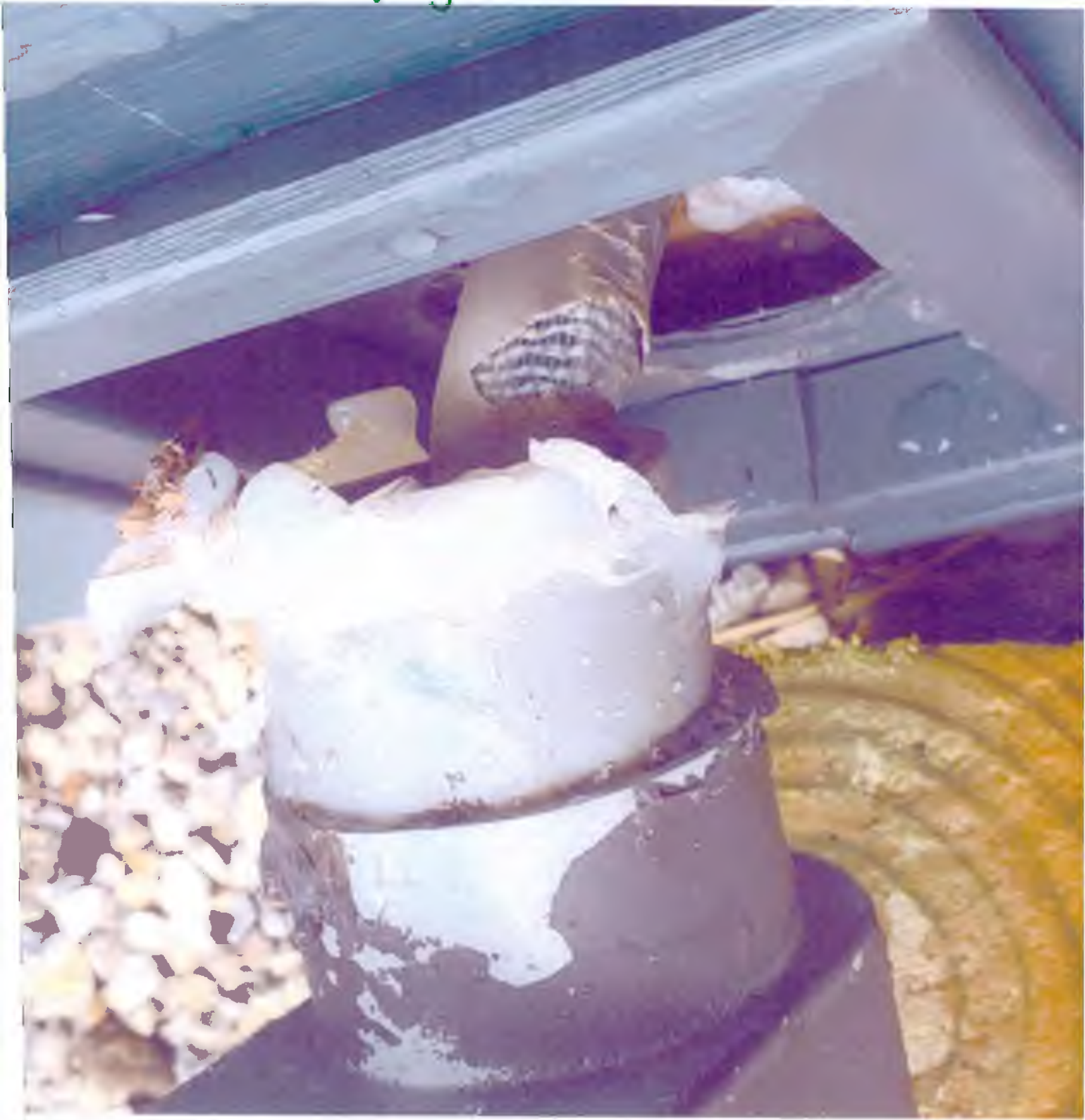
Electrical wire exposure - leads to home's basement. 12/30/24
