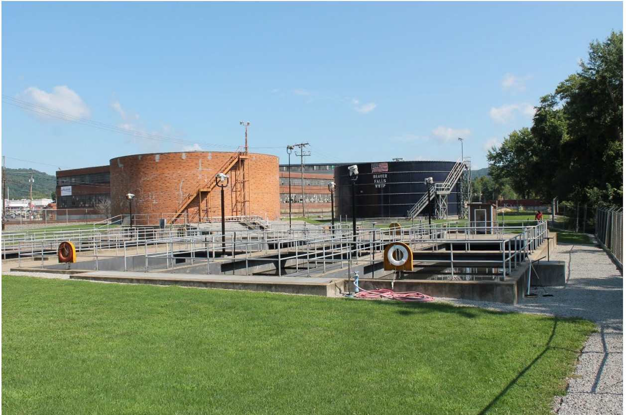
FIGURE 5.3 - 10: SECONDARY SETTLING TANKS AND OXIDATION TOWERS
