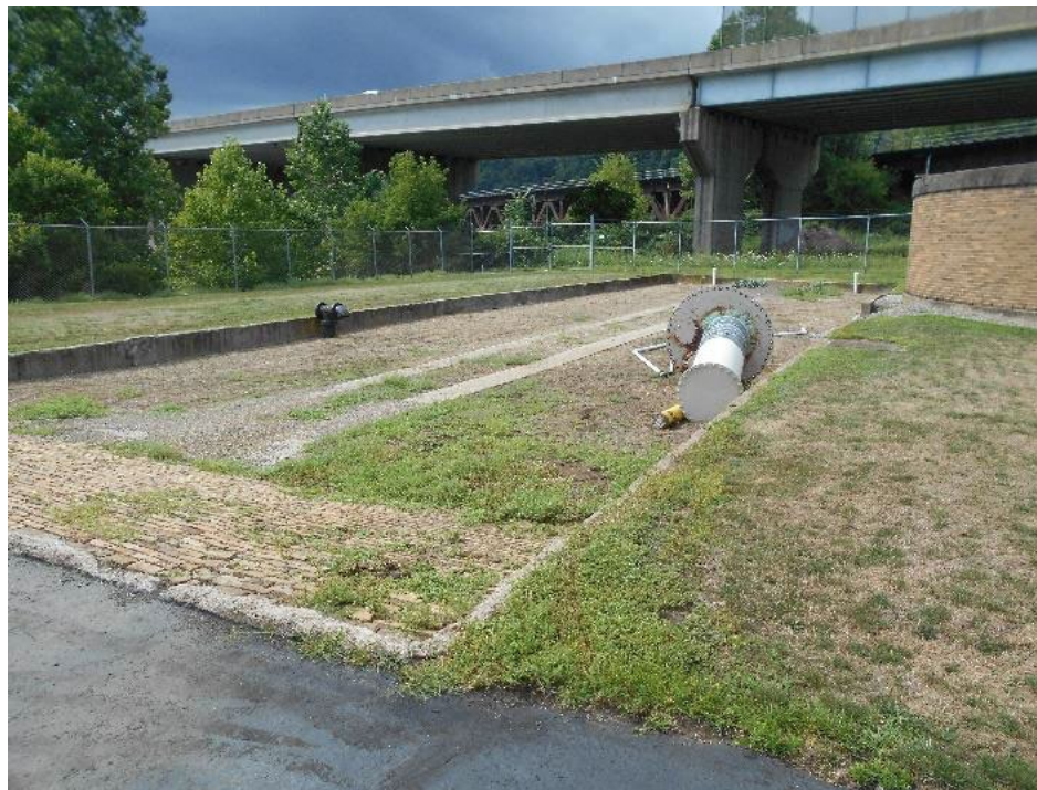
FIGURE 5.3 - 26: REMAINING SLUDGE DRYING BED
