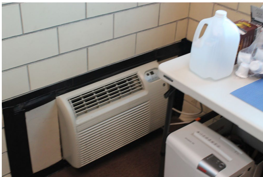
FIGURE 5.3 - 44: COMBO HEAT-AC UNIT
