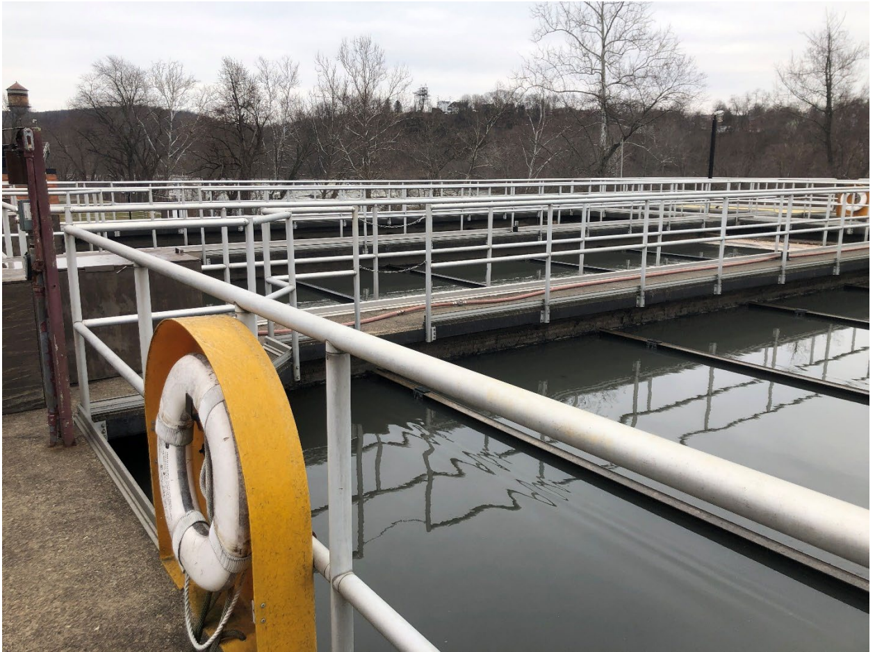
FIGURE 5.3 - 7: PRIMARY SETTLING TANKS-TOP VIEW
