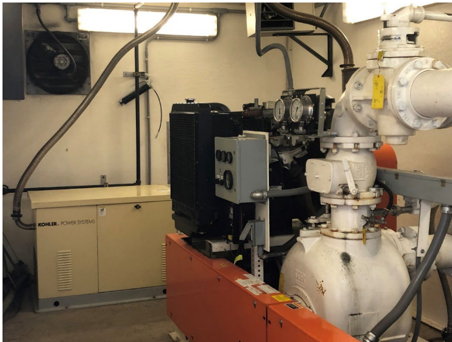
FIGURE 5.2-3: EASTVALE PUMP STATION SUCTION LIFT PUMPS
