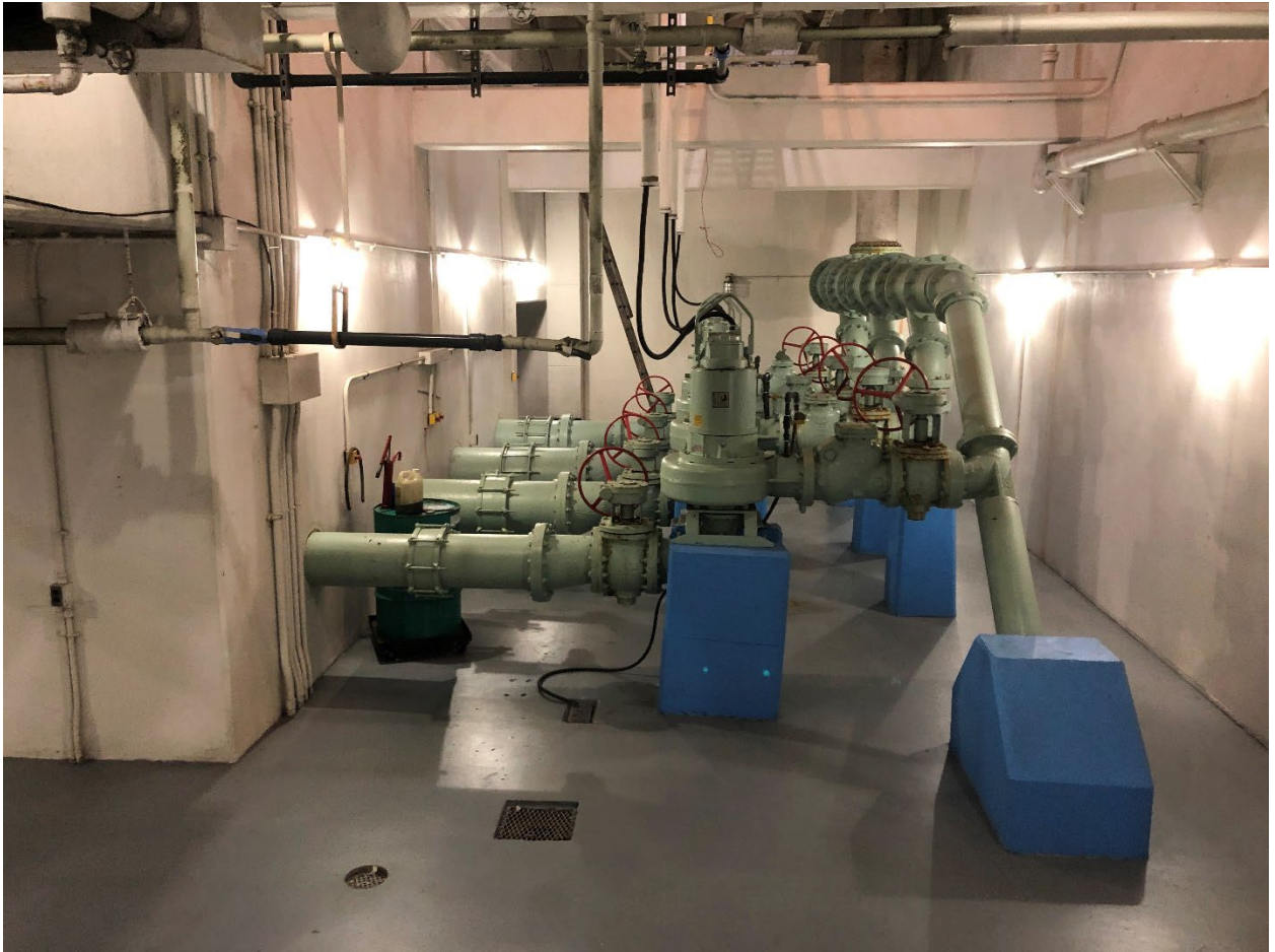
FIGURE 5.3 - 4: RAW SEWAGE PUMPS
