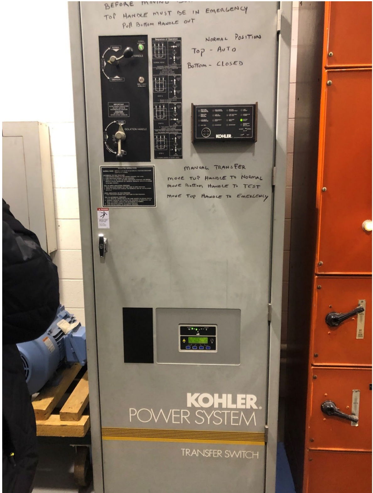
FIGURE 5.3 - 35: AUTOMATIC TRANSFER SWITCH
