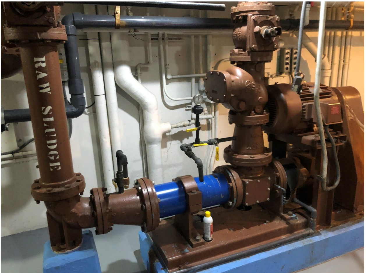
FIGURE 5.3 - 30: SLUDGE TRANSFER PUMPS
