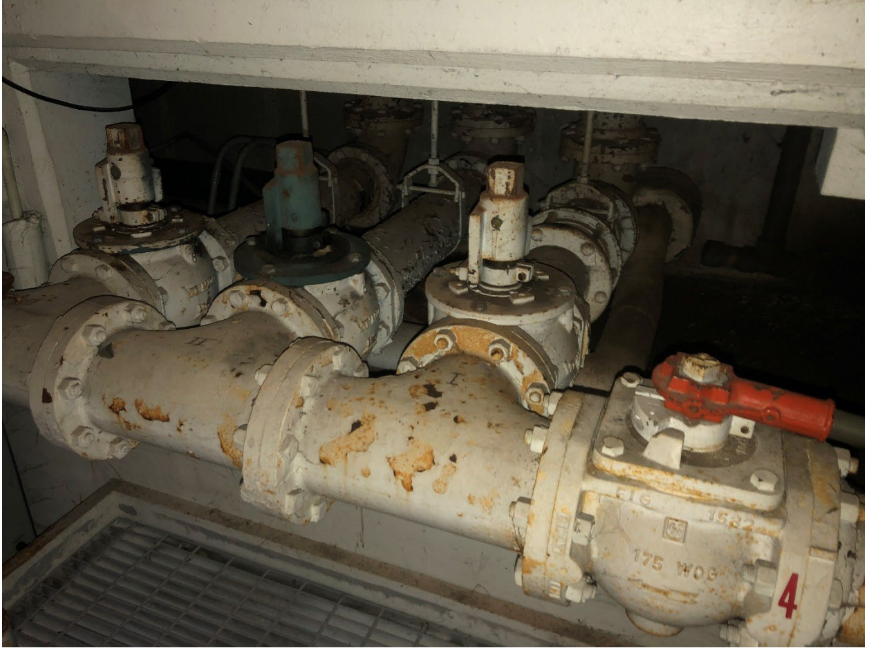
FIGURE 5.3 - 31: PRIMARY TANK FEED PIPING
