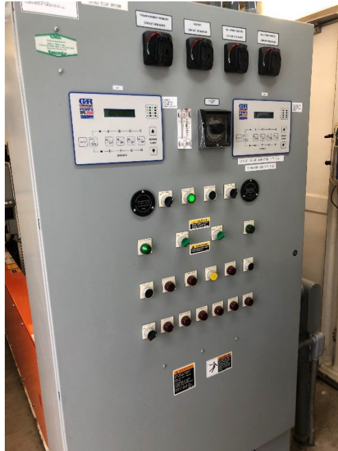
FIGURE 5.2-4: EASTVALE PUMP STATION PUMP CONTROLS
