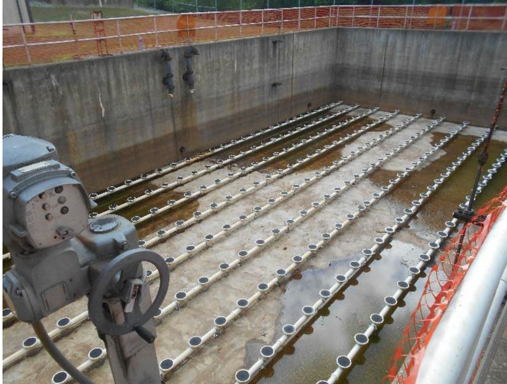
FIGURE 5.3 - 14: SLUDGE THICKENING TANK
