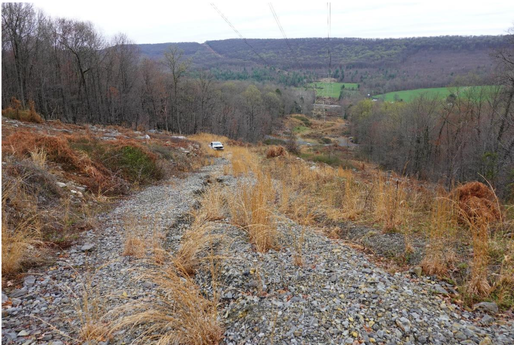
Photo 2: Significant road erosion along the center of the 500kv ROW access route
