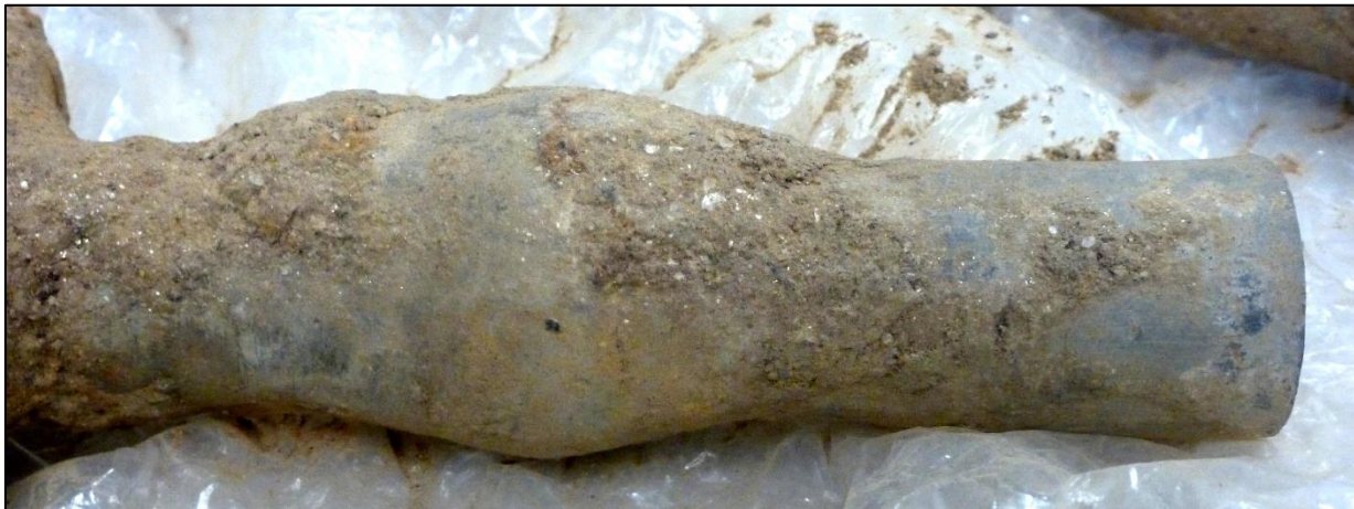
Lead pipe at curbstop. Source: Philadelphia Water
