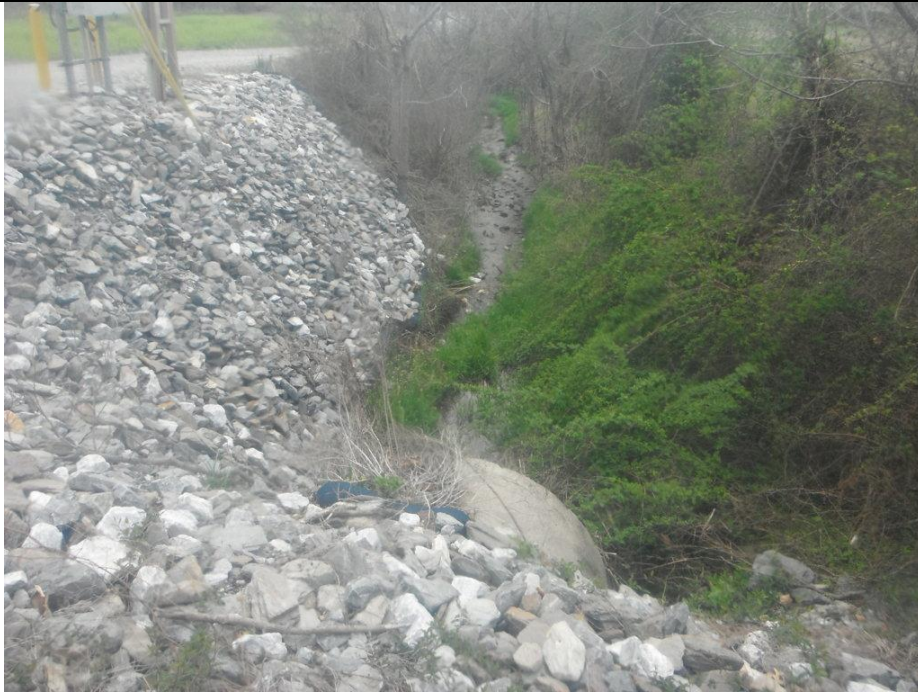
Picture 31 - Looking south/downstream along Stream Channel 3 (UNT to Cabin Creek) from E Prospect Road (4/14/2025)
