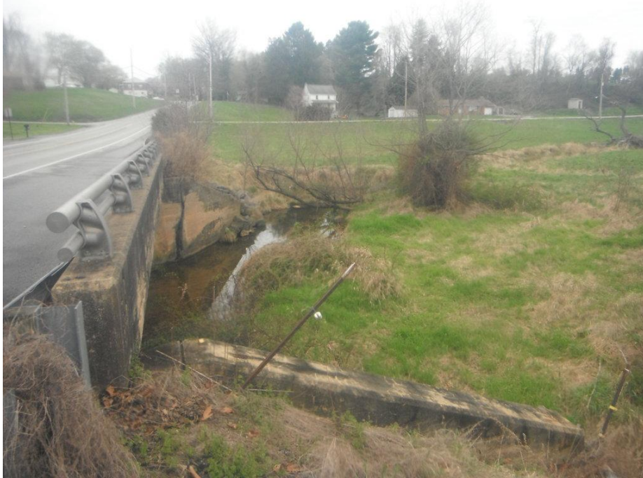
Picture 21 - Looking west across Stream Channel 2 (UNT to Cabin Creek)to the north of E Prospect Road (4/14/2025)
