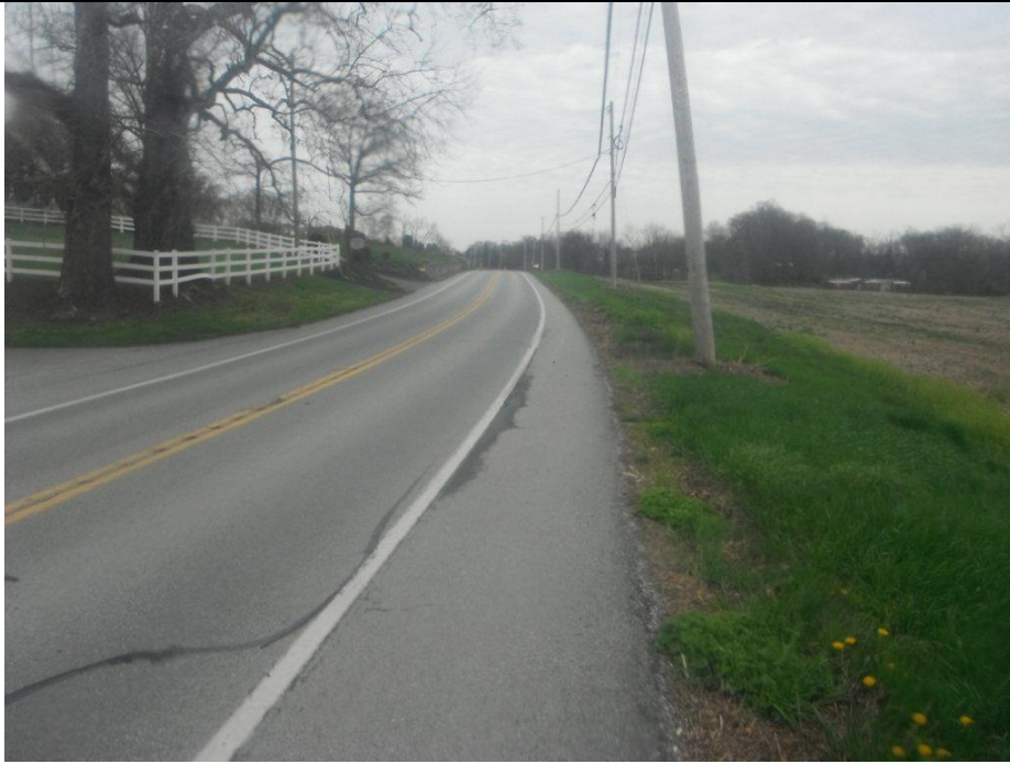
Picture 27 - Looking east along E Prospect Road near the Stream Channel 2 (UNT to Cabin Creek) crossing (4/14/2025)
