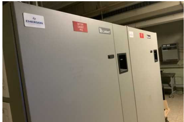
30 UNINTERRUPTIBLE POWER SUPPLY, UPS
