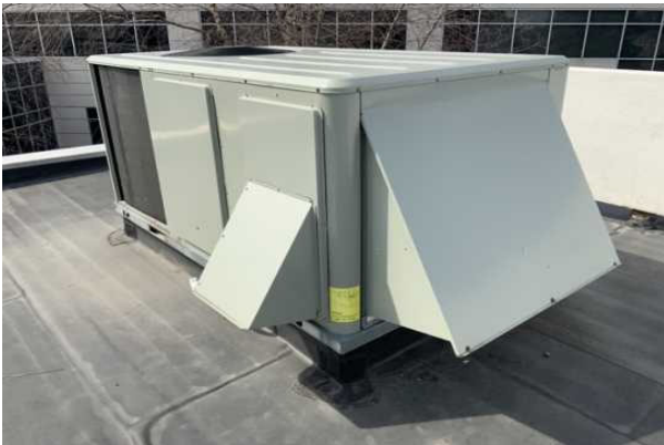
15 PACKAGED UNIT, RTU
