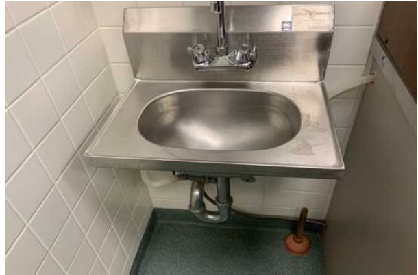
20 COMMERCIAL KITCHEN SINK
