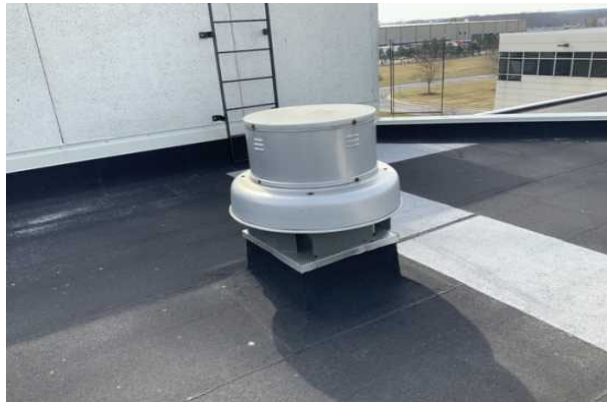
16 EXHAUST FAN, ROOF
