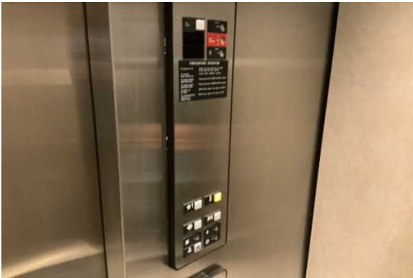
27 PASSENGER ELEVATOR, HYDRAULIC
