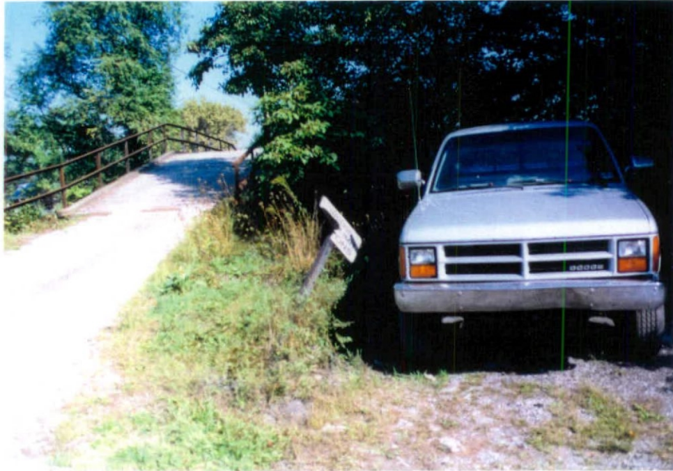
DAMAGED BRIDGE POSTING SIGN AT SOUTH APPROACH
