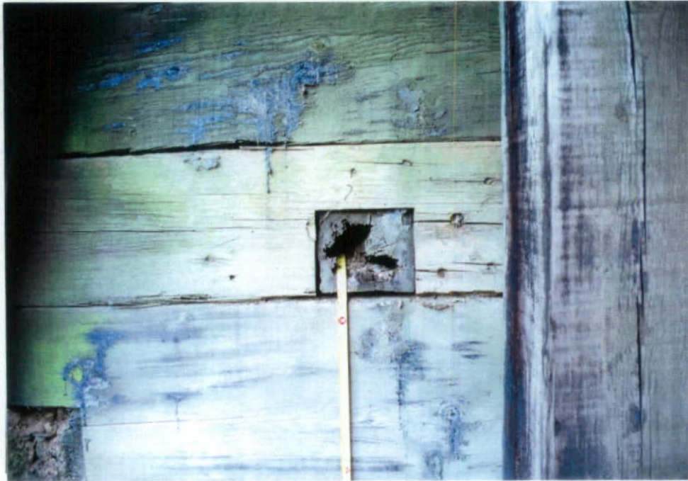
TYPICAL ROTTED TIE-BACK TIMBER AT NORTH ABUTMENT
