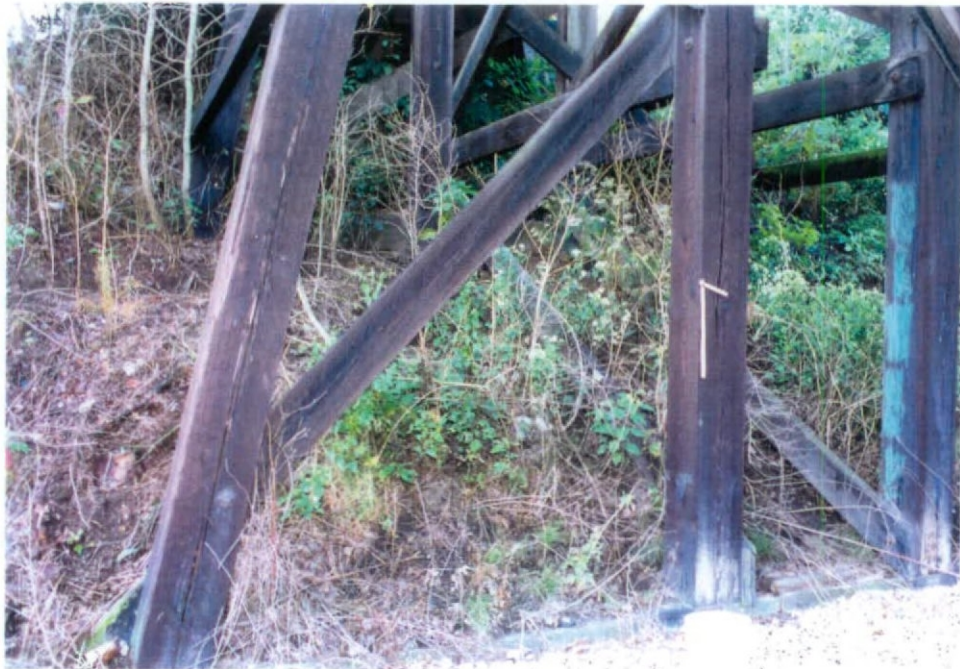
SPLITS AND CHECKS IN COLUMNS OF BENT NO. 2
