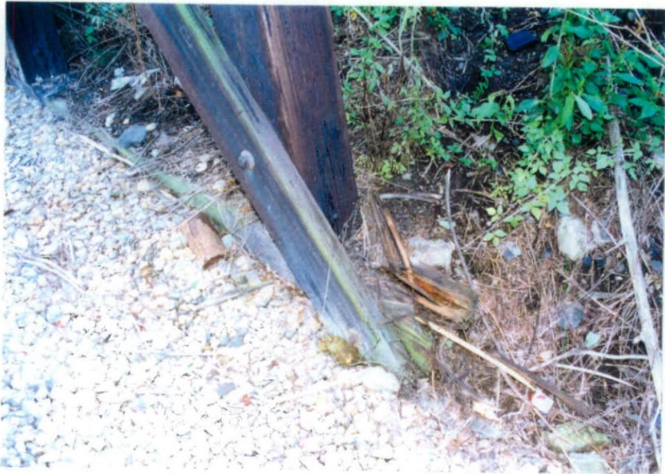
DECAYED AND SPLIT SILL OF BENT NO. 2
