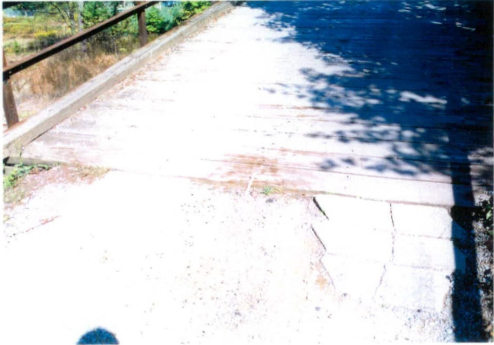
SETTLEMENT OF SOUTH APPROACH ROADWAY
