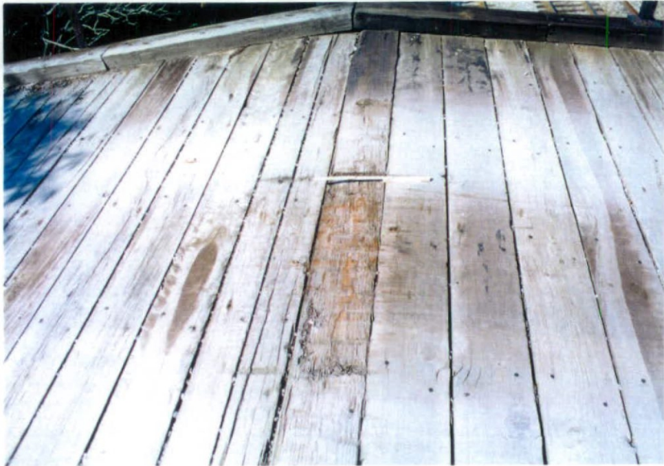
VEHICULAR SCRAPE HACKS IN TIMBER DECKING ABOVE BENT NO. 2
