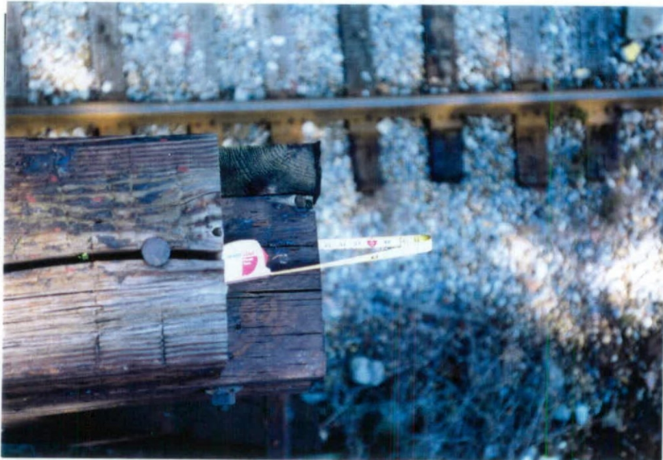
DECAY AND ROT IN BENT NO. 2 CAP BEAM
