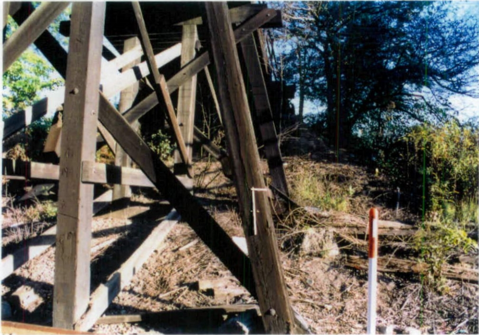
SPLITS AND CHECKS IN COLUMNS OF BENT NO. 3
