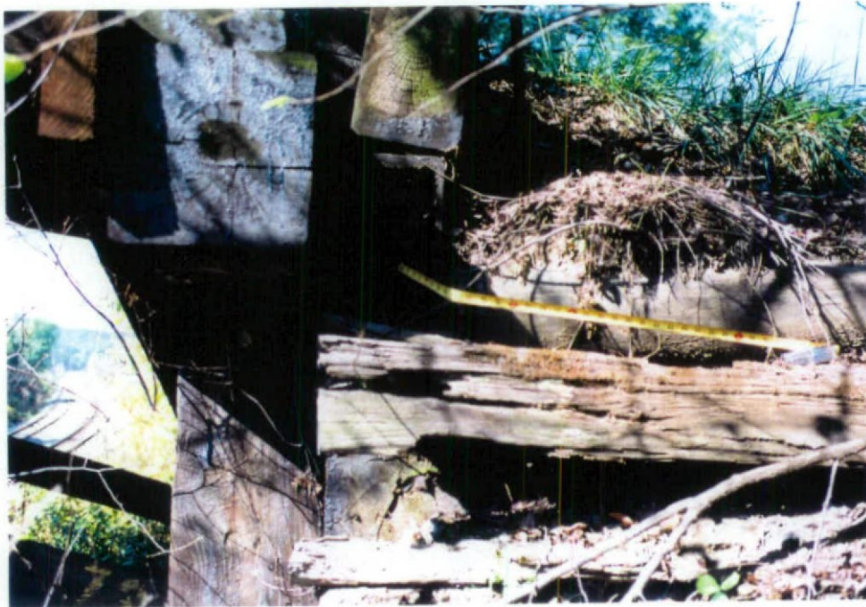
ROTTED RETAINING WALL TIMBERS AT NORTH ABUTMENT - EAST SIDE
