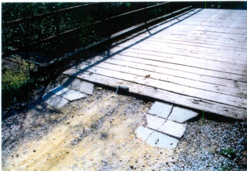
SETTLEMENT OF NORTH APPROACH ROADWAY
