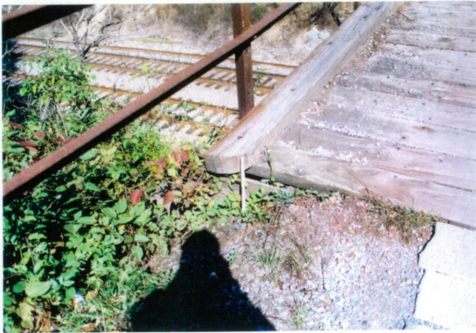
EROSION OF SOUTHWEST ROADWAY EMBANKMENT
