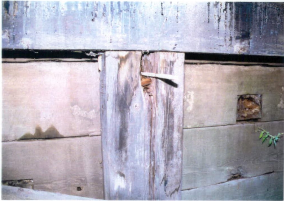
SPLITS, CHECKS, AND HOLE ROTTED IN COLUMN OF SOUTH ABUTMENT
