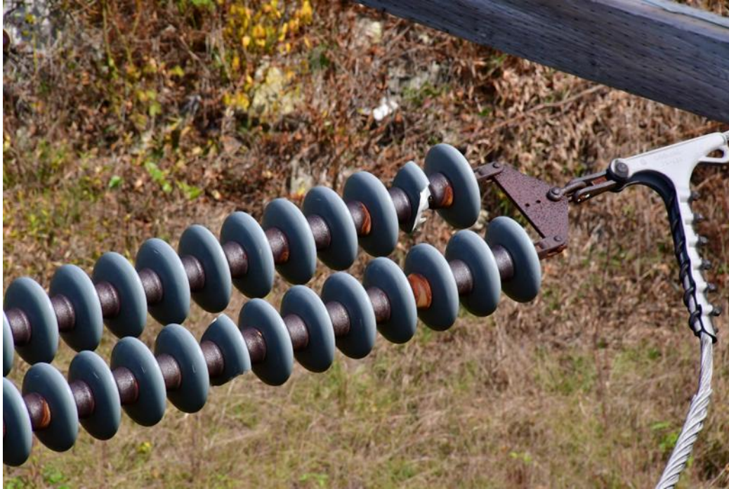
Figure 3: Broken insulator bells original to the construction of the line. Located at structure 43
