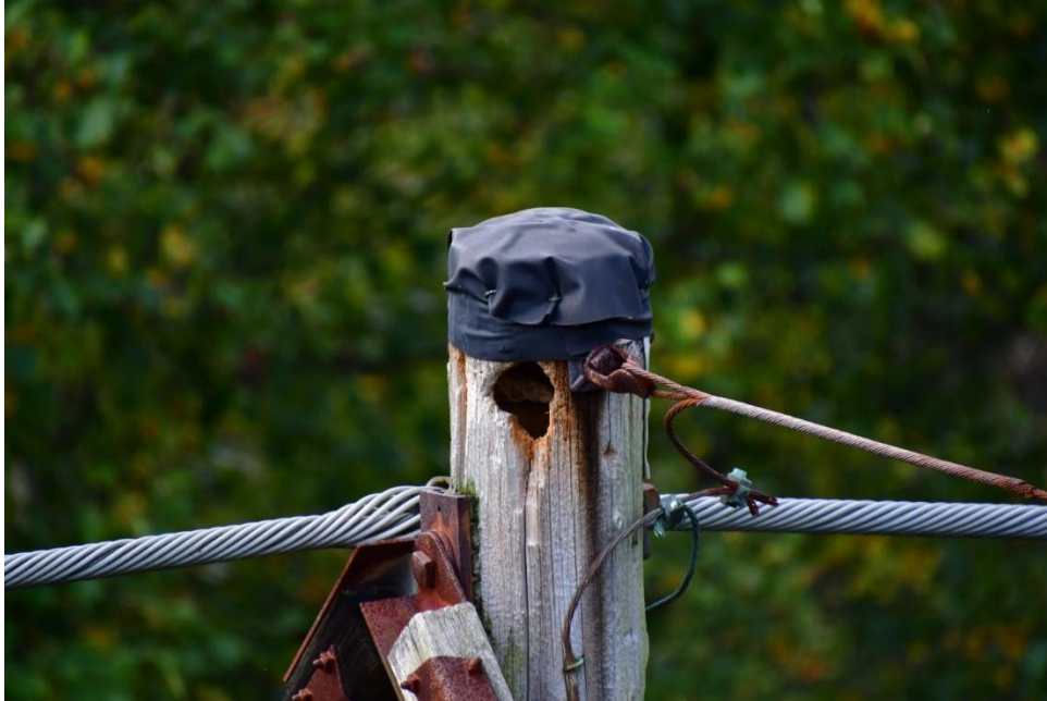
Figure 1: Active woodpecker hole on structure 7. This pole was also repaired in 2016 with a pole top cap due to extensive pole top rot.
