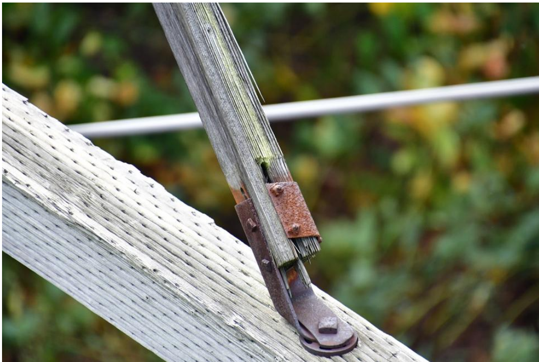
Figure 2: A cross-arm brace or “knees and vees” has degraded, allowing the metal bracket supporting the cross arm to slide down the wood. Located at structure 15.
