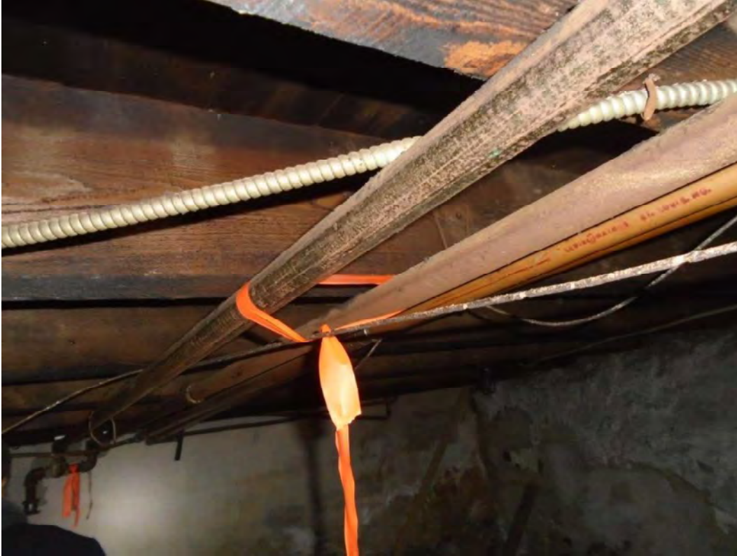
Photograph #21: Natural gas pipes in basement.
