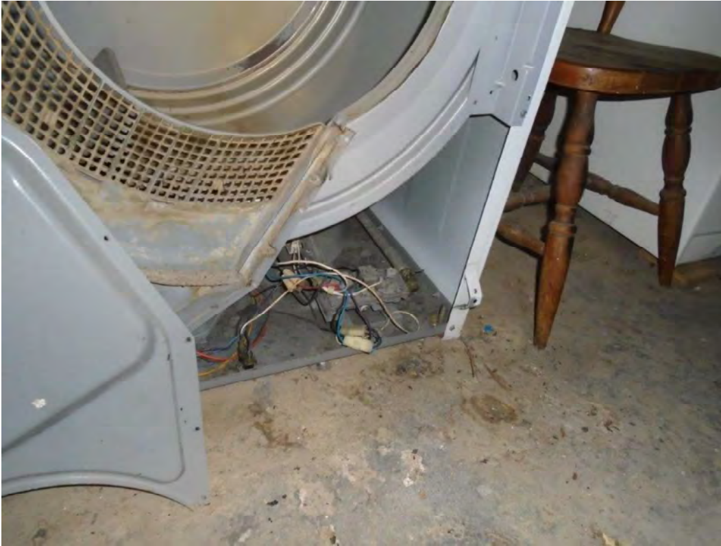
Photograph #33: Flame chamber for gas dryer.
