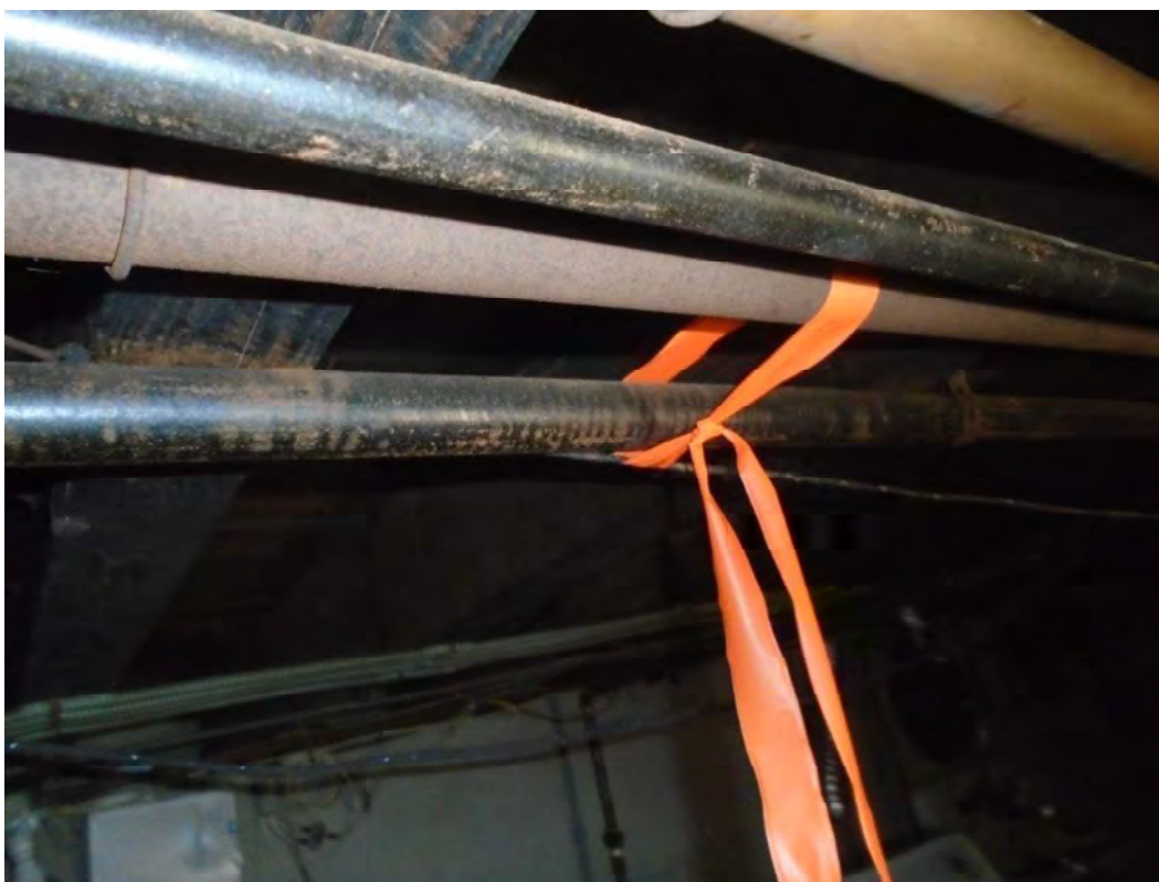
Photograph #14: Natural gas pipes located in basement at 815 Jackson Street.
