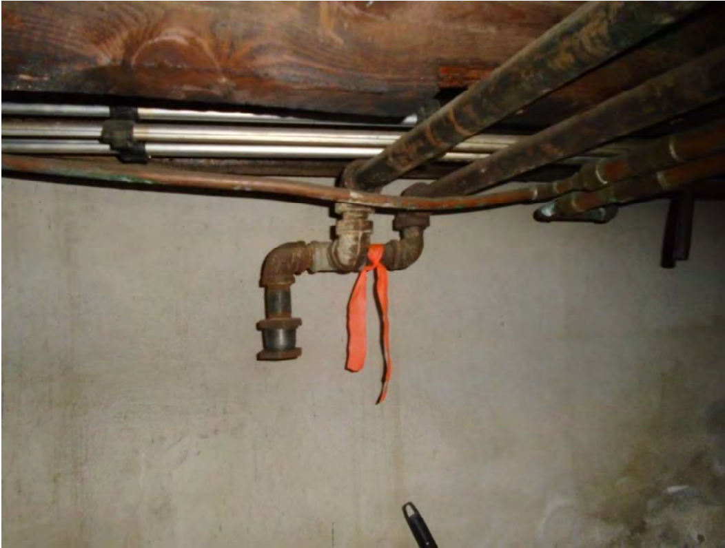
Photograph #17: Gas pipes where gas meter was located.
