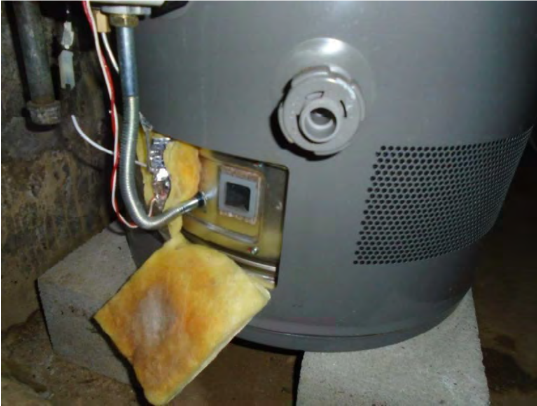
Photograph #31: Flame chamber for hot water.
