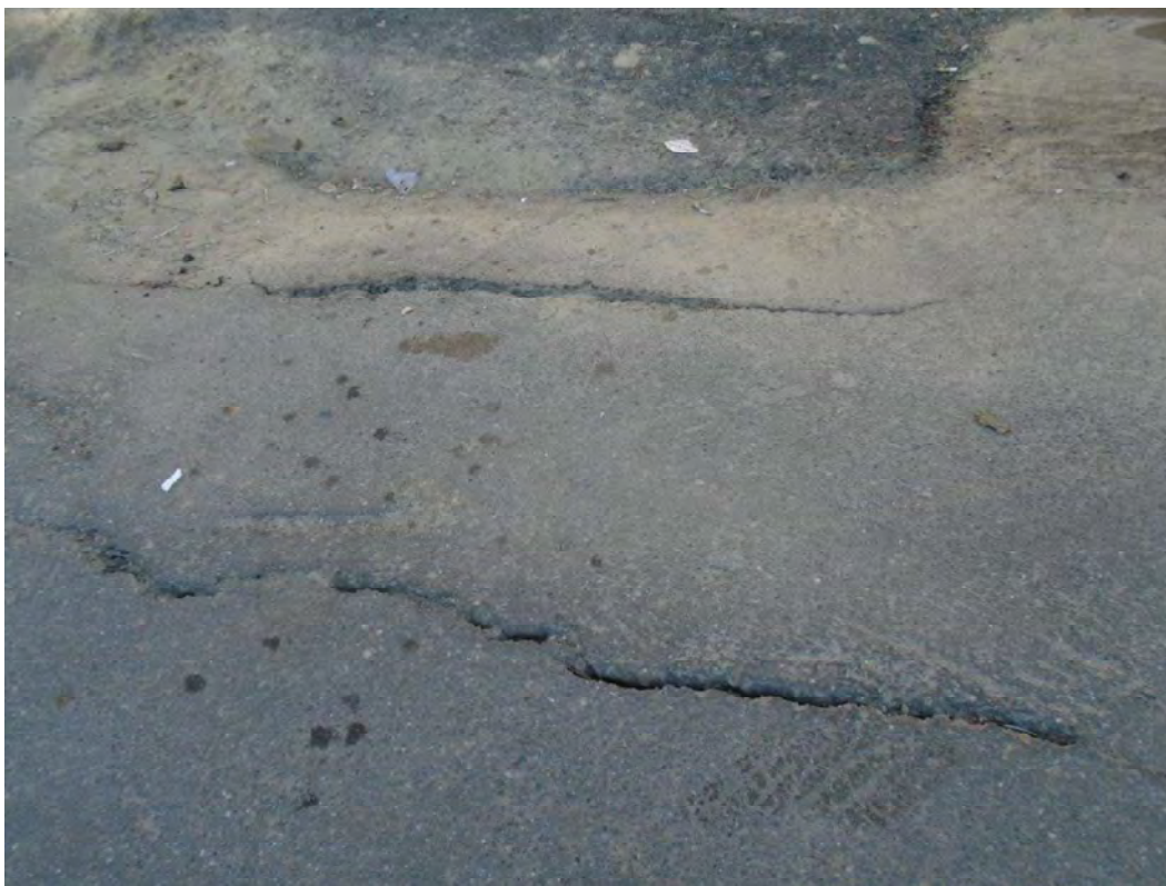
Photograph #44: Ground undermined in the front of 815 Jackson Street.
