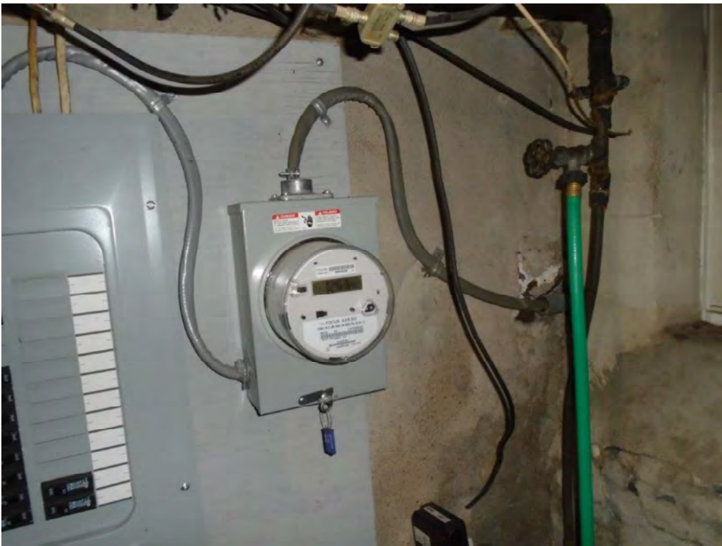
Photograph #18: Electric meter in basement.
