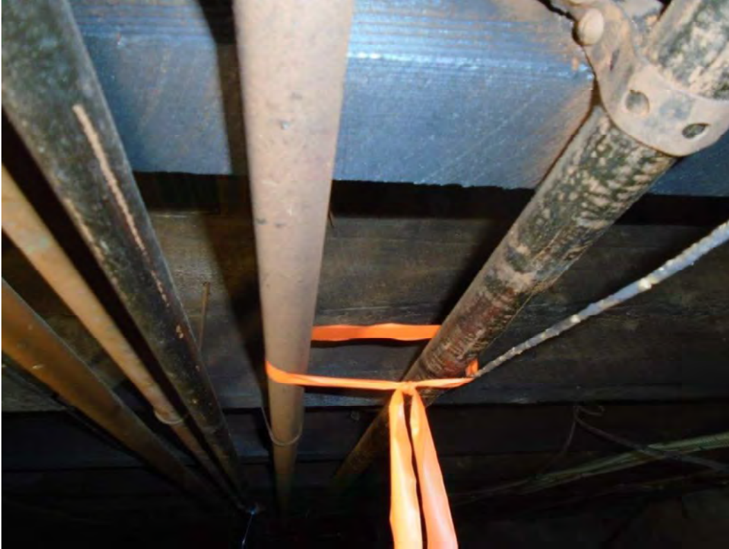
Photograph #23: Natural gas pipes in basement.
