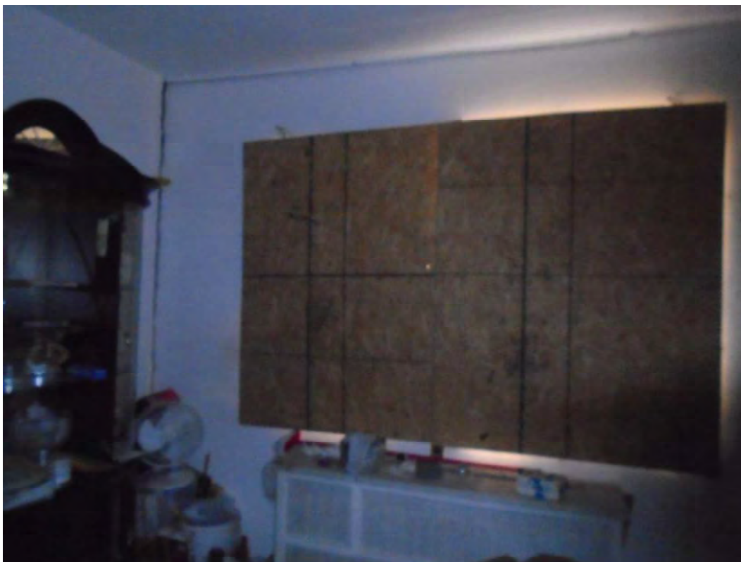
Photograph #12: Front window broken out in living room.
