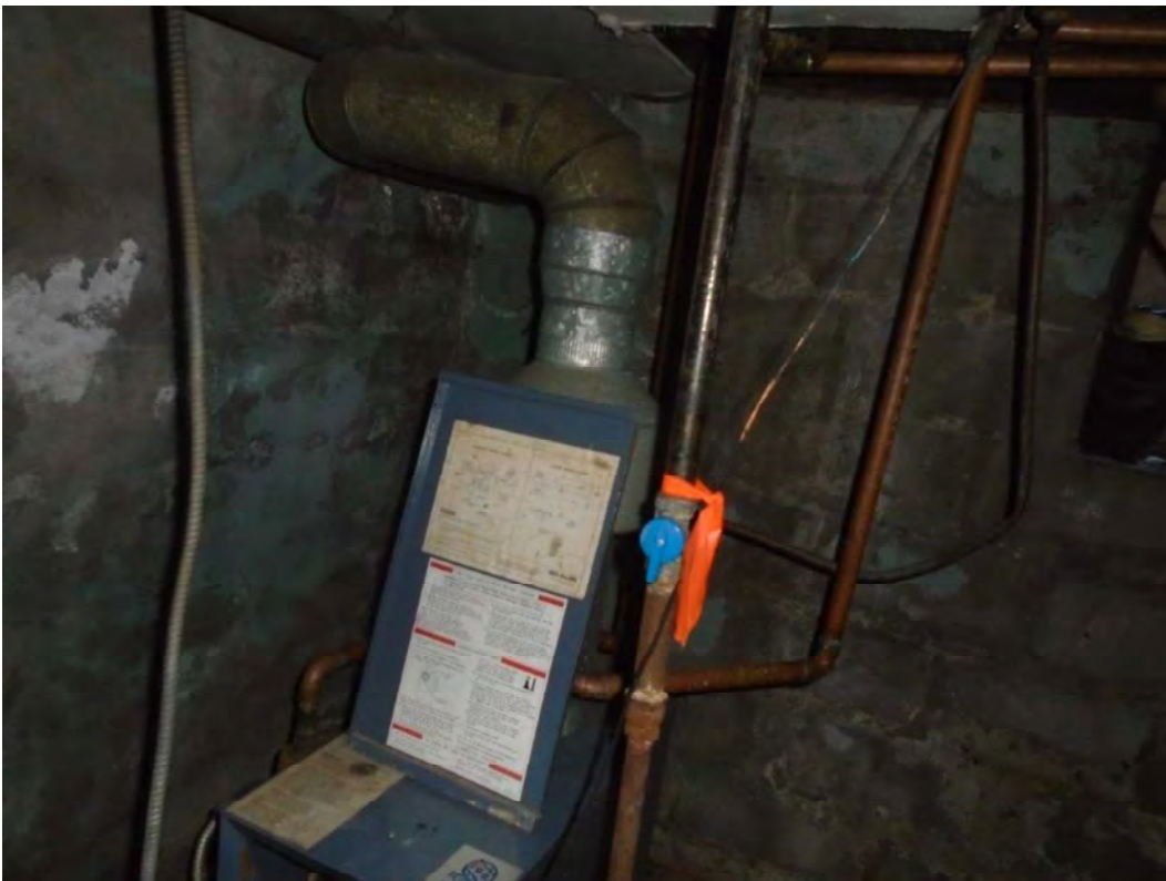
Photograph #28: Flue pipes for heater.
