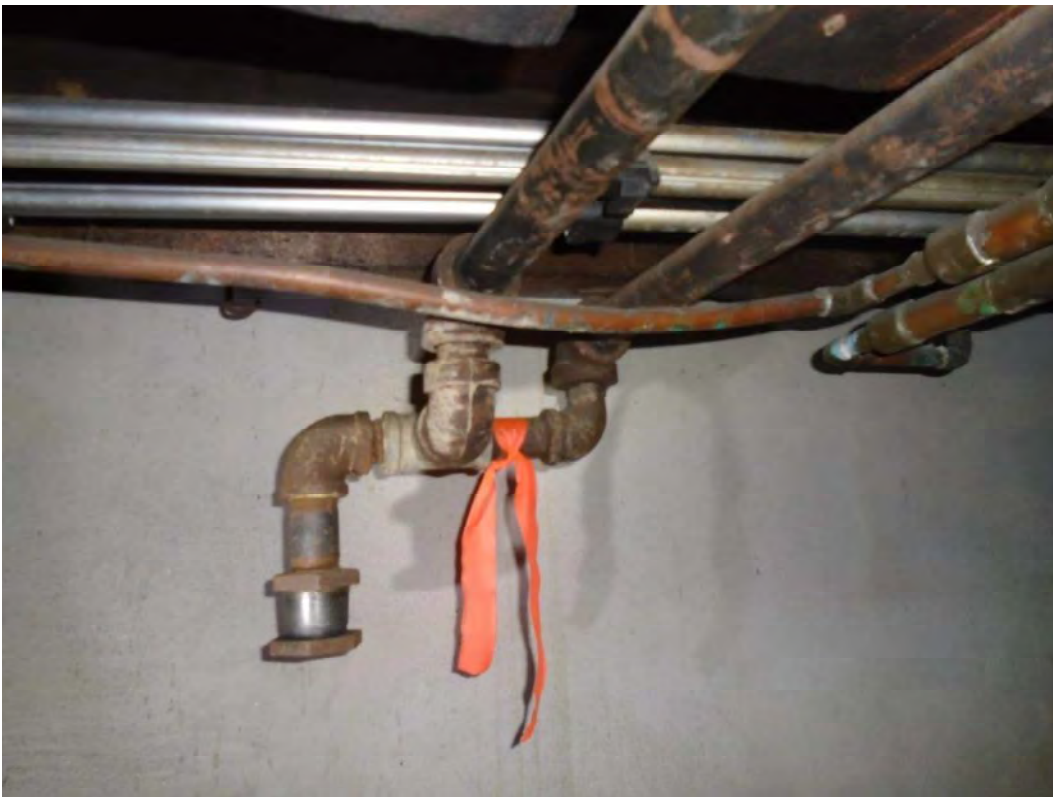
Photograph #22: Natural gas pipes in basement.
