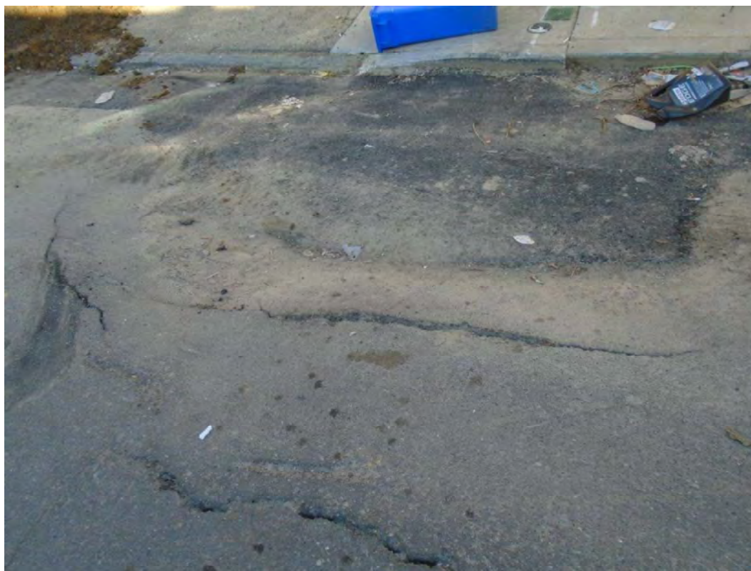
Photograph #45: Ground undermined in the front of 815 Jackson Street.
