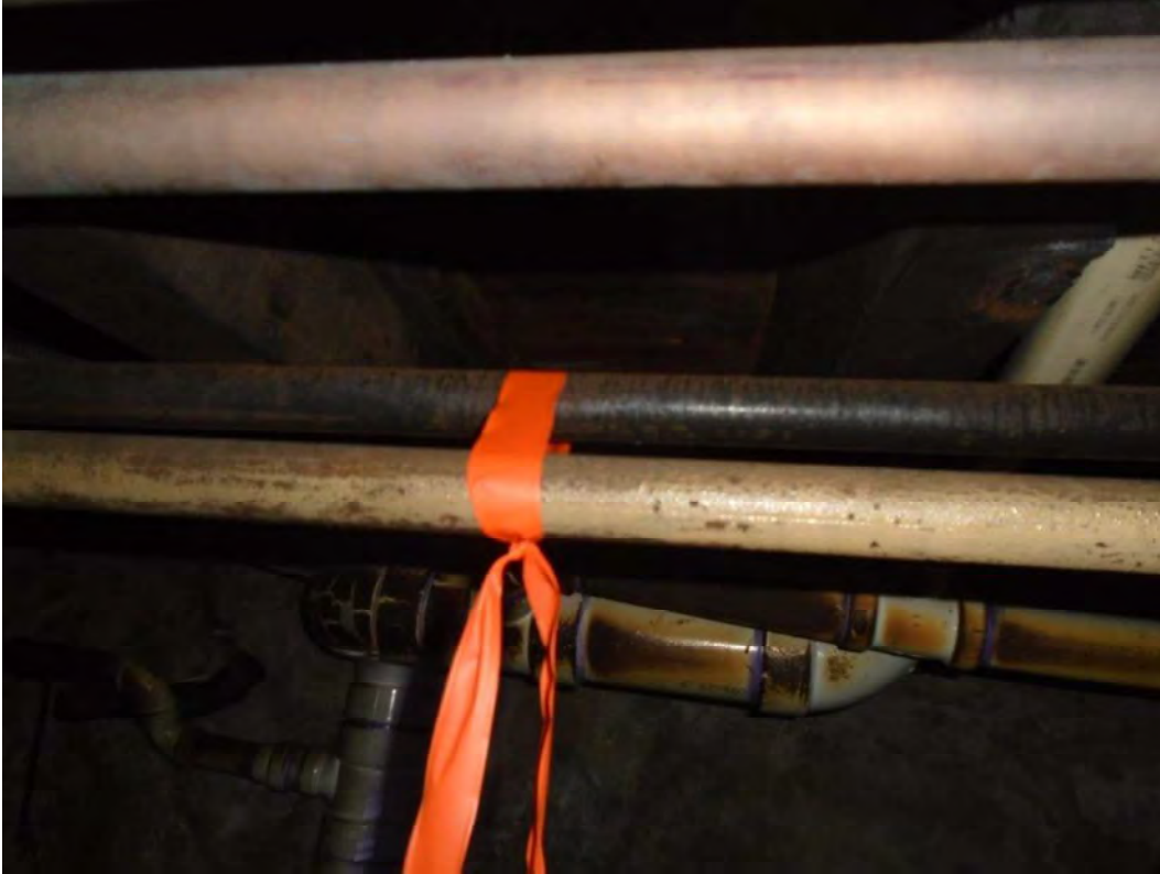
Photograph #25: Gas pipes in basement/heat stains on drainpipes.
