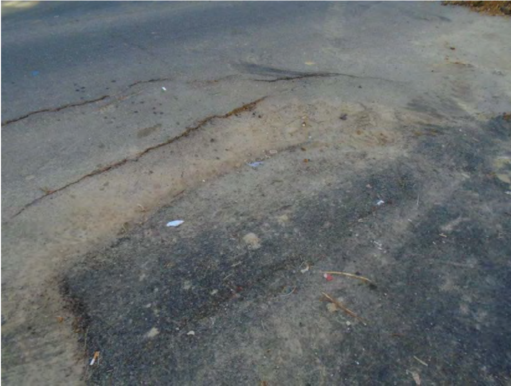
Photograph #41: Ground undermined in the front of 815 Jackson Street.
