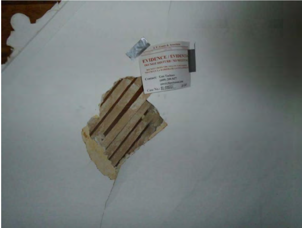
Photograph #11: Damaged living room wall at stairwell.
