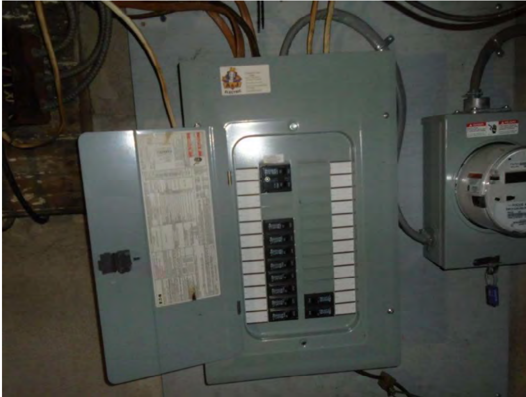
Photograph #19: Circuit breaker panel in basement.
