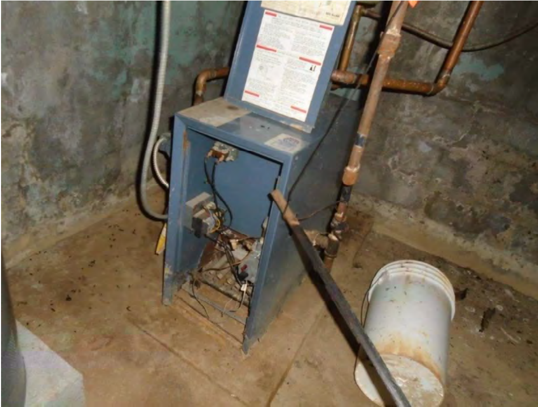
Photograph #27: Natural gas-fired heater in basement.
