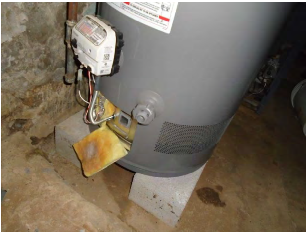
Photograph #30: Flame chamber for hot water.
