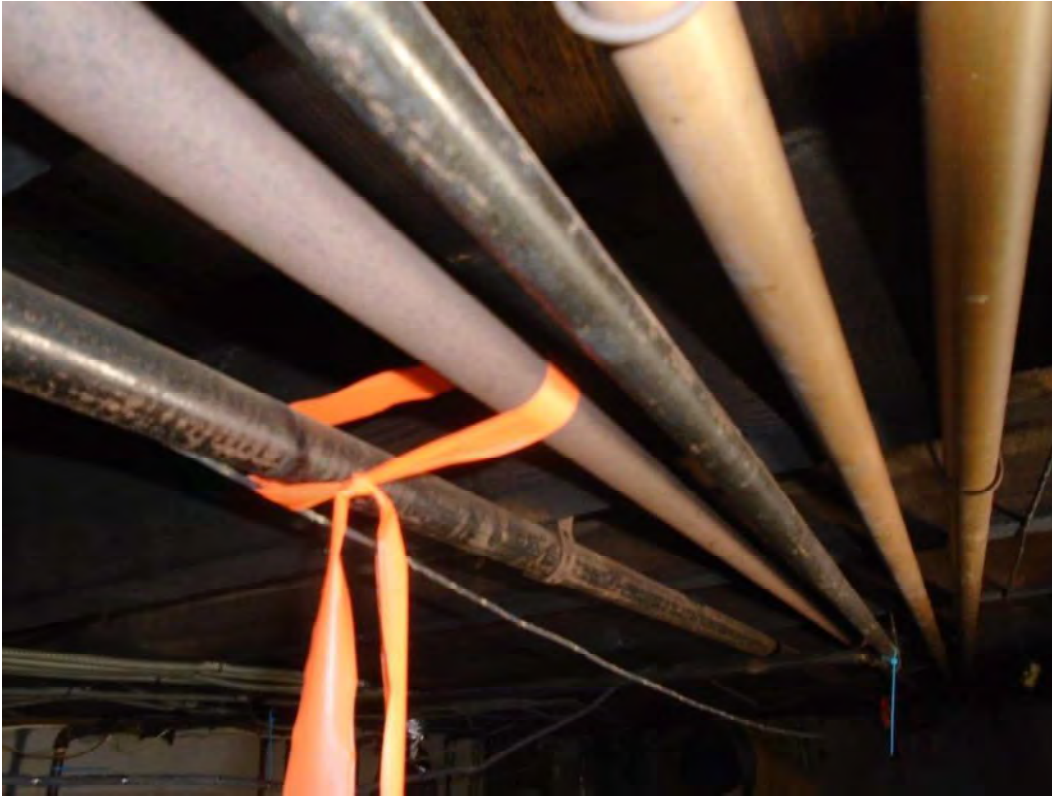
Photograph #35: Gas pipes in basement.
