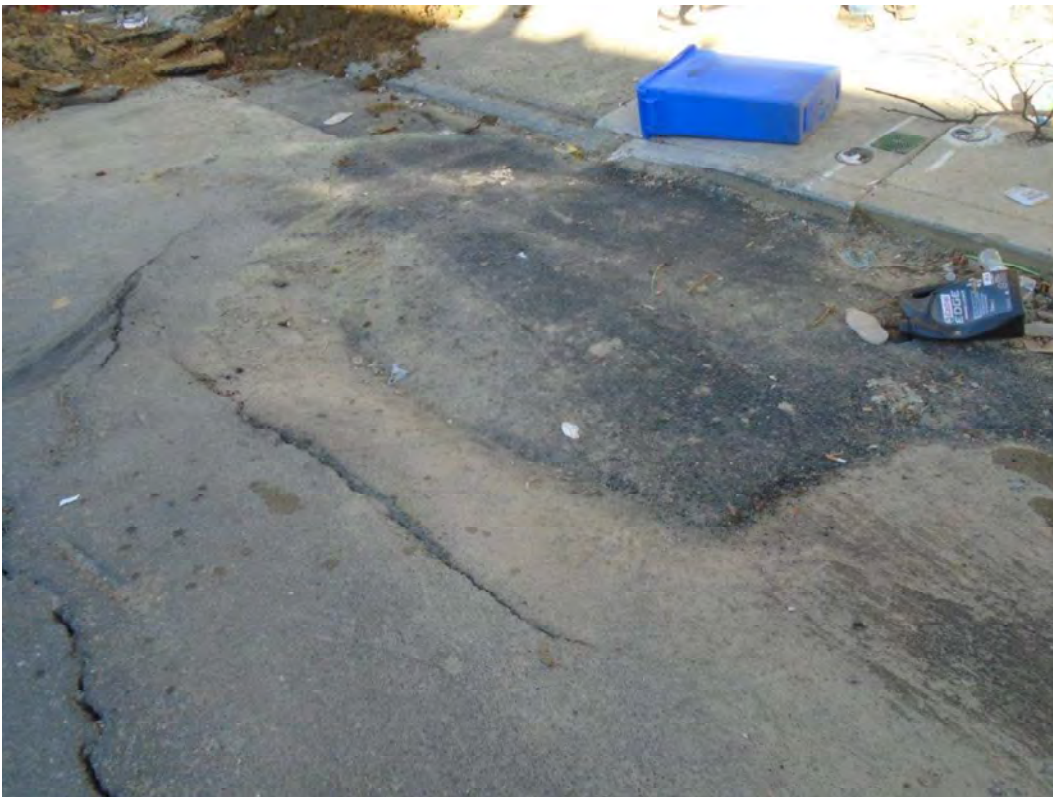
Photograph #42: Ground undermined in the front of 815 Jackson Street.
