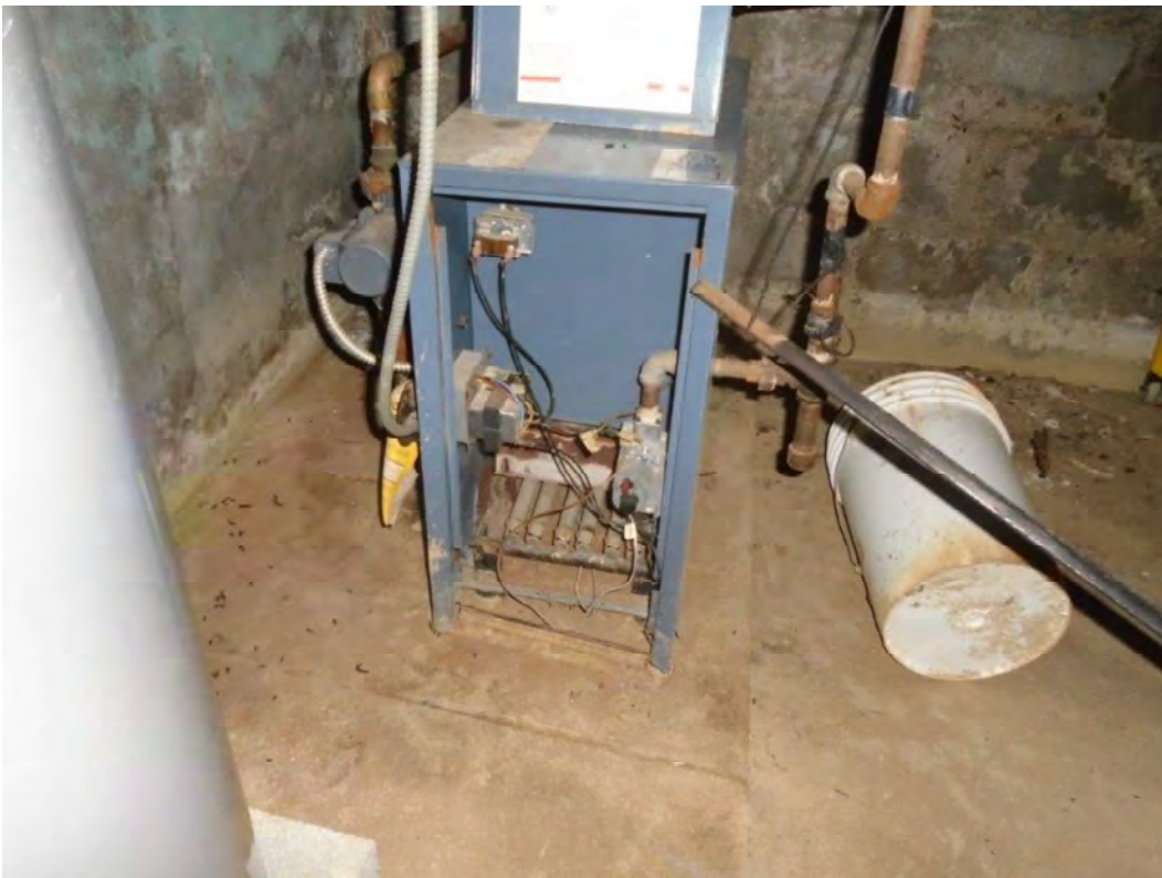
Photograph #32: Flame chamber for heater.
