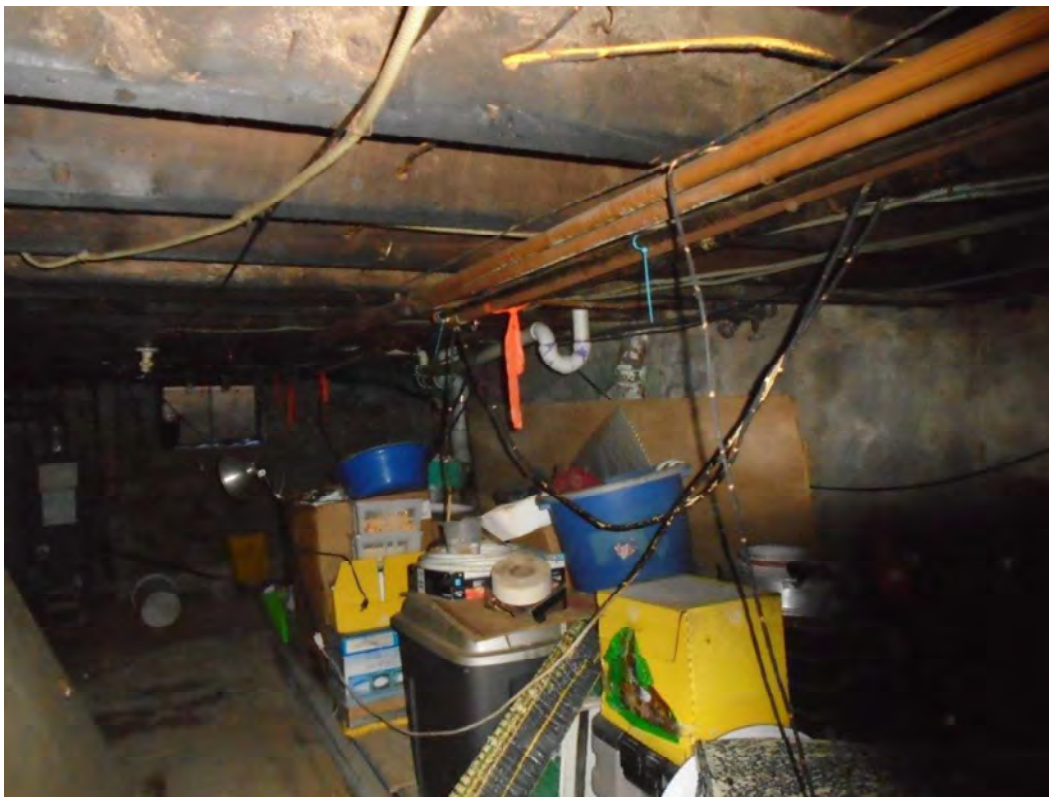
Photograph #13: Natural gas pipes located in basement at 815 Jackson Street.
