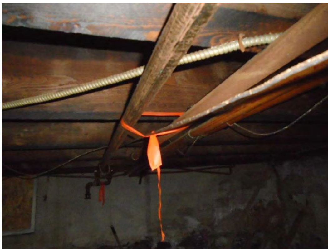
Photograph #16: Natural gas pipes in basement.
