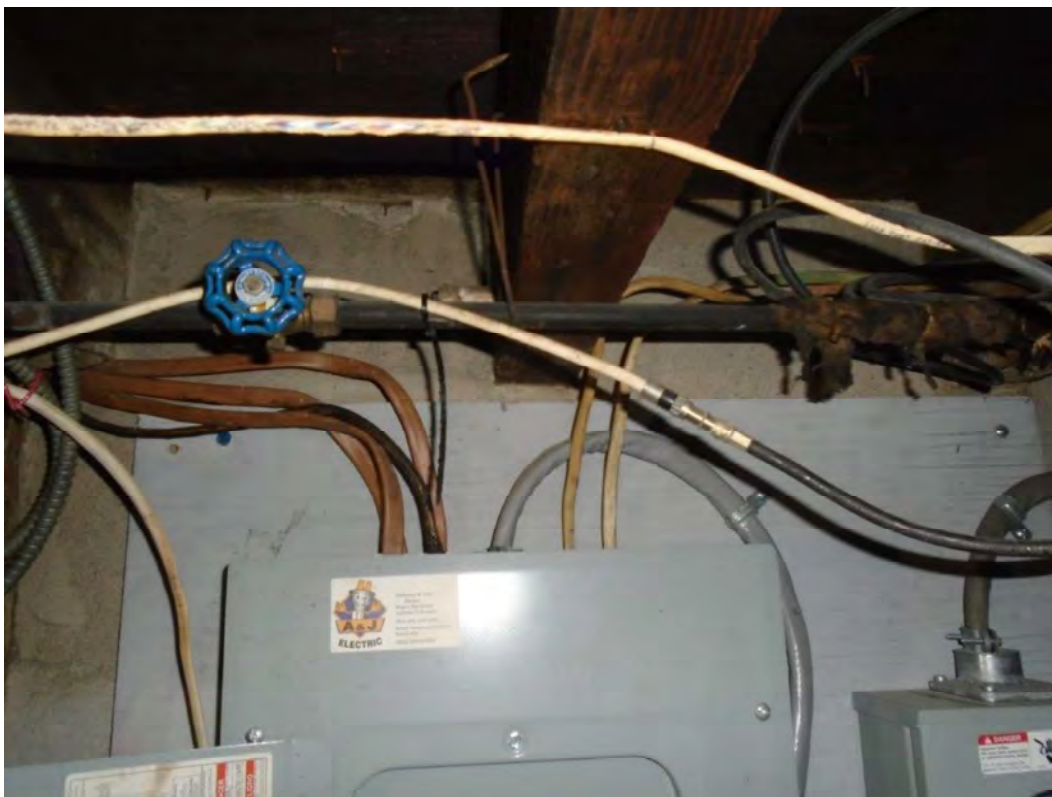
Photograph #20: Associated wiring from circuit breaker panel.
