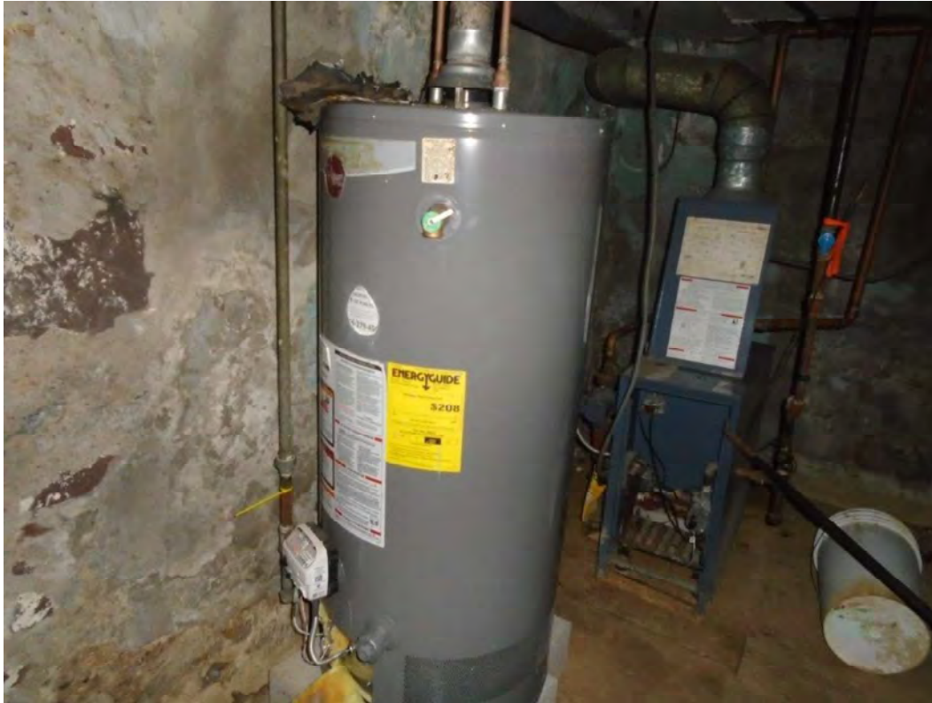
Photograph #29: Natural gas-fired hot water heater located in basement.
