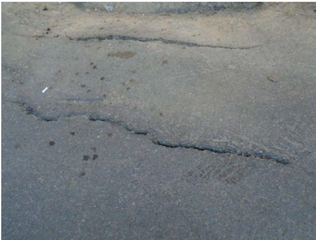
Photograph #43: Ground undermined in the front of 815 Jackson Street.
