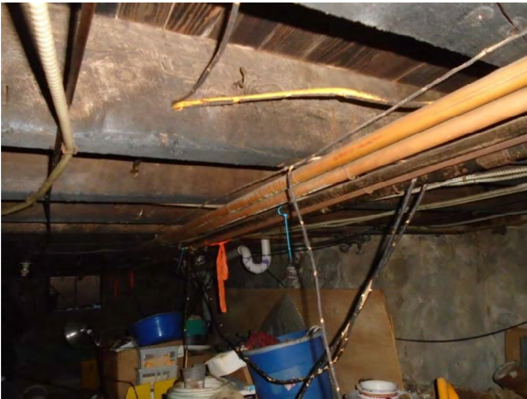
Photograph #36: Gas pipes in basement.
