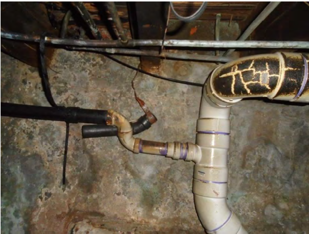
Photograph #26: Heat stains on drainpipes in basement.
